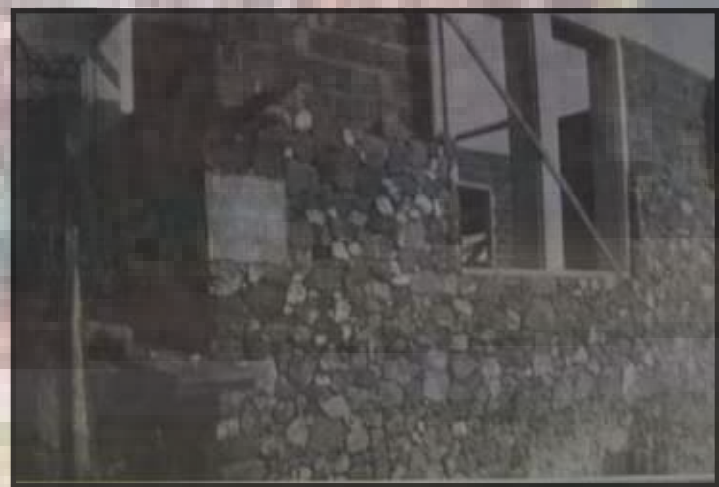
In this view the core of the walls is nearly complete and the windows and door are framed. The application of stone to the exterior continued, section by section. The hand-lettered cornerstone placed by J.C. Bankston Jr. reads "Built by J.C. Bankston and son 1938. (U.S. Air Force courtesy photo)
