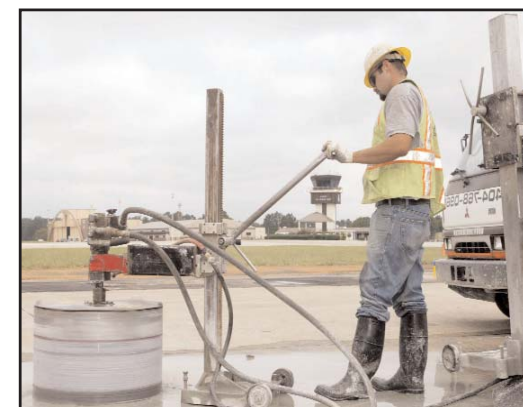
A construction crew member drills into the runway to remove a segment of concrete required to replace aging runway lighting. The runway was closed Aug. 18 through Sept. 19 during the renovation. (Air Force photo/Don Peek)
