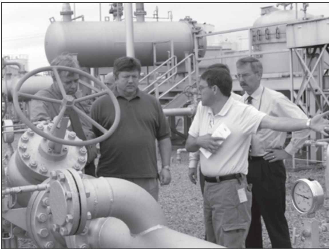
From left to right, DESC representatives Bill Gibson, Jim Mandziara and Tom Ashman receive a tour of the Plantation Pipeline Company's facilities a mile from Fort Belvoir, Va. Murray Clayton gestures as he explains pipeline operations. The visit was part of the Automatic Identification Technology Working group's continuing efforts to identify ways the Department of Defense could employ AIT to improve bulk fuel supply chain operations. (Photo by Susan Declercq Brown)
