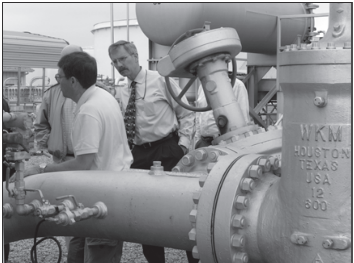
From left to right, Plantation Pipeline Company's Murray Clayton, center, explains site operations to representatives of the AIT Working Group May 6, as a partially hidden Bob Koeller and Tom Ashman lean in for the presentation. (Photo by Susan Declercq Brown)
