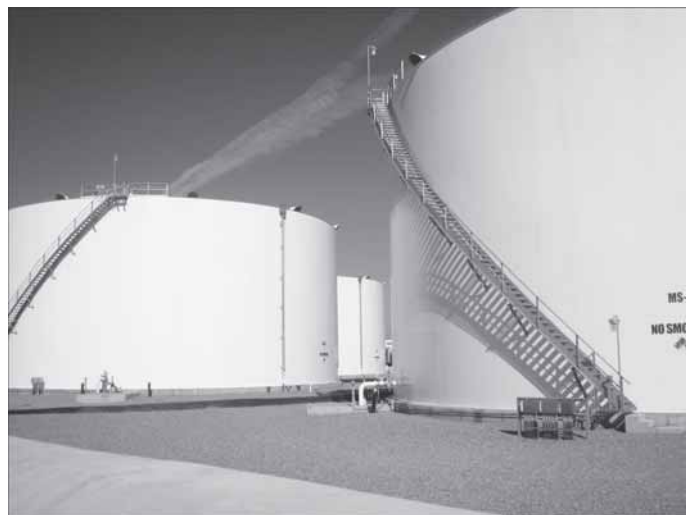
Storage tanks at a new fuel terminal, Marine Corps Air Station Miramar, Calif. (Courtesy photo)
