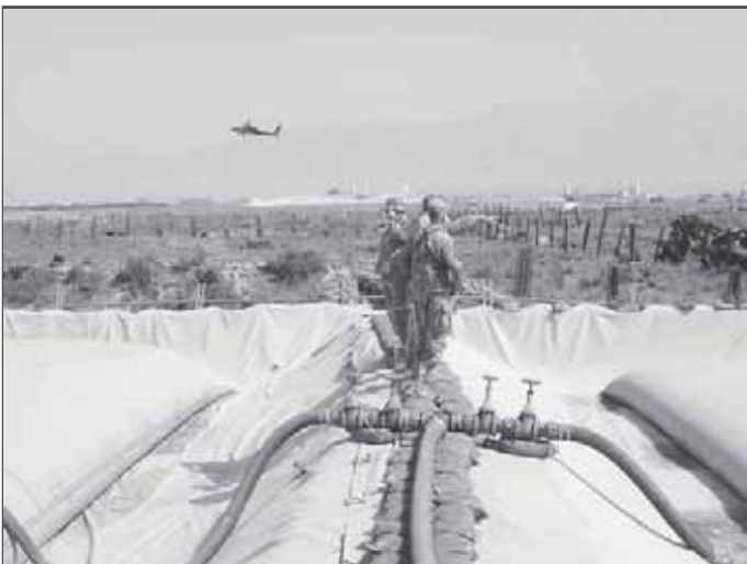
Challenging mountainous terrain is visible from the fuel farm area at Bagram Air Base, Afghanistan.
