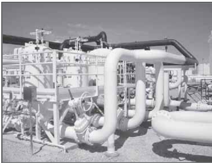
Defense Energy Support Center micronic filters and filter separators at the Las Vegas terminal Kinder Morgan facility outside Nellis Air Force Base, Nev. (Photo by Lt. Col. Jon Ramer)
