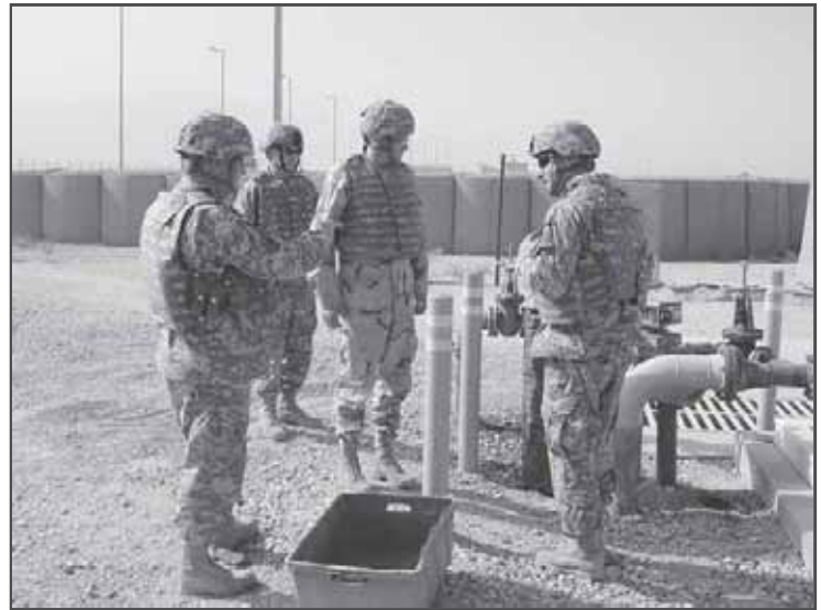
The entourage gathers around a pipeline that delivers fuel from the Red Star Enterprises facility to Bagram Air Base, Afghanistan.
