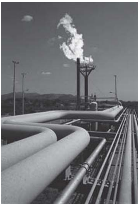
A natural gas pipeline.
