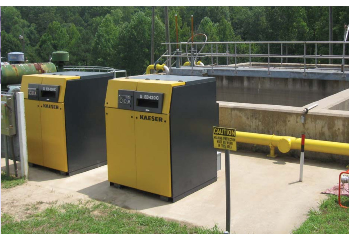
Contractor-owned waste water backup generators at Fort AP Hill, Va., prevent sewage overflow during power outages. Photo provided by Carla Biver, DLA Energy, Energy Enterprise.
