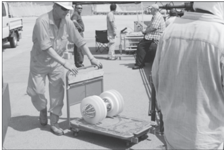
A pipeline scrubber pig is wheeled into position before the August pigging operation begins.
