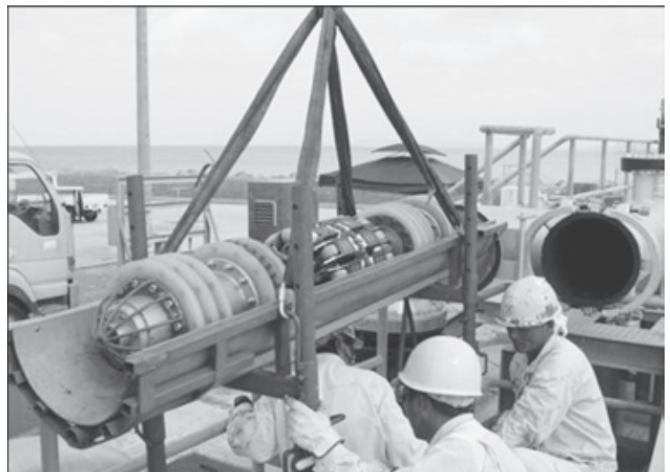
The pipeline inspection pig is recovered at the end of the pigging operation.
