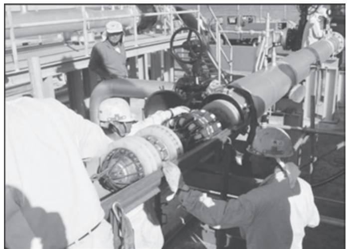
The pipeline inspection pig is launched as the pigging operation begins the final phase.
