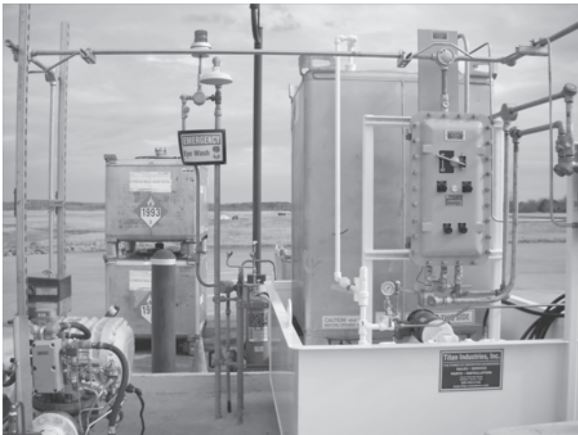
An additive injector and additive tank setup at Little Rock Air Force Base, Ark., which will be used to additize Jet A fuel.
