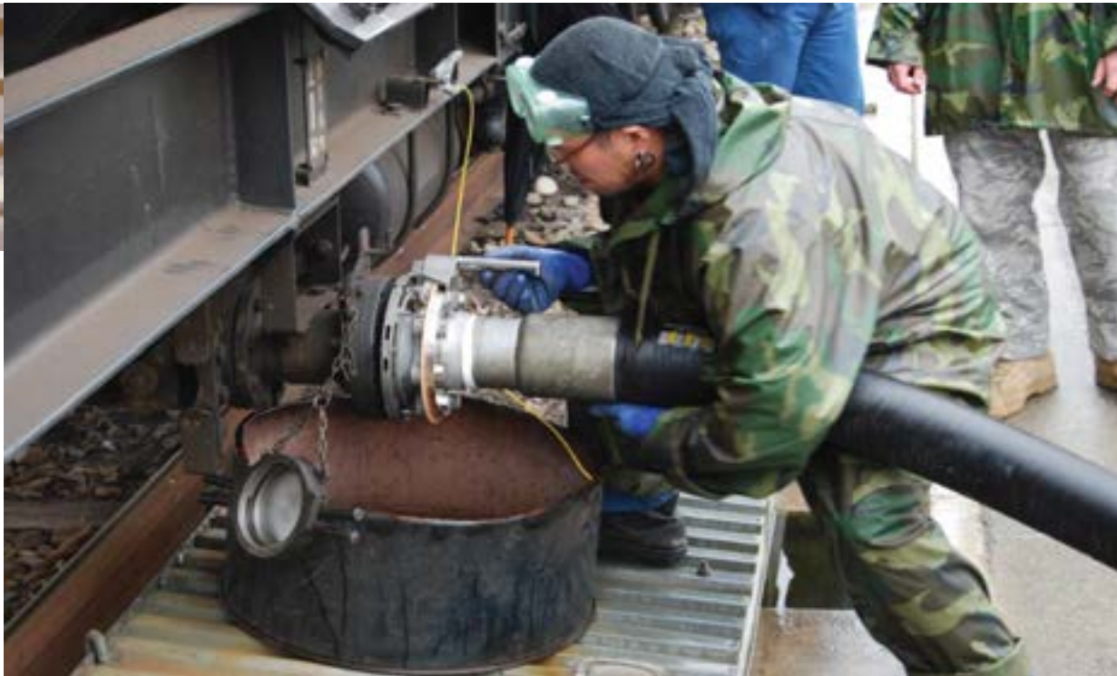
QUICKER Connection installed on rail car manifold and receipt hose line is demonstrated at Yokota Air Base, Japan. Photo courtesy of DLA Energy Pacific.
