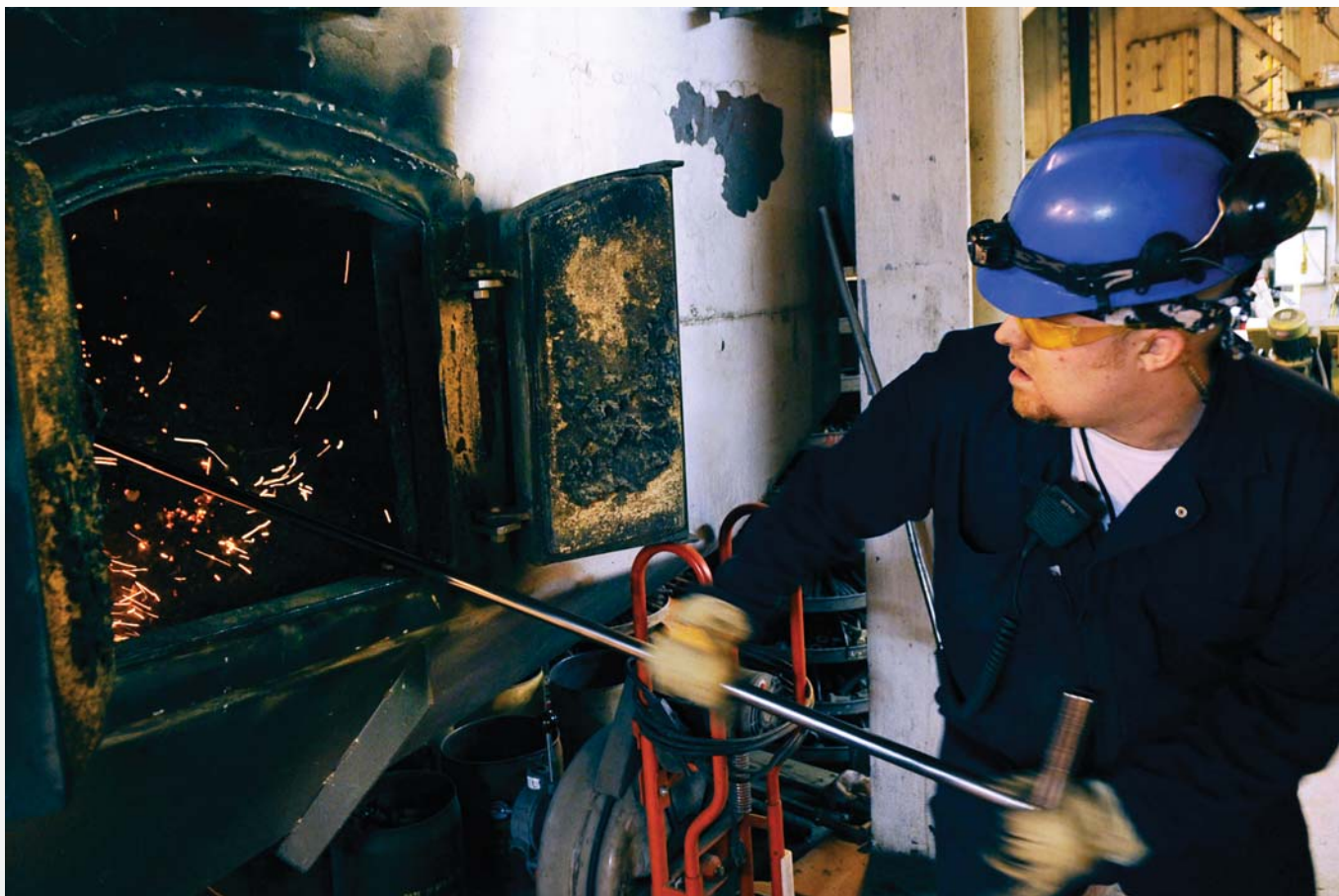
An ash puller clears a furnace at the Eielson Air Force Base, Alaska, Central Heat and Power Plant. DLA Energy Installation Energy provides Defense Department facilities with coal through its Natural Gas Program. Photo by Air Force Staff Sgt. Jim Araos
