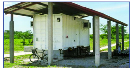
The Volpe Center designed and built this transmitter station for the port of San Lorenzo in Honduras, modifying an ISO shipping container. A differential GPS radio beacon, in concert with Volpe-developed mobile navigation units, allows harbor pilots to accurately determine the position and progress of their own ships as they navigate narrow inland waterways.
