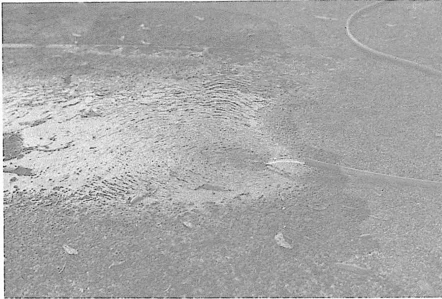
Figure 2. Initial surface ponding of water after rapid flooding
