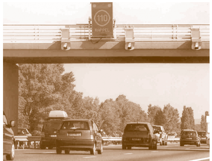
Figure 13. Enforcement cameras and speed limit signage on the A7. (French Ministry of Transport)
