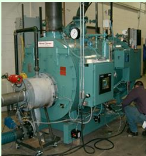
Figure 5.5 Laboratory Prototype Boiler (Rabovister and Knight, 2005)
