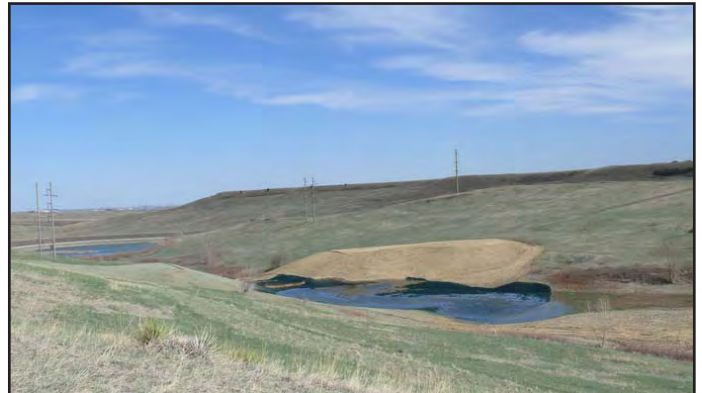
Dam A-3 following completion. The former pond bottom has been seeded with native wetland species and the disturbed areas have been reseeded with native grasses and covered with either a spray-on mulch or erosion matting.
