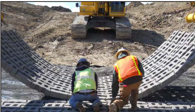
Workers position the pieces of articulated concrete armor to provide erosion control. The concrete armor encourages the establishment of vegetation in the channel.
