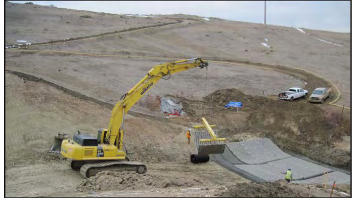
A track hoe with boom attachment is used to place the articulated concrete armor in the dam breach channel.
