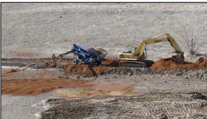
A "soil slinger" was used in some areas to evenly fill the bowl-shaped pond bottom with soil removed during the dam excavation.
