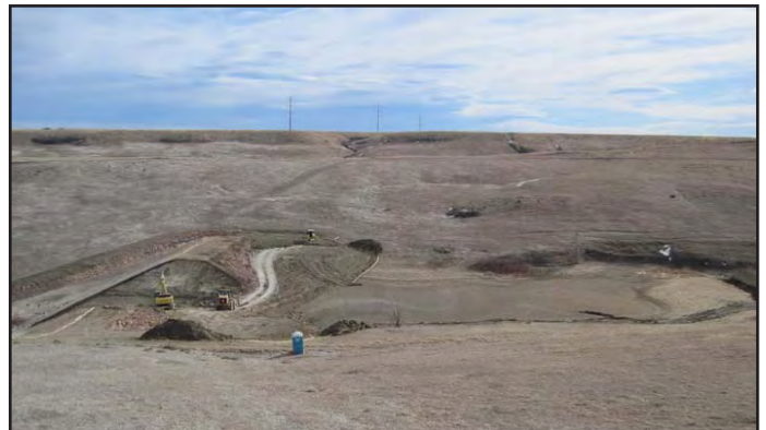
Heavy equipment is used to excavate a notch in the dam to create a channel for surface water flow.
