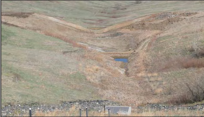
The Present Landfill (PLF) dam breach excavation is nearly complete. In the foreground the coffer dam retains water that flows from the PLF Treatment System. Once the breach is completed, the treated water will flow into No Name Gulch.
