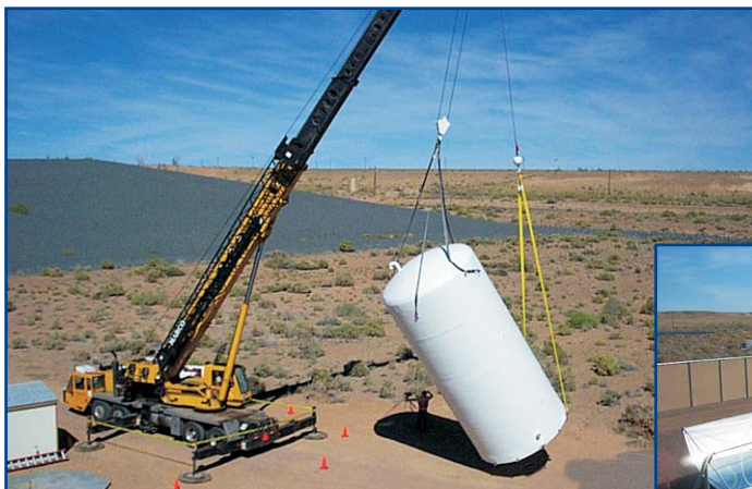
A crane is utilized to install the 20,000 gallon insulated hot water storage tank.
