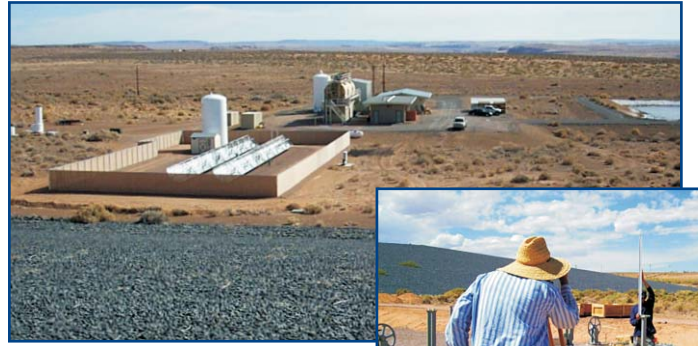
The solar hot water system is estimated to reduce the amount of electricity used to operate the Tuba City Site groundwater treatment system by 15 percent.
