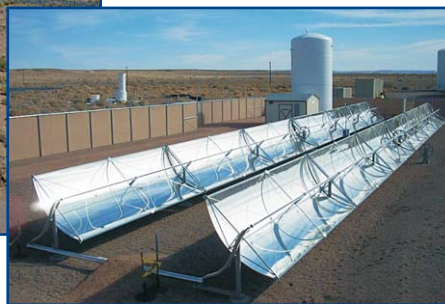
The parabolic mirrors focus solar energy to preheat the water to 170 degrees before it goes into the treatment system.
