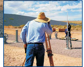
Surveyors mark the precise location to install the solar thermal parabolic mirrors to maximize efficiency.
