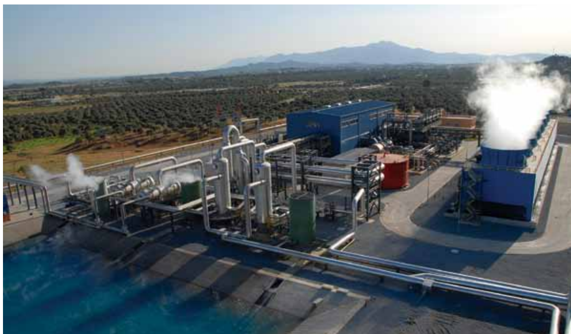
Based on a USTDA study, over 40 MW of new geothermal power was brought online in Germencik, Turkey utilizing more than $23 million in U.S. exports.
