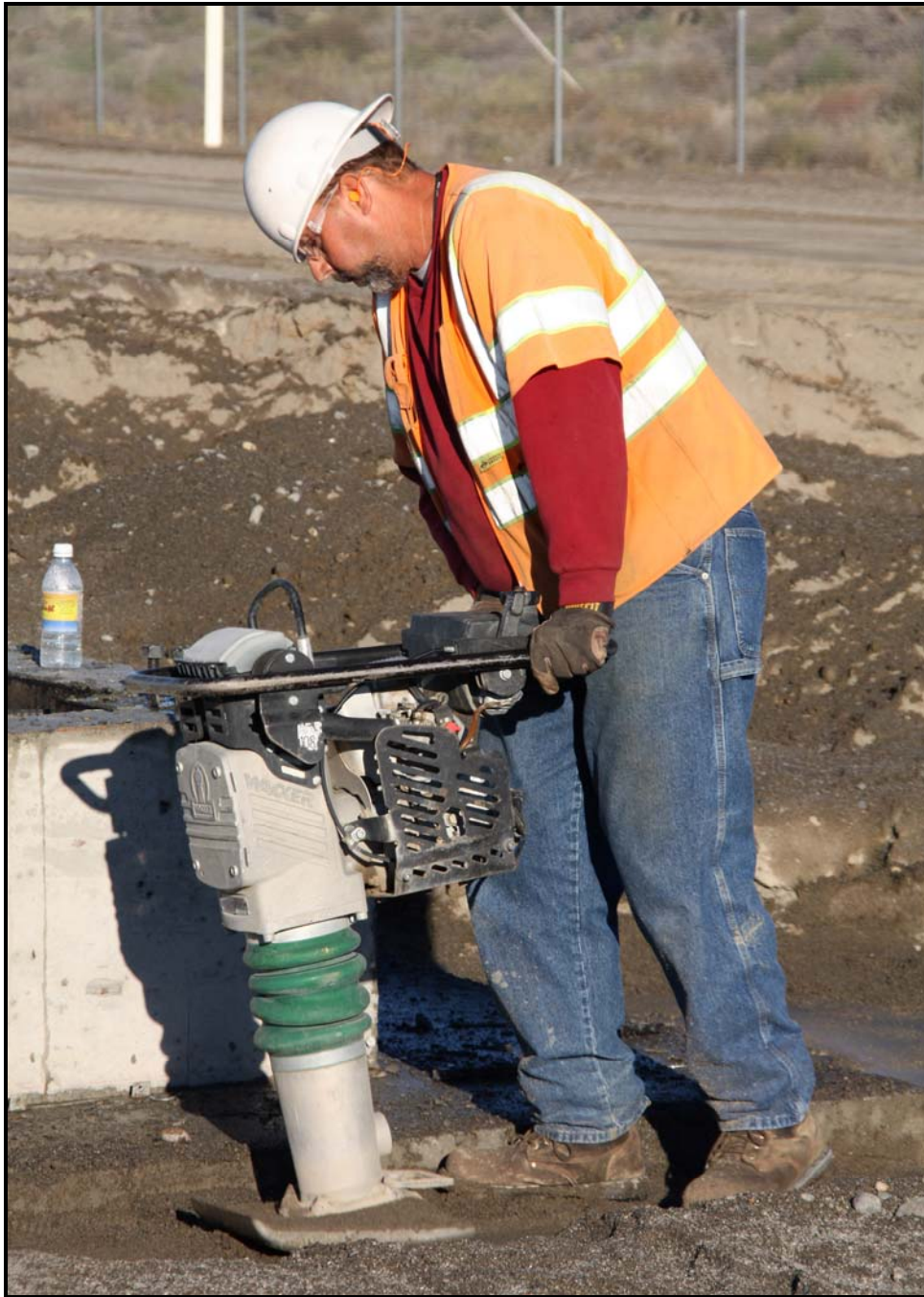
An employee with subcontractor Fowler General Construction works to compact the soil around the foundation of the container maintenance facility. (Photo 3)
