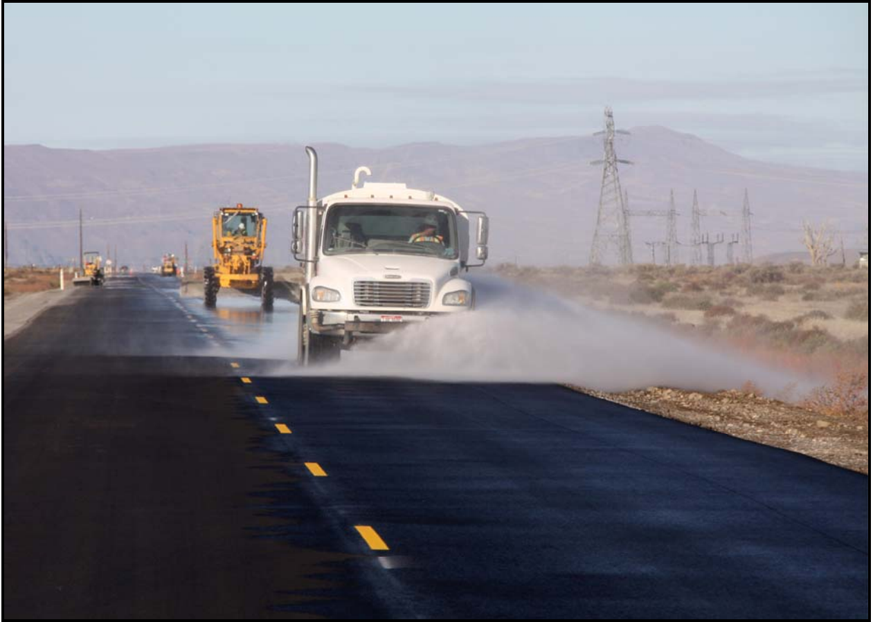
Washington Closure Hanford subcontractor Fowler General Construction completes shoulder work on Route 1, one of three Hanford Site roads being repaired. Route 1 is scheduled to open next week. (Photo 4)
