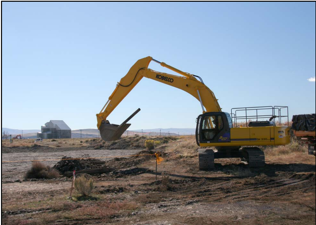
Washington Closure Hanford subcontractor Ojeda Business Ventures continues remediation excavation and loadout activities at site 100-F-48. (Photo 5)
