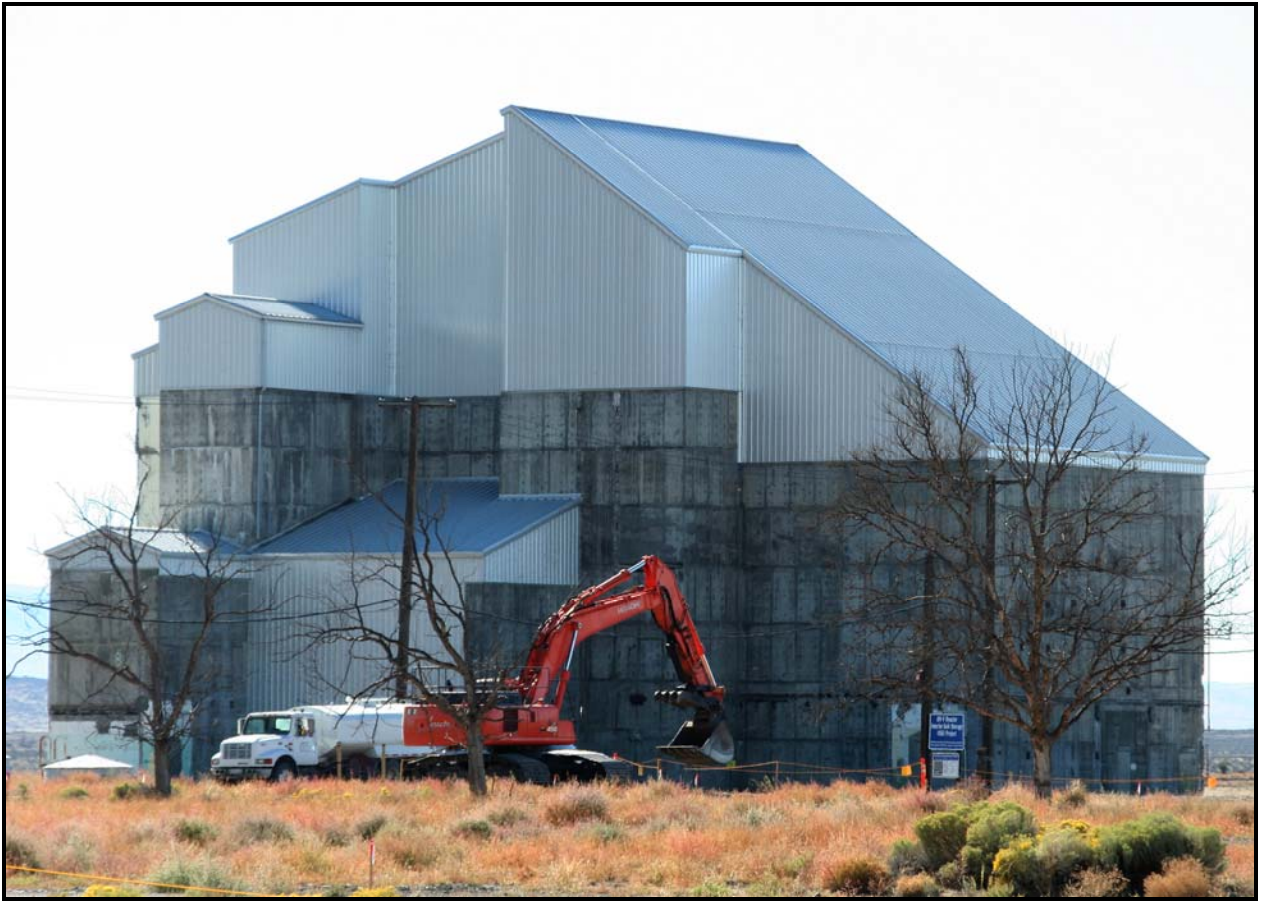
Potholing work to collect samples for the development of waste profiles continues at site 100-F-26:4, one of 18 waste sites to be remediated. (Photo 6)
