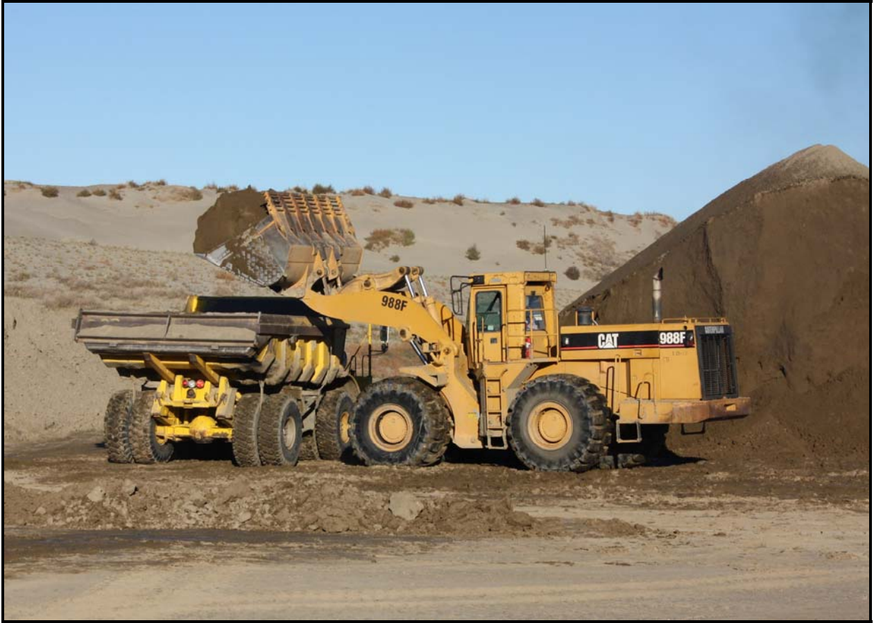
Admix is loaded into a dump truck for placement in super cell 10 at the Environmental Restoration Disposal Facility. (Photo 2)
