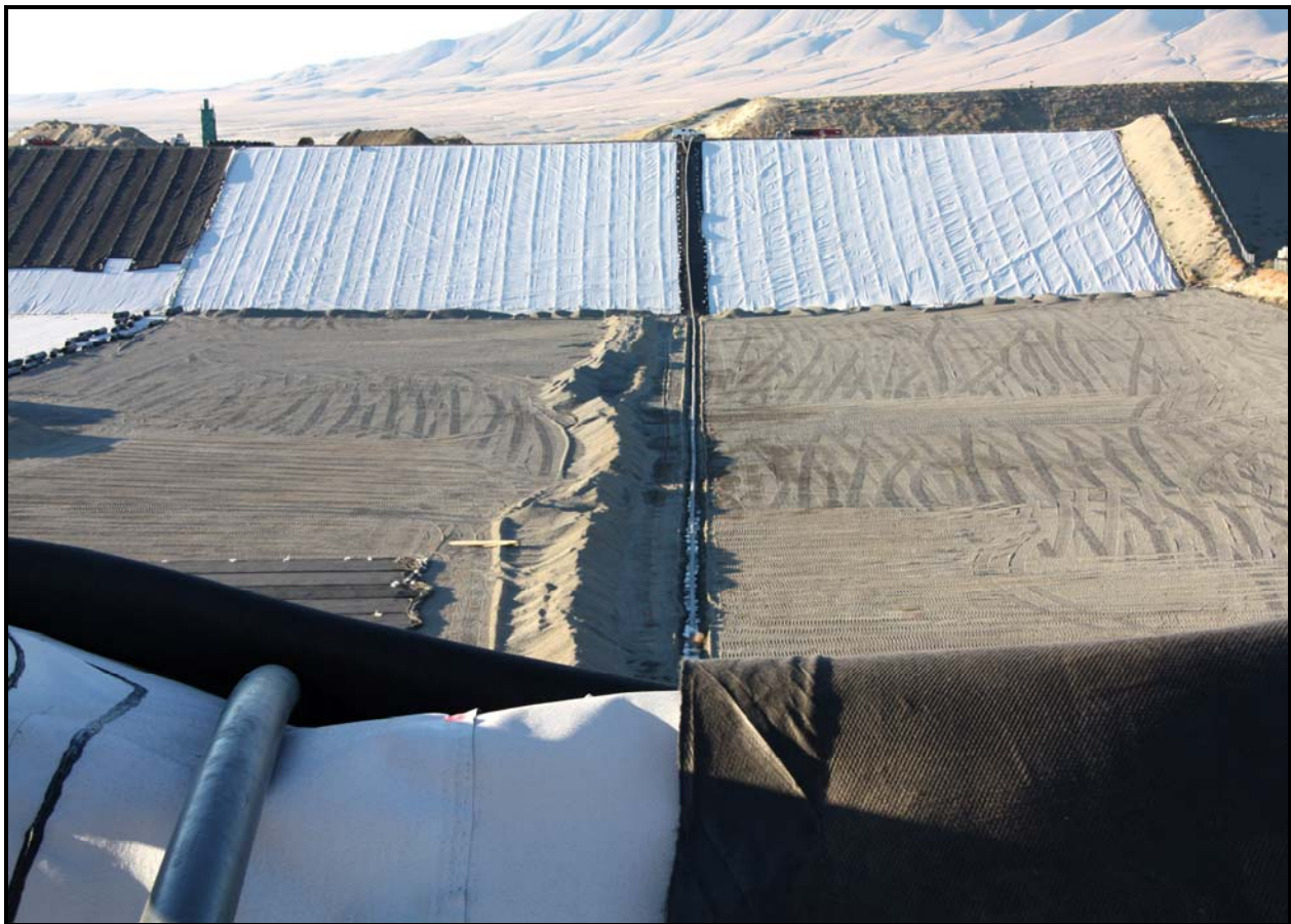
The leachate collection pipe (the length of super cell 9) is being installed at the Environmental Restoration Disposal Facility. (Photo 1)
