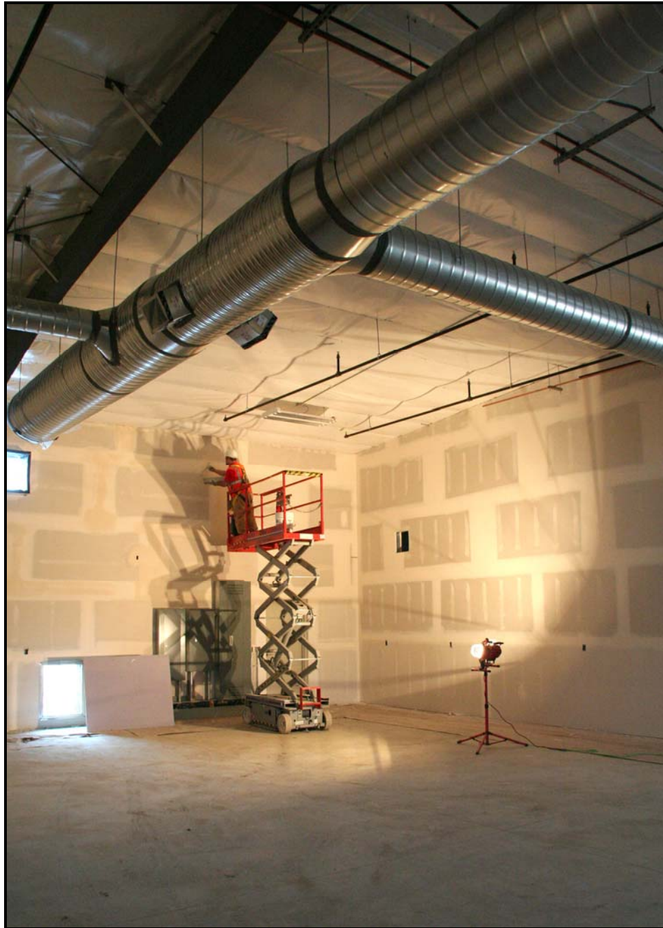
An ELRFowler employee tapes the drywall at ERDF's container maintenance facility. (Photo 4)
