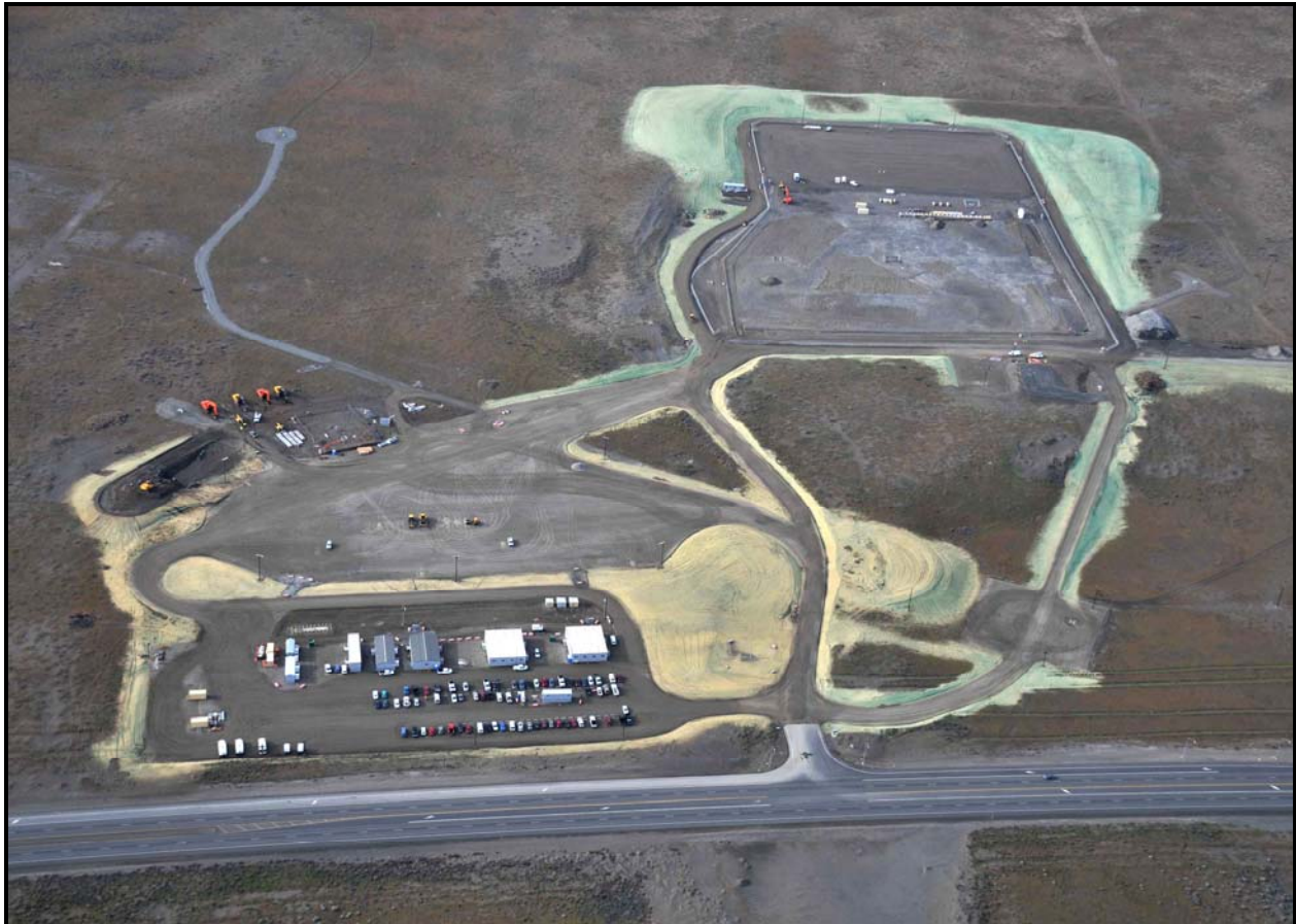
Washington Closure Hanford subcontractor White Shield/Apollo has nearly completed utility installation at the 618-10 Burial Ground. The project team is scheduled to begin field activities next week. (Photo 6)
