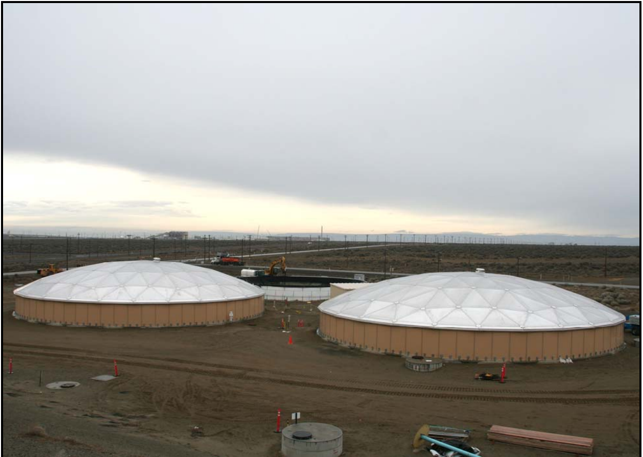
Construction of the two leachate storage tanks and their dome covers was completed at the Environmental Restoration Disposal Facility. (Photo 2)
