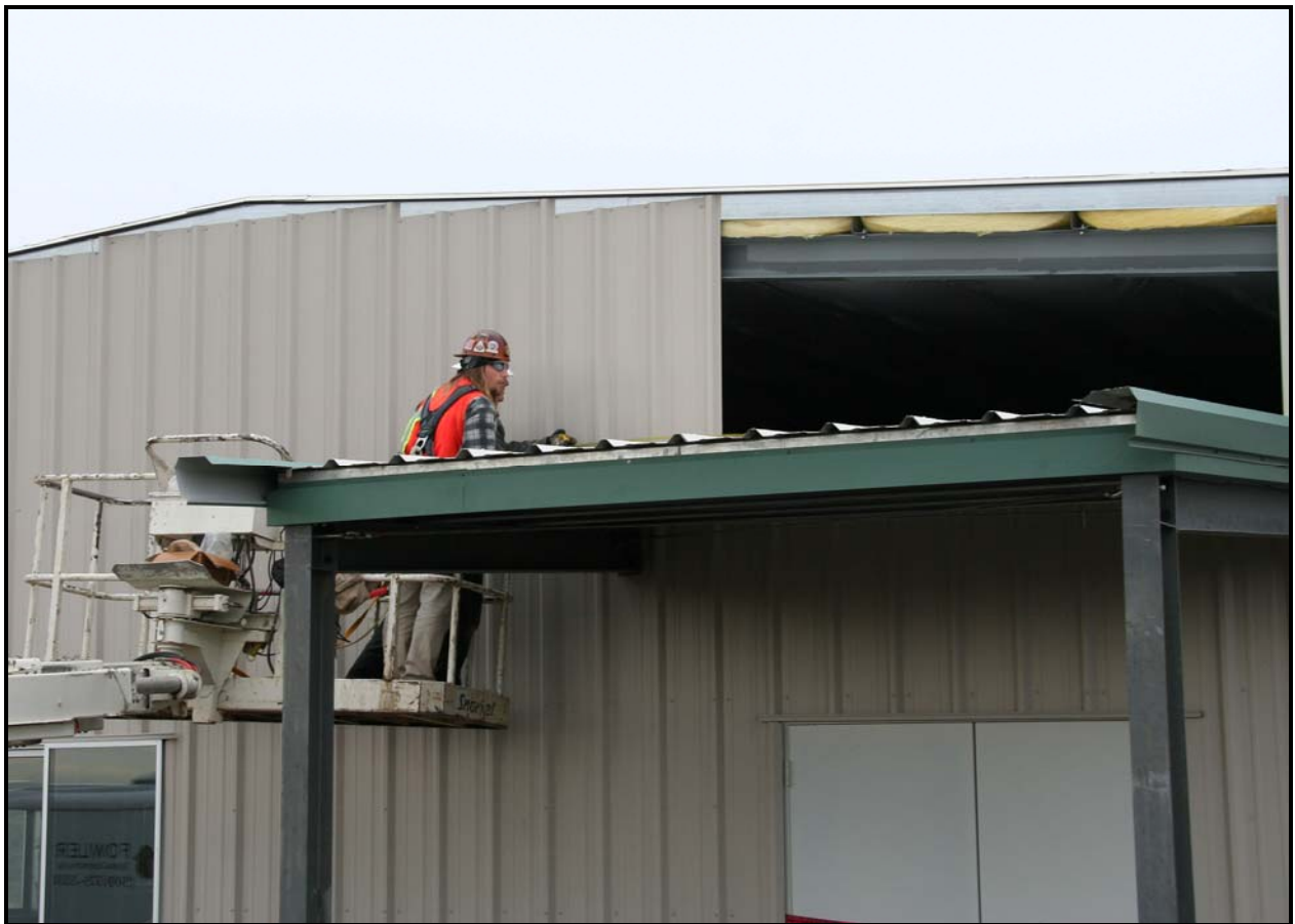
An employee with Washington Closure Hanford subcontractor ELRFowler installs siding on the west side of ERDF's equipment maintenance facility/operations center. (Photo 3)
