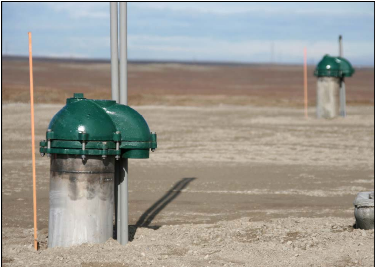
Washington Closure Hanford is installing wells at the 618-10 Burial Ground where remediation activities are scheduled to begin this month. (Photo 5)
