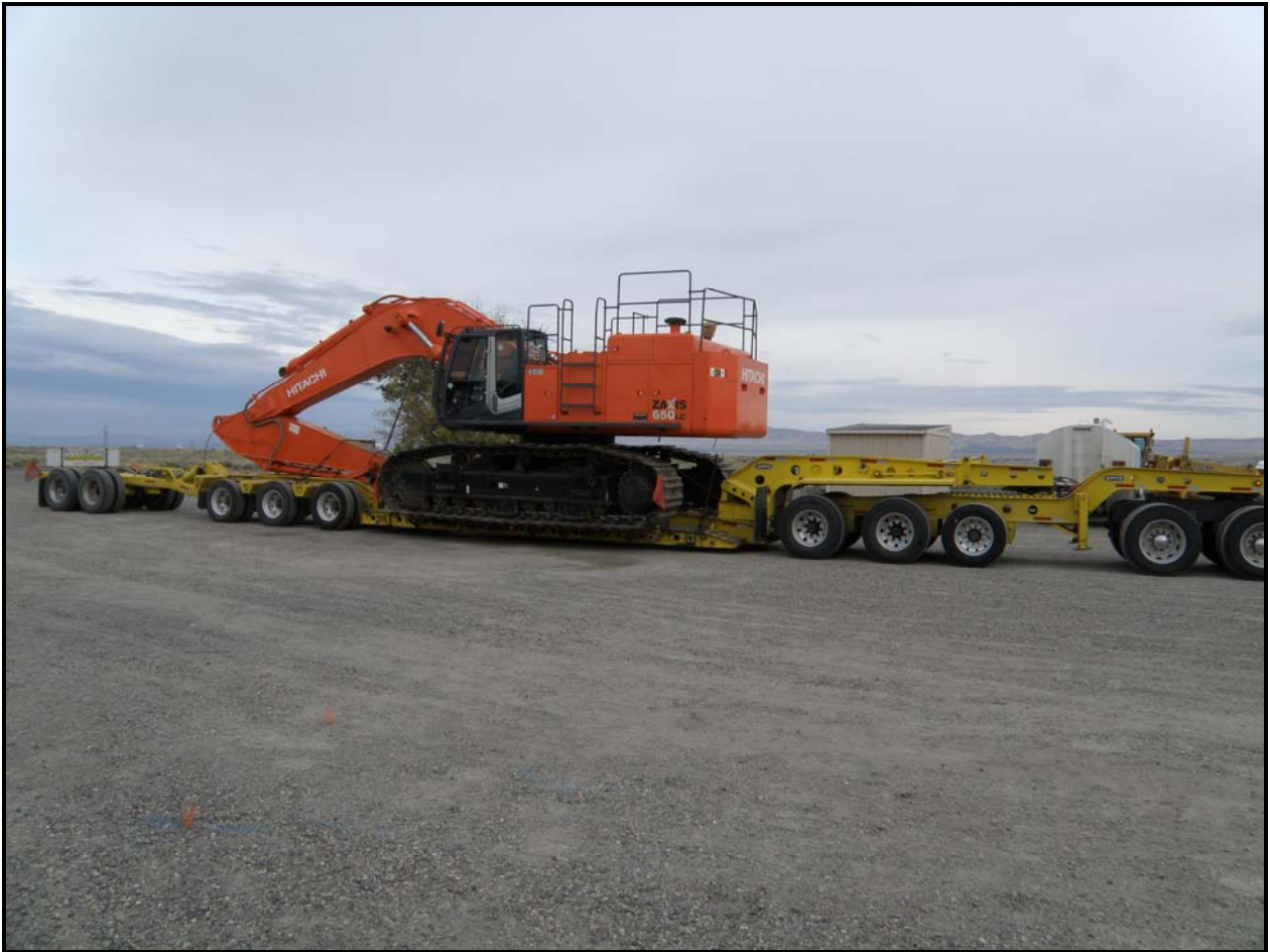
An excavator is delivered to 100-F Area as Washington Closure Hanford subcontractor Ojeda Business Ventures continues mobilization activities.
