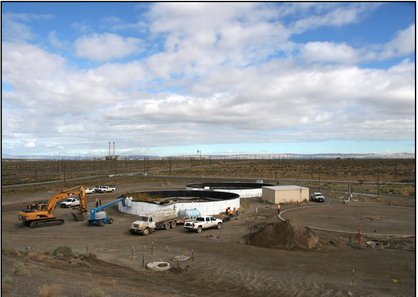
One of the original leachate collection tanks for ERDF is being demolished to make way for a new, larger leachate collection tank. ERDF produces about 100,000 gallons of leachate a month.
