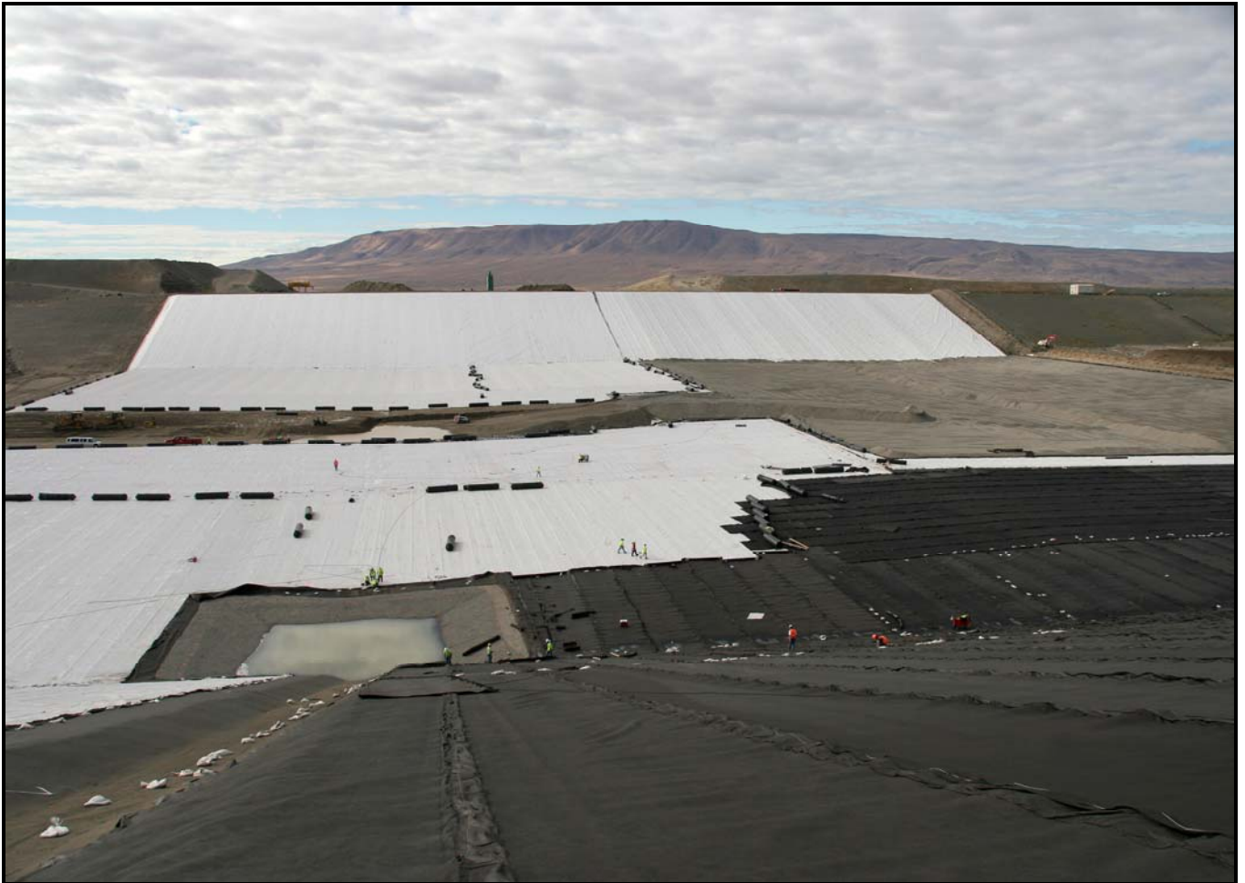
The installation of the geocomposite layer for super cell 9 was completed last week at the Environmental Restoration Disposal Facility.
