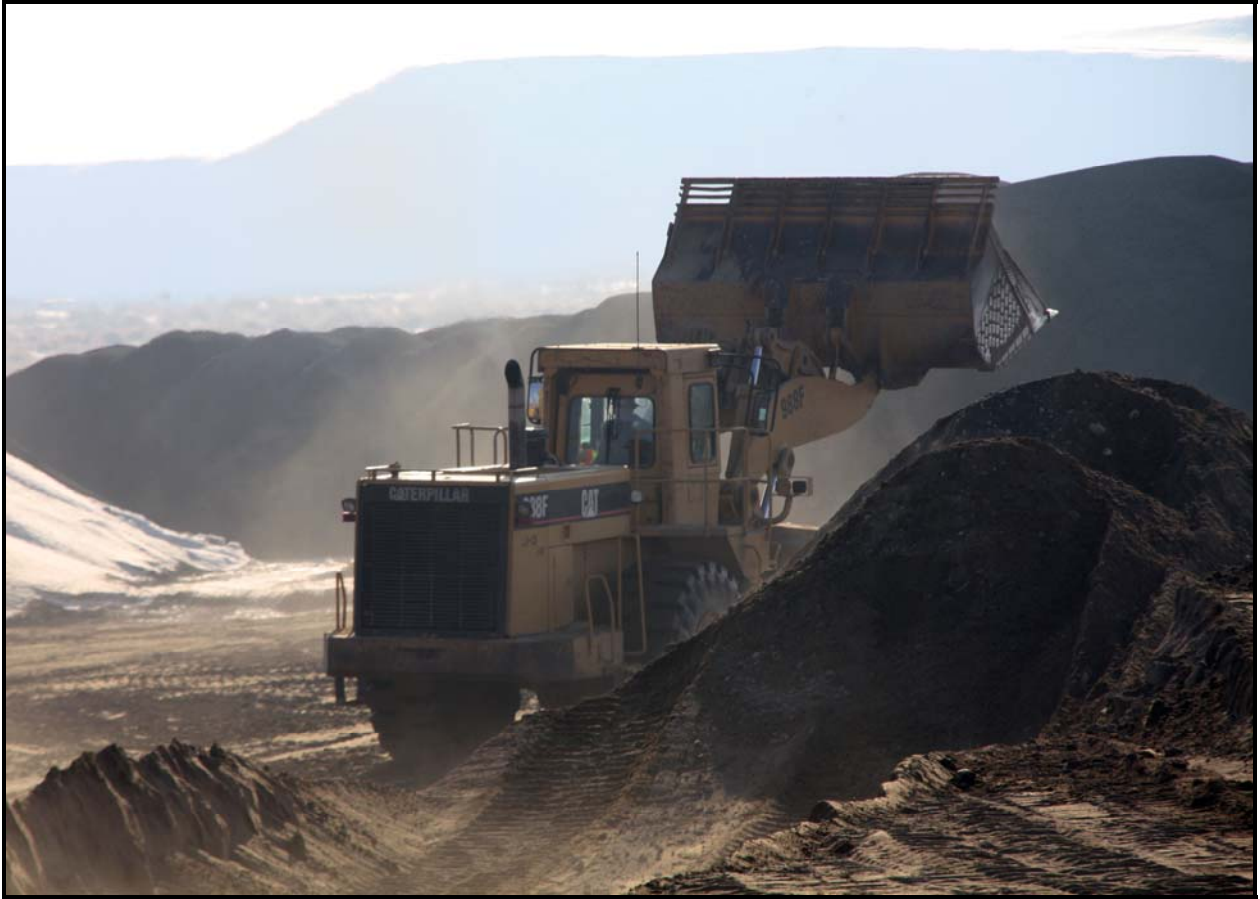
DelHur Industries personnel work on the site of the expanded container transfer area at the Environmental Restoration Disposal Facility. (Photo 4)
