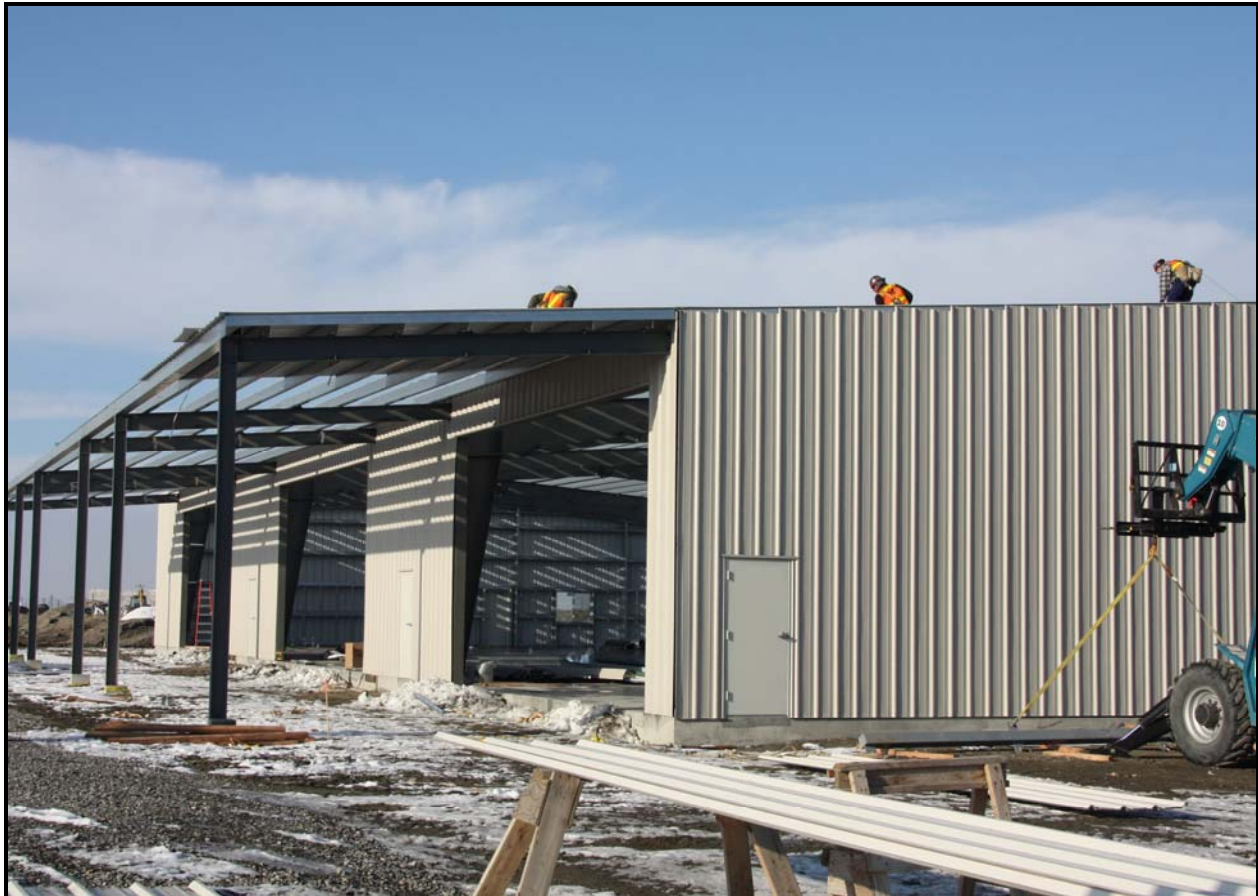
Washington Closure Hanford subcontractor Fowler General Construction employees work to construct the roof at ERDF's container maintenance facility. (Photo 3)
