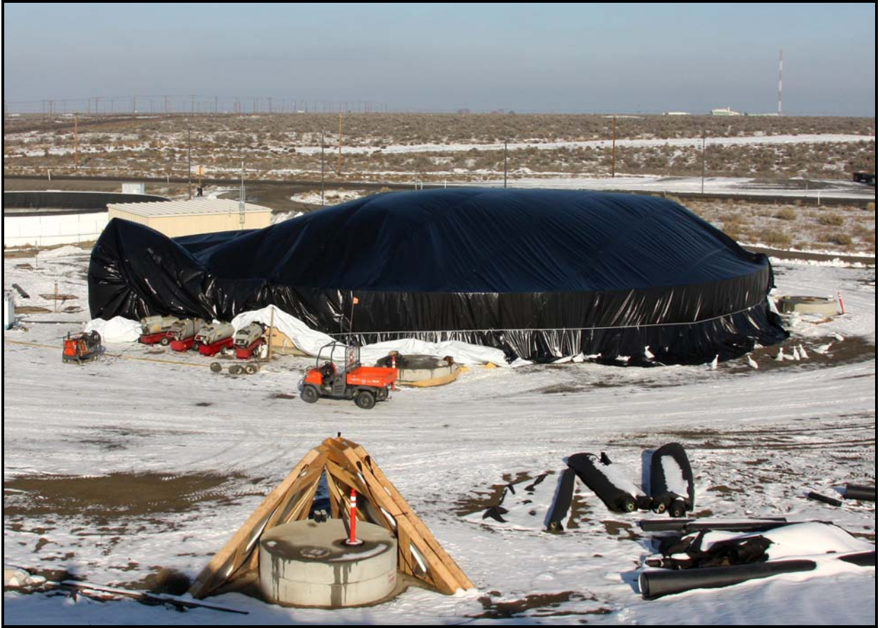
Work continues on the new leachate storage tanks at the Environmental Restoration Disposal Facility. A weather enclosure was constructed to allow liner construction to resume in leachate storage tank No. 3. (Photo 1)
