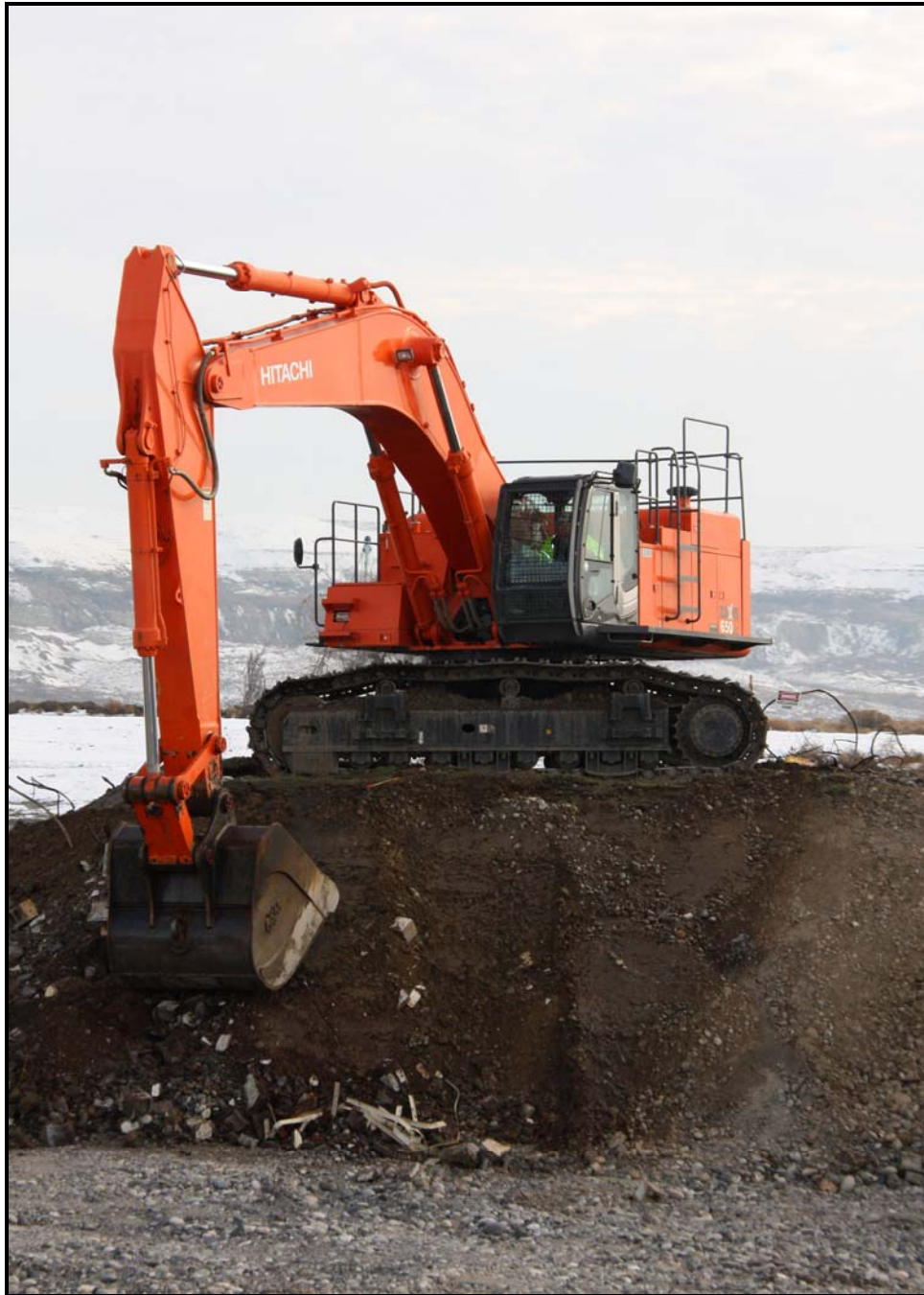
Ojeda Business Ventures continues excavation and loadout activities at 100-F-48, which contains coal pit debris. (Photo 9)
