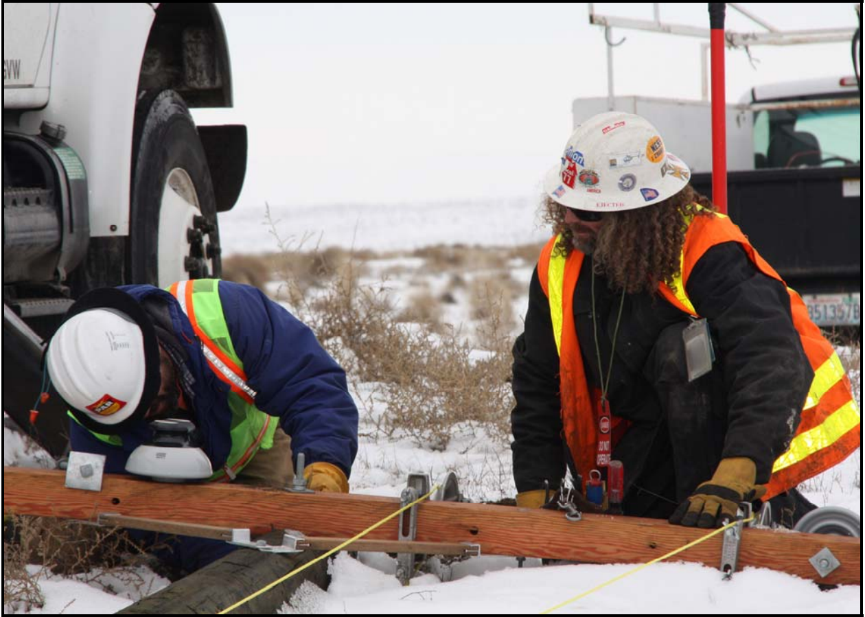
White Shield/Apollo workers prepare a power pole for installation at the 618-10 Burial Ground. (Photo 7)
