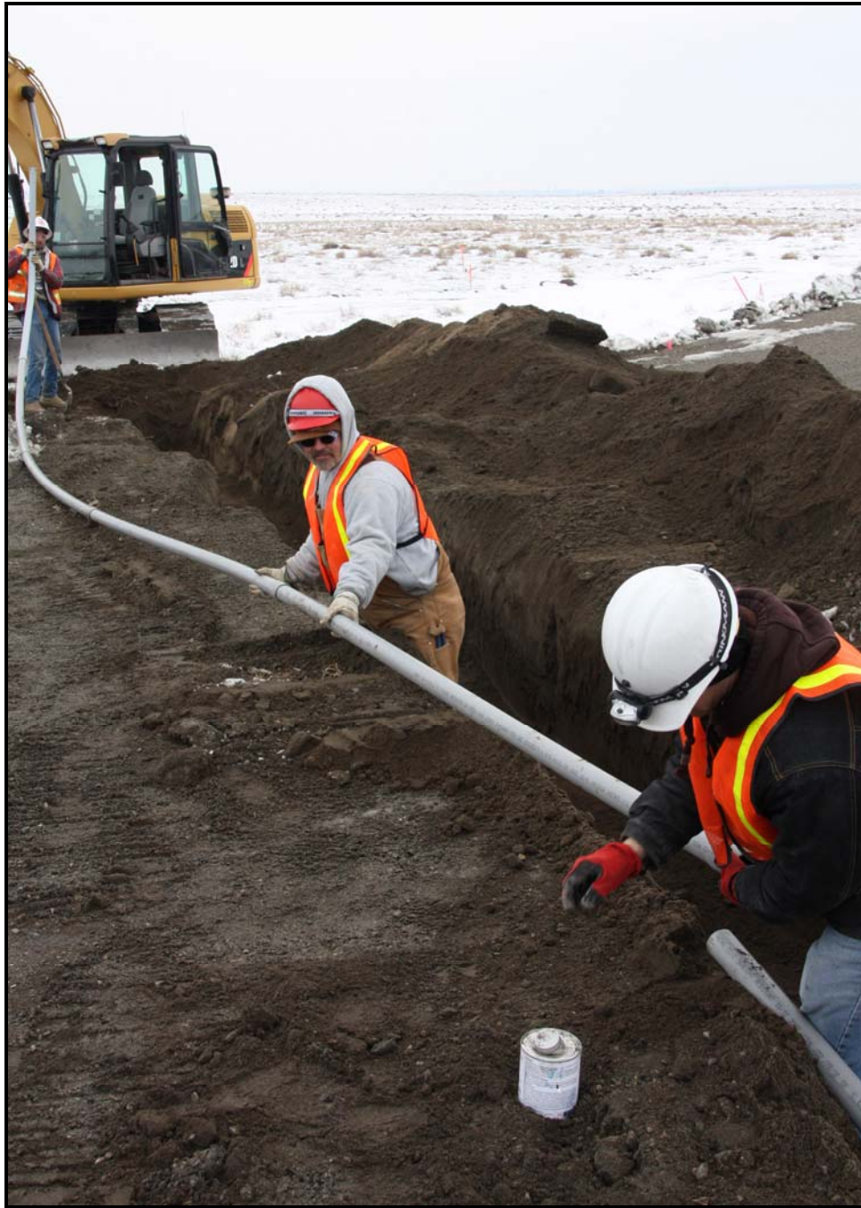
Washington Closure Hanford subcontractor White Shield/Apollo workers install electrical conduit at the 618-10 Burial Ground. (Photo 5)
