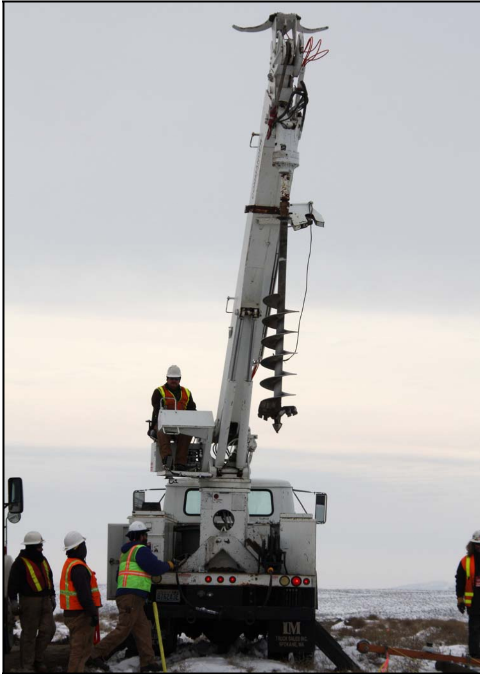
White Shield/Apollo workers use an auger to bore a hole for a power pole at the 618-10 Burial Ground. (Photo 6)
