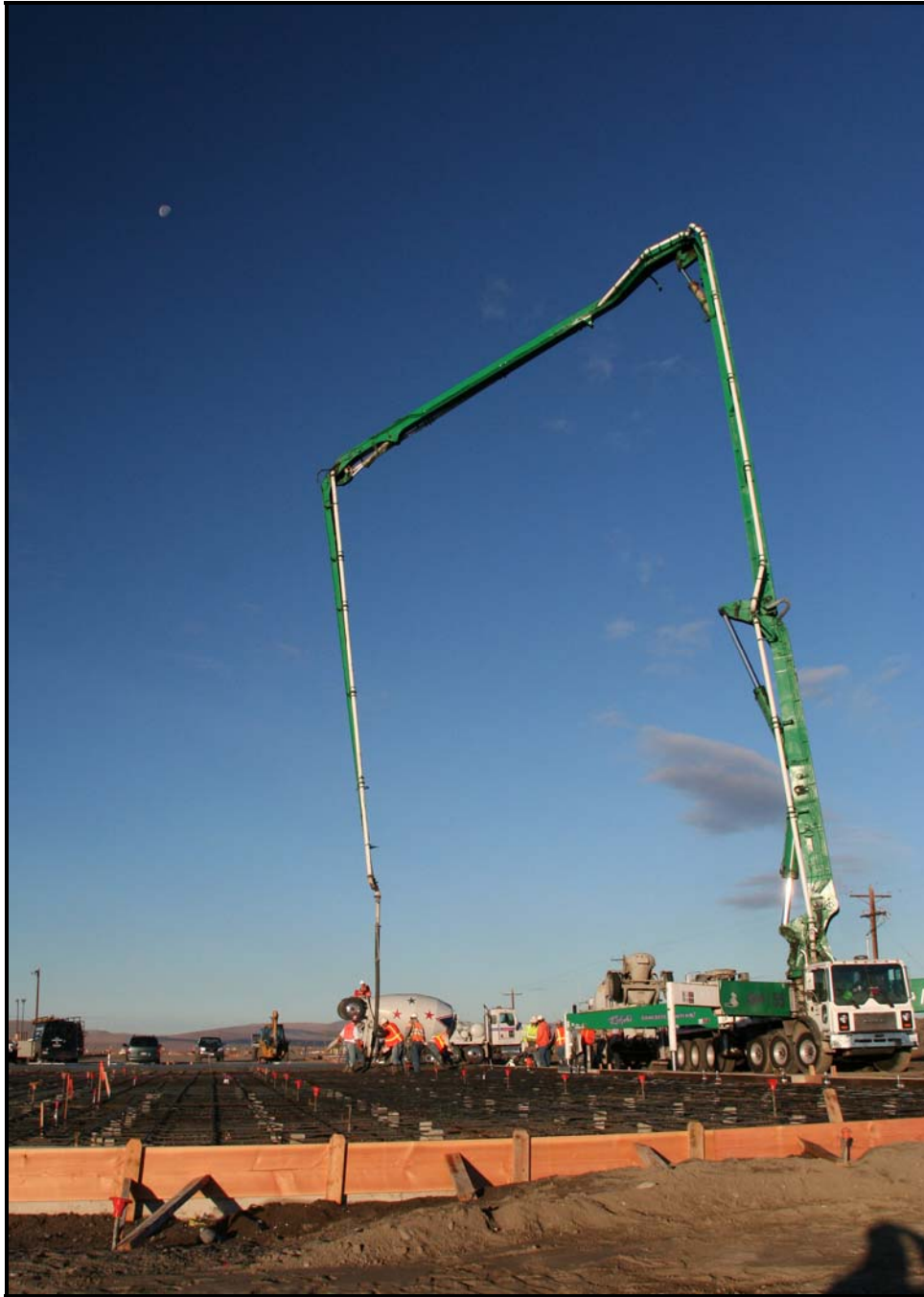
Workers begin to pour the concrete slab at the Environmental Restoration Disposal Facility's container maintenance facility. (Photo 2)
