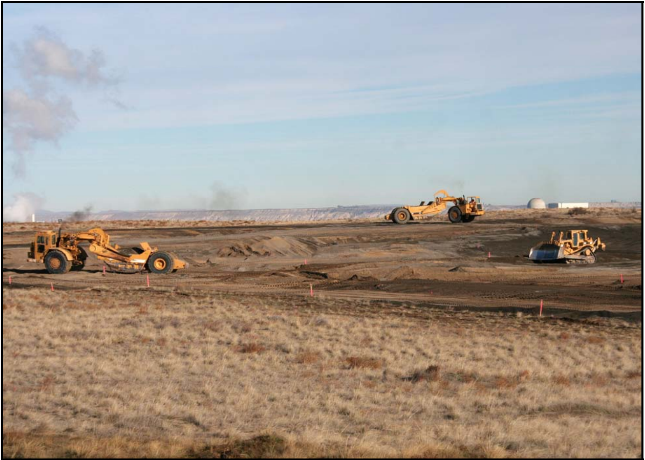
White/Shield Apollo continues construction of site roads at the 618-10 Burial Ground. (Photo 7)
