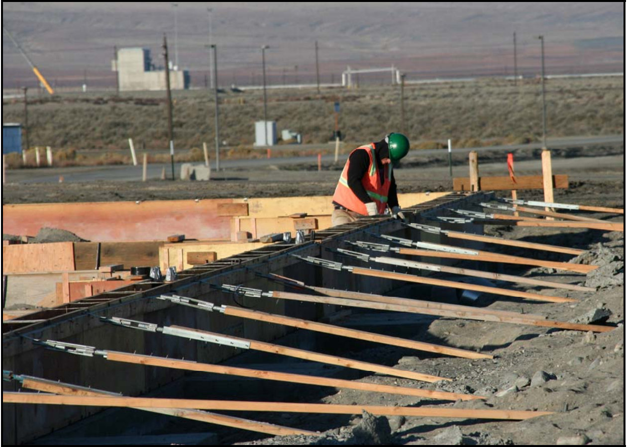
Fowler General Construction continues to construct the stem walls at the Environmental Restoration Disposal Facility's maintenance facility/operations center. (Photo 5)
