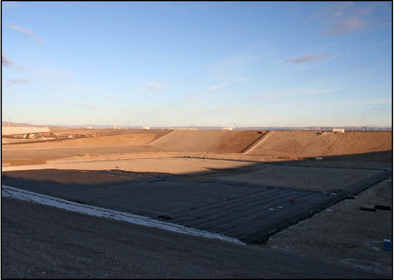
A view from the southeast corner of the Environmental Restoration Disposal Facility shows liner construction progress in super cells 9 and 10. (Photo 1)
