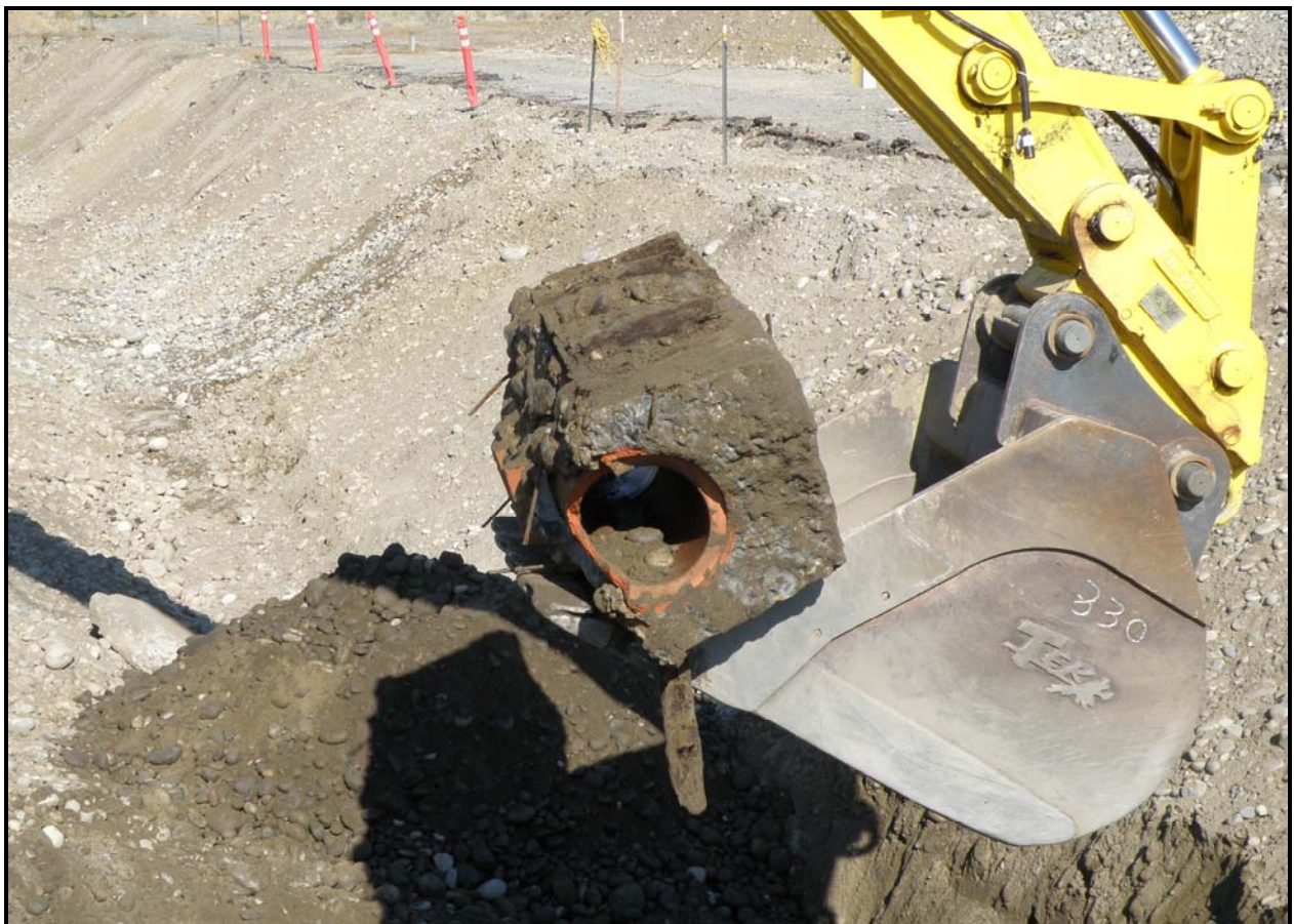
Washington Closure Hanford subcontractor Ojeda Business Ventures removes a section of processed sewer line at 100-F-26:4. (Photo 8)
