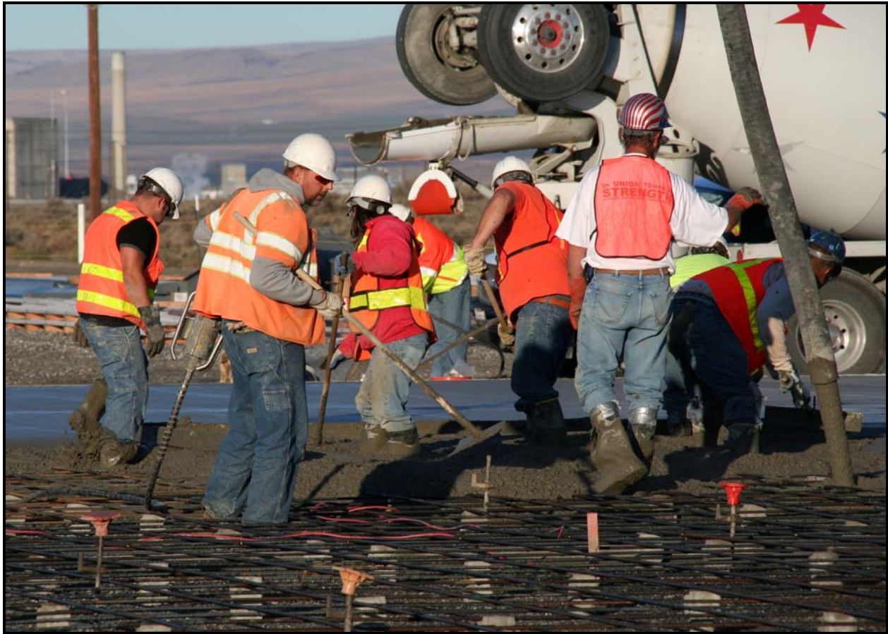
A team from Washington Closure Hanford subcontractor Fowler General Construction spreads concrete at the container maintenance facility. (Photo 3)
