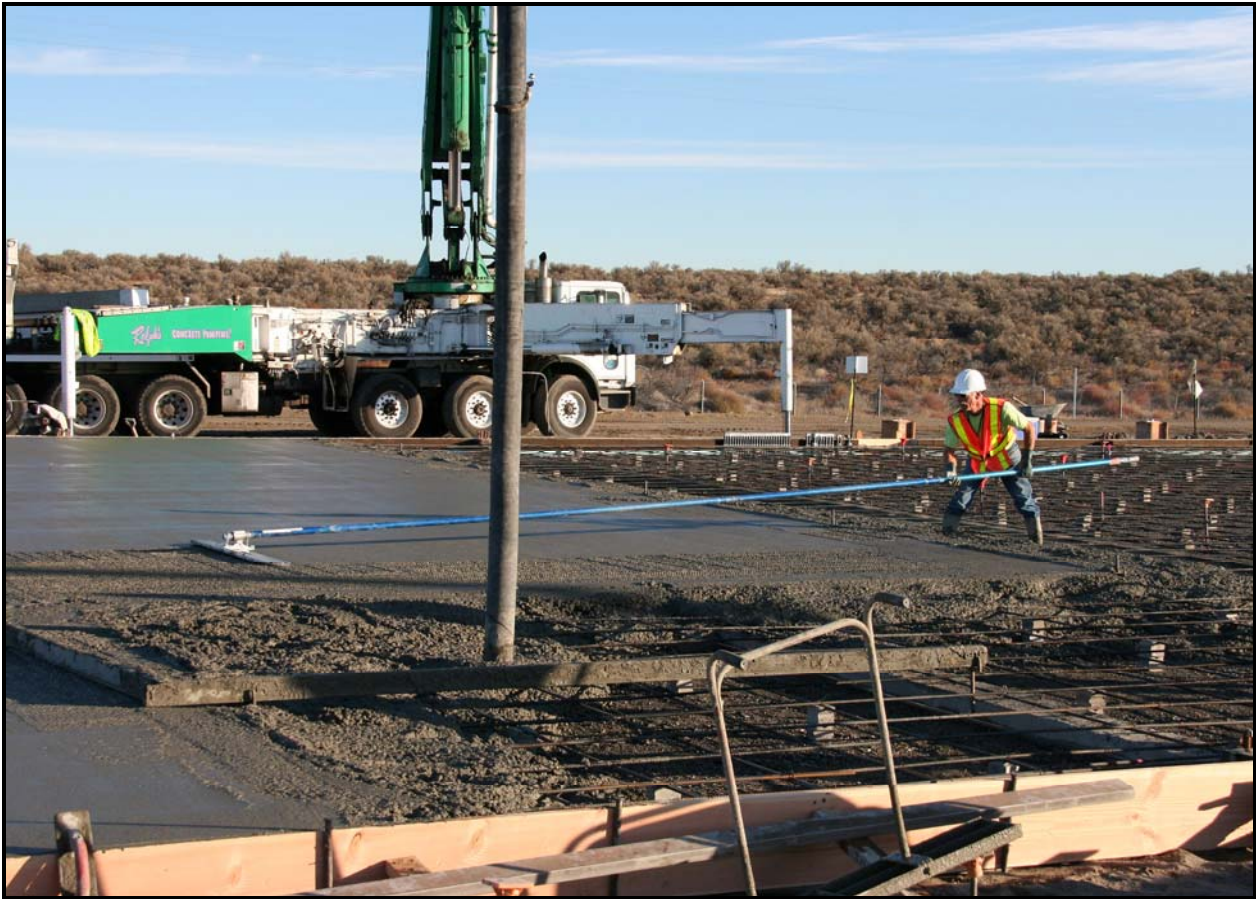
A Fowler General Construction employee works to smooth recently poured concrete at the container maintenance facility. (Photo 4)
