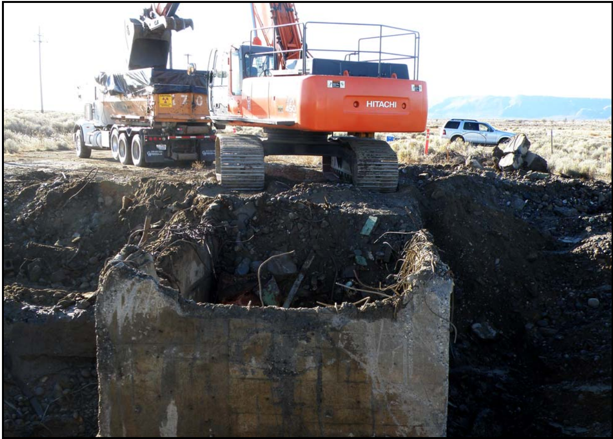
A transformer pad is exposed during remediation activities at 100-F-47 – an electrical substation foundation. (Photo 9)
