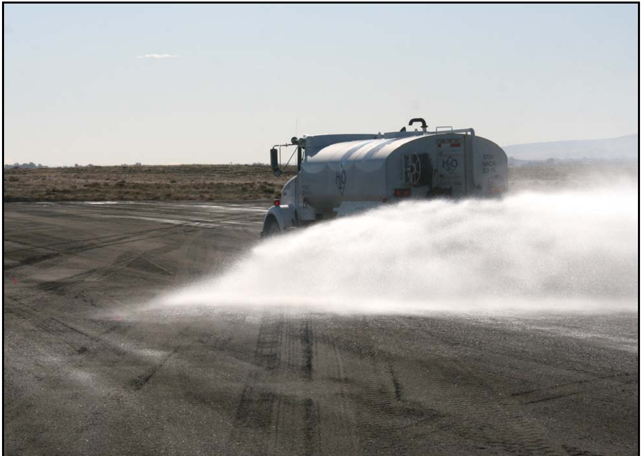
Washington Closure Hanford subcontractor White/Shield Apollo completed construction of the site to be used for office trailers at the 618-10 Burial Ground. (Photo 6)
