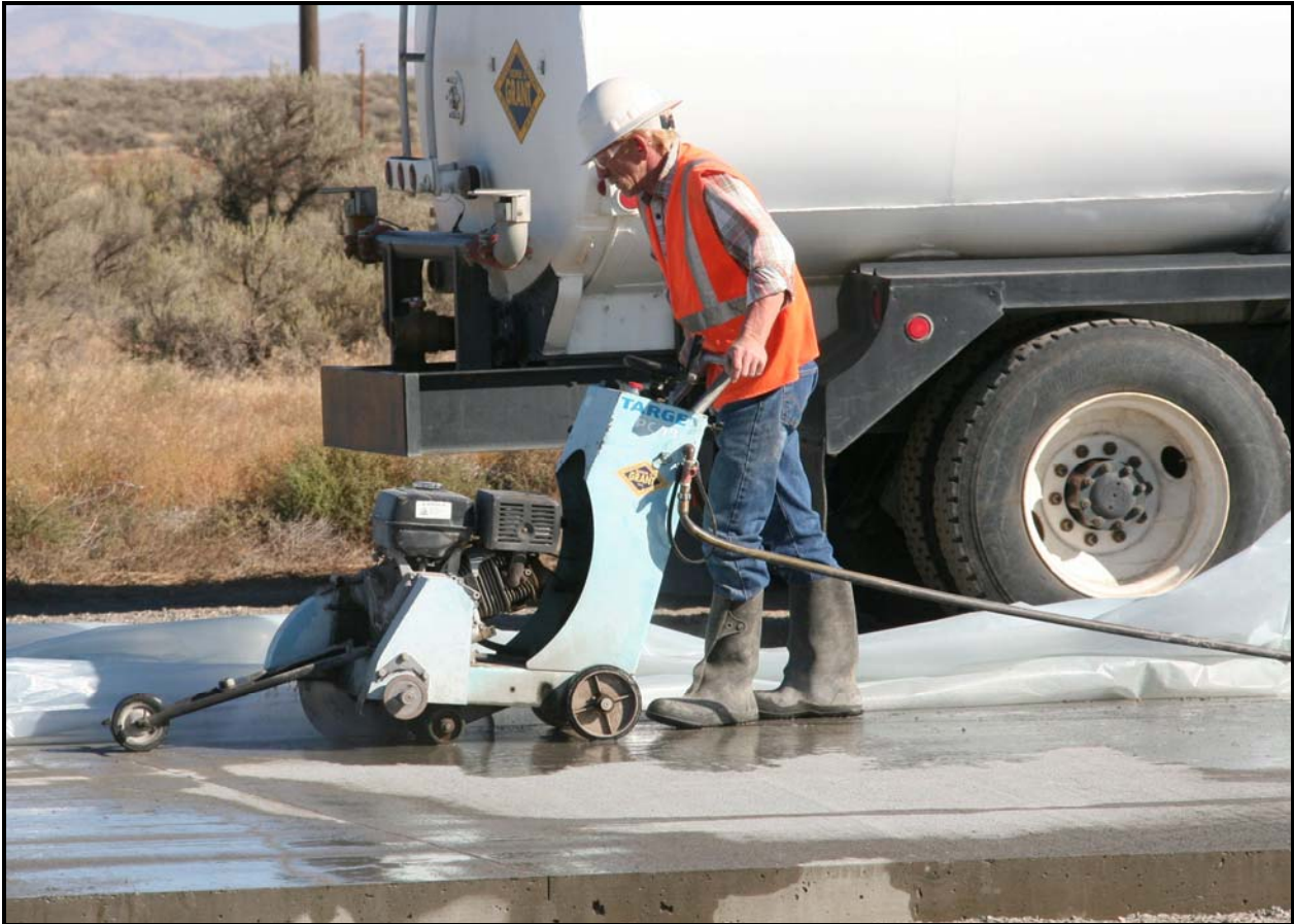
An employee with subcontractor Grant Construction works the 13 th Street upgrade at the Environmental Restoration Disposal Facility. (Photo 2)
