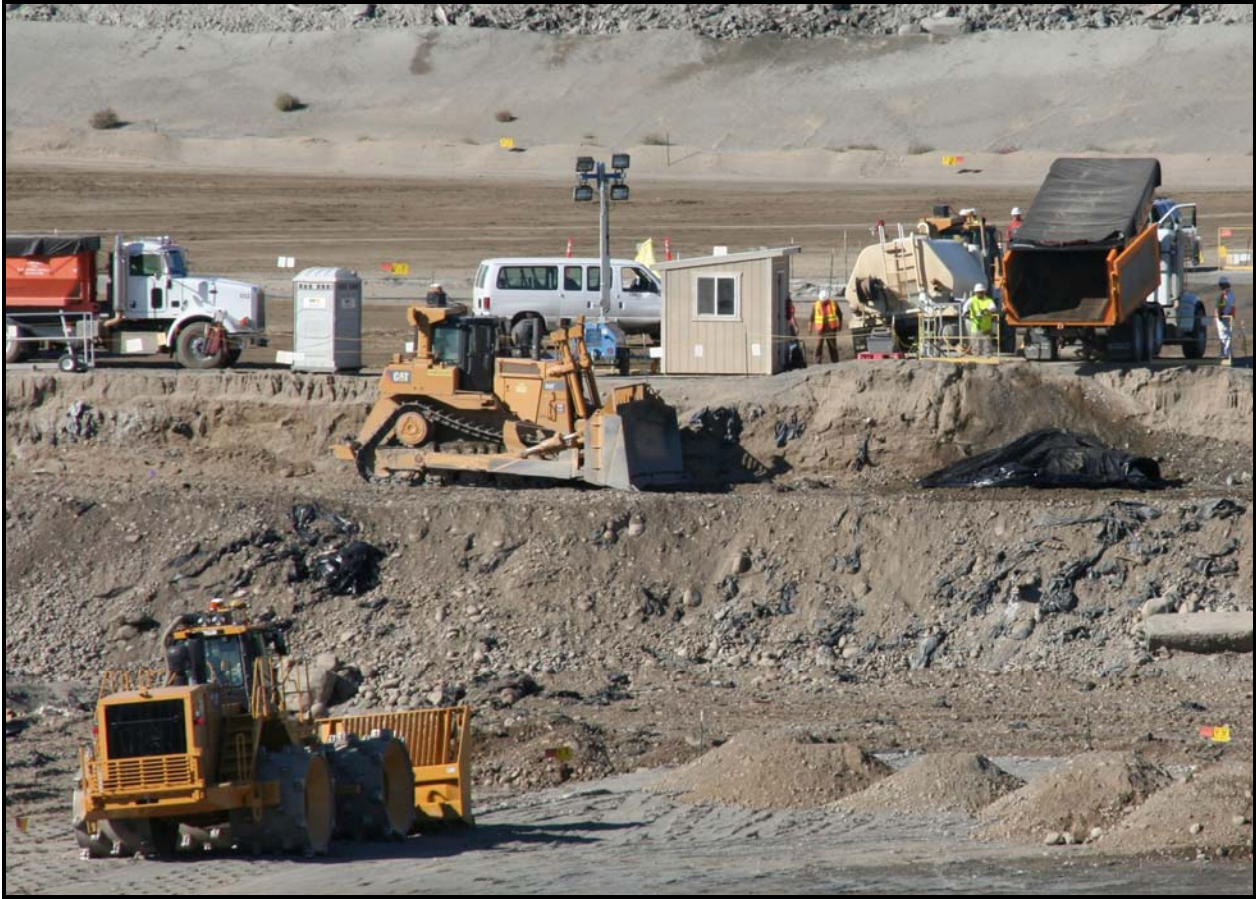
The Waste Operations team at the Environmental Restoration Disposal Facility disposed of a record 2.2 million tons of waste material this fiscal year, breaking the previous record of 1.6 million tons. Disposal operations are funded by Recovery Act dollars. (Photo 1)
