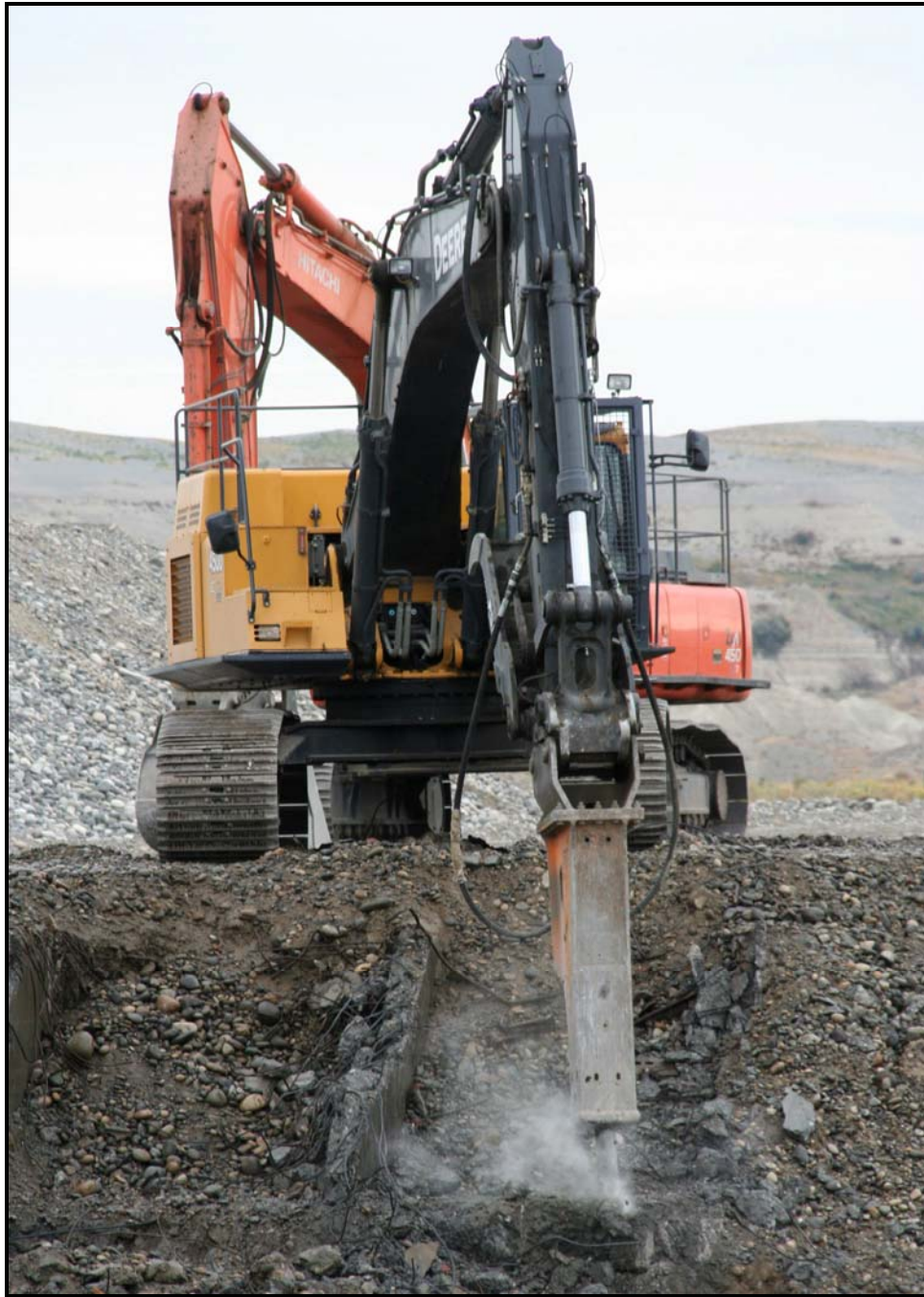
Washington Closure Hanford subcontractor Ojeda Business Ventures hammers concrete at 100-F-57. (Photo 4)
