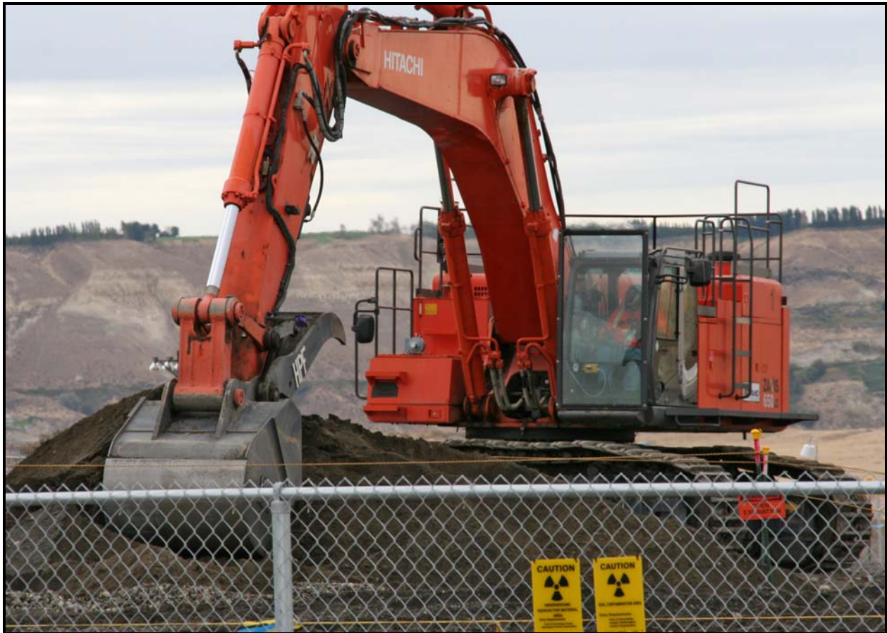
Washington Closure Hanford excavates the east-side waste trench at the 618-10 Burial Ground. (Photo 3)
