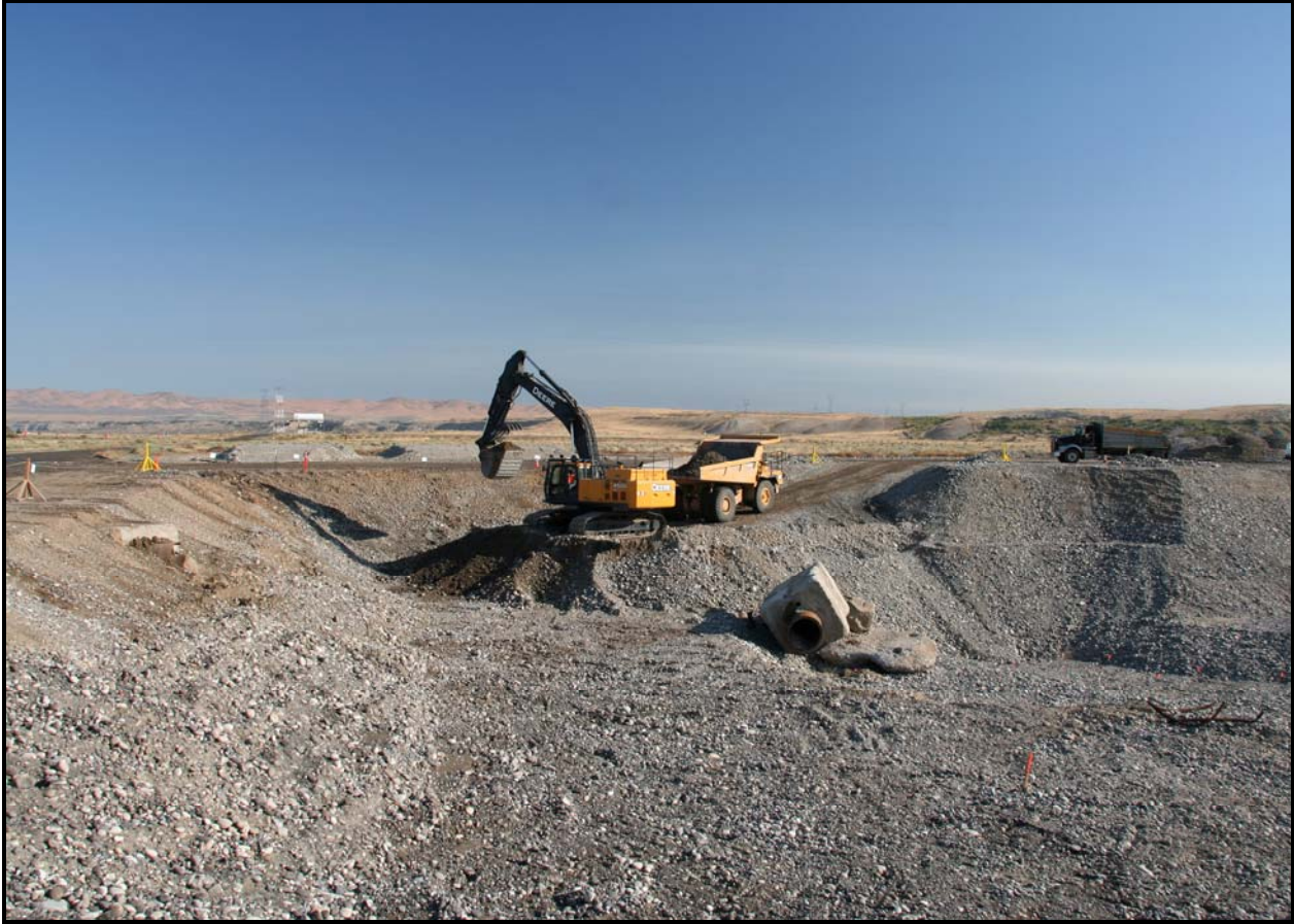
Washington Closure Hanford subcontractor Ojeda Business Ventures continues with excavation and loadout at 100-F-57. (Photo 4)
