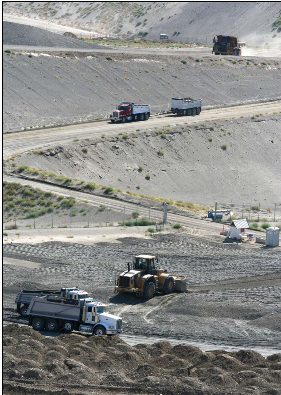
Waste material is transported for disposal in super cell 10 at the Environmental Restoration Disposal Facility. (Photo 1)
