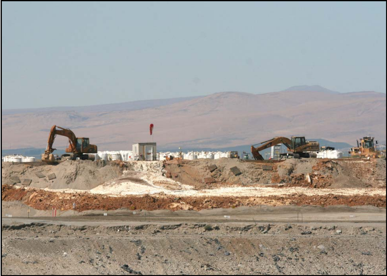
The Waste Operations team continues to treat chrome waste from 100-C-7 at the Environmental Restoration Disposal Facility. (Photo 2)
