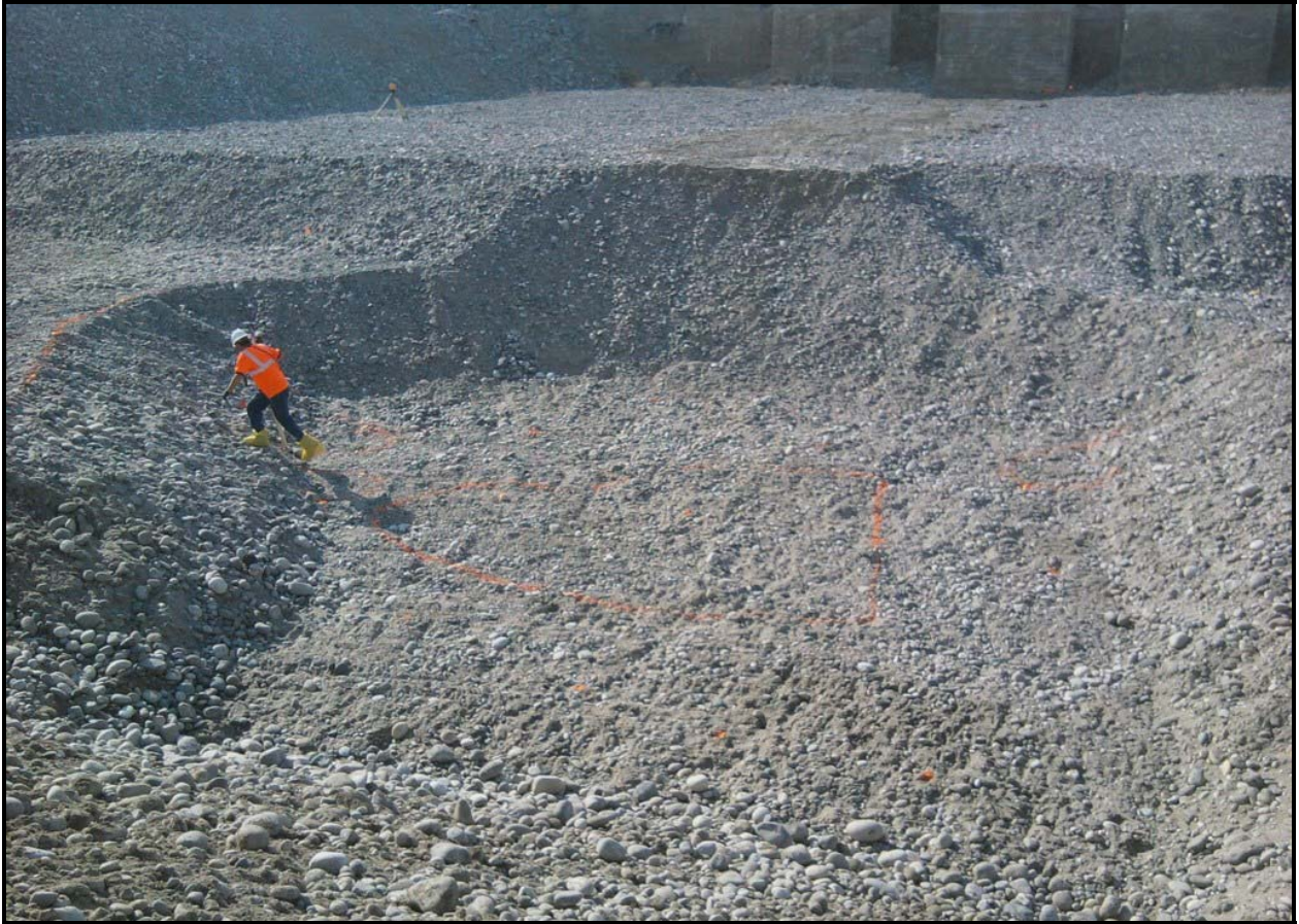
Washington Closure Hanford and subcontractor Ojeda Business Ventures excavated a section of 100-F-57 to 25 feet. (Photo 6)
