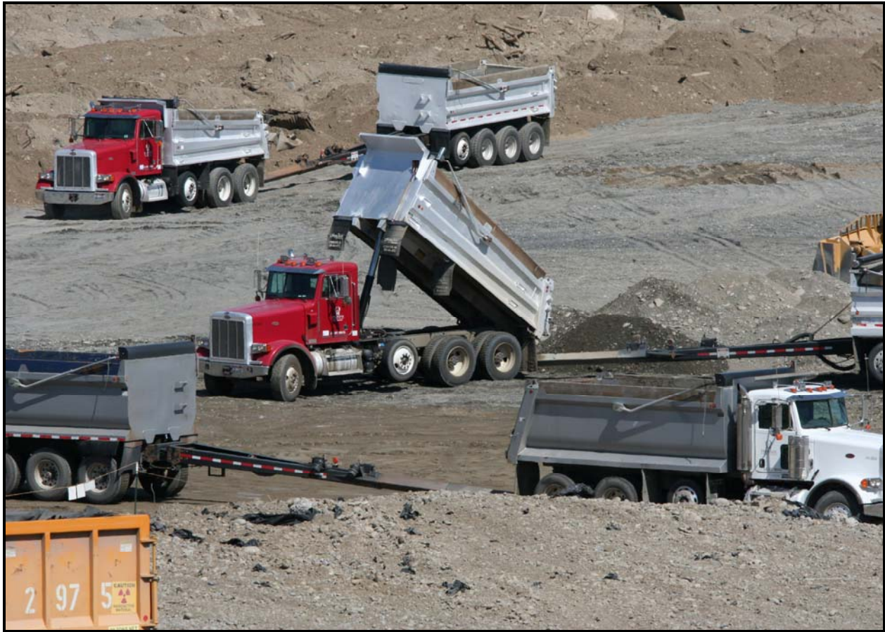
Truck-and-trailers dispose of contaminated soil in the north side of super cell 10 at the Environmental Restoration Disposal Facility. (Photo 3)
