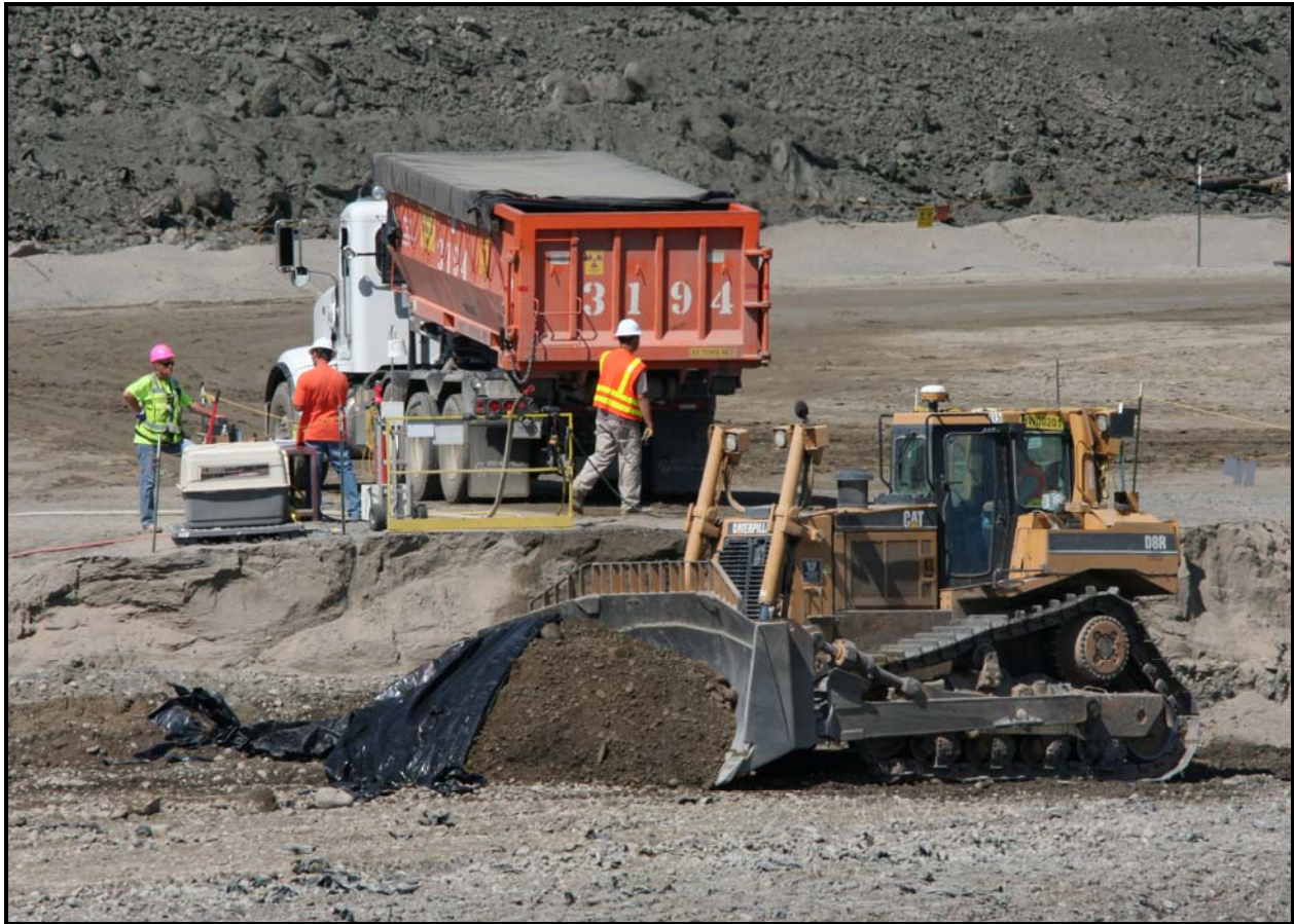
Washington Closure Hanford has disposed of more than six million tons of waste since it assumed management of the River Corridor Closure Project in August 2005. (Photo 2)
