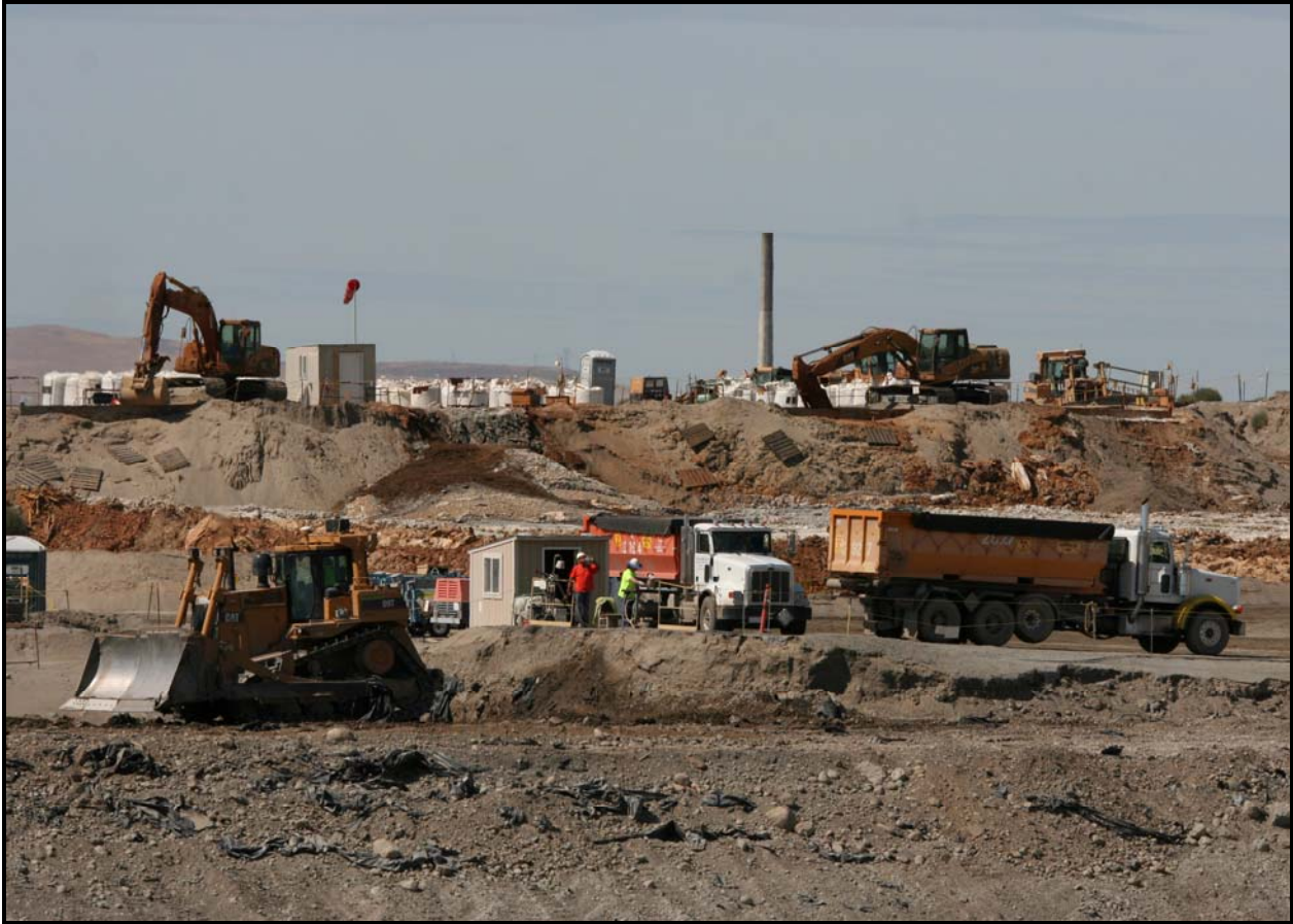
The Waste Operations team treats chrome waste, top, from 100-C-7 before disposal at the Environmental Restoration Disposal Facility. (Photo 4)
