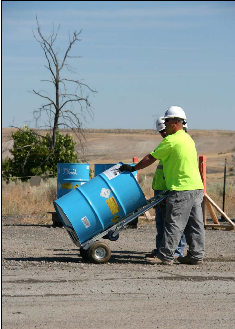
Workers at 100-F Area load a drum of sodium silicate and sodium dichromate from 100-F-26:7 for transport to a treatment facility. (Photo 5)
