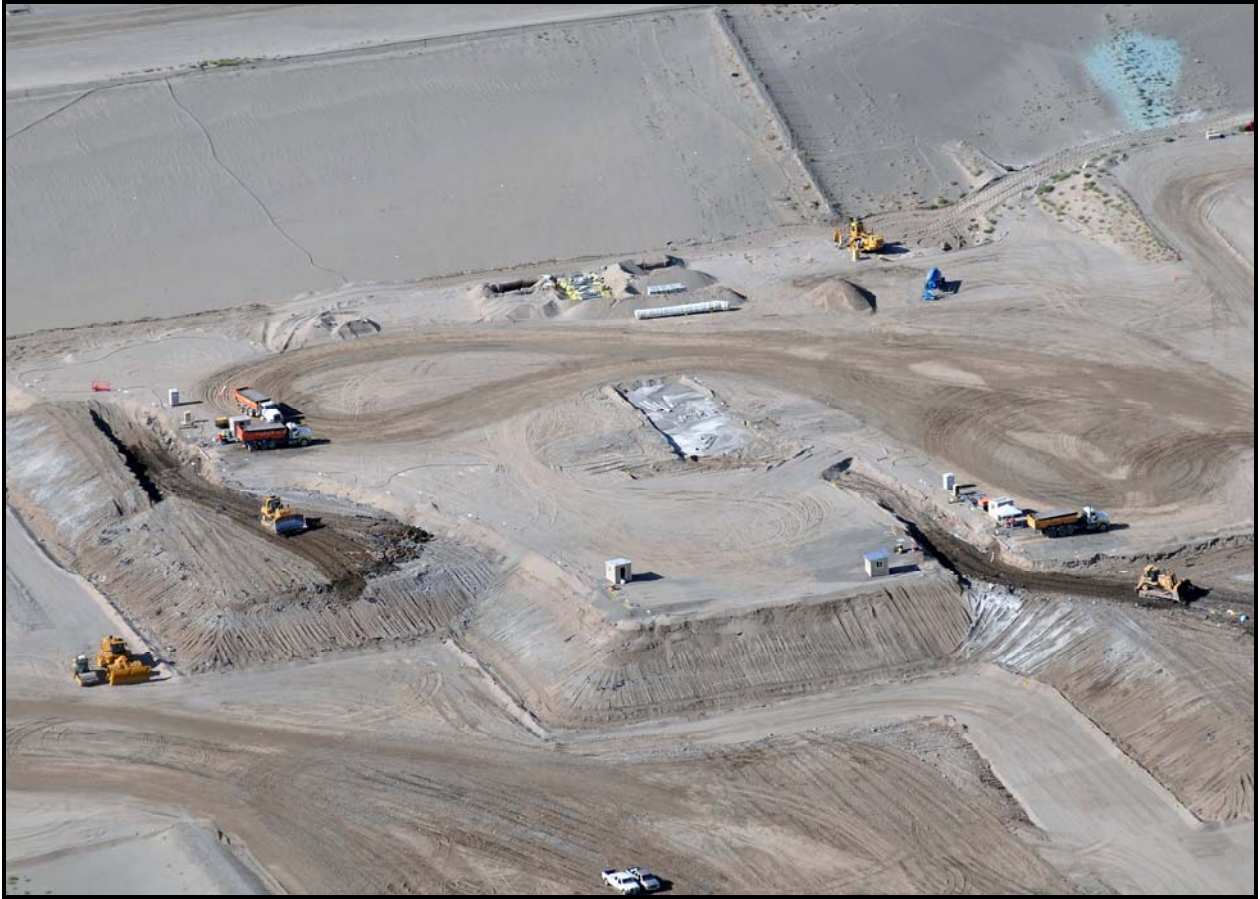
The Waste Operations team continues to fill super cell 9 at the Environmental Restoration Disposal Facility. (Photo 1)
