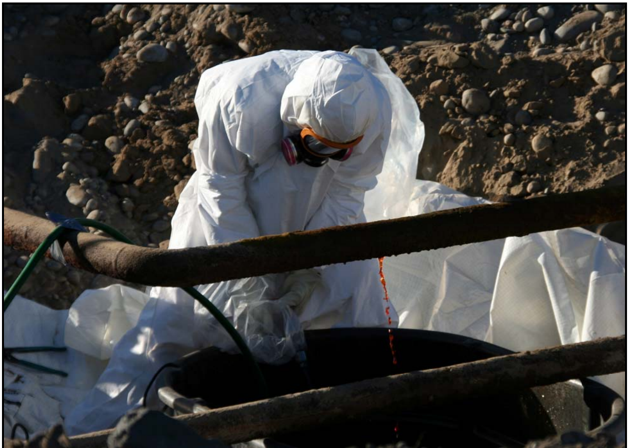
In February, Washington Closure Hanford safely removed sodium dichromate from pipelines at 100-F-26:7. (Photo 4)
