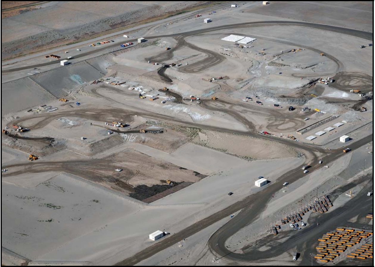
A view from the northwest corner of the Environmental Restoration Disposal Facility shows contaminated soil being spread over railroad ties (bottom left) that were recently disposed in super cell 9. (Photo 1)
