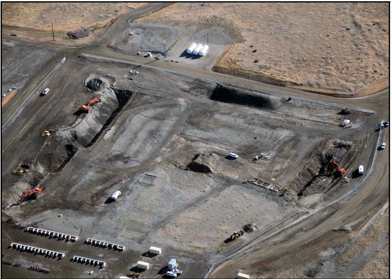
Washington Closure Hanford is excavating waste trenches on the north and south sides of the 618-10 Burial Ground. (Photo 3)
