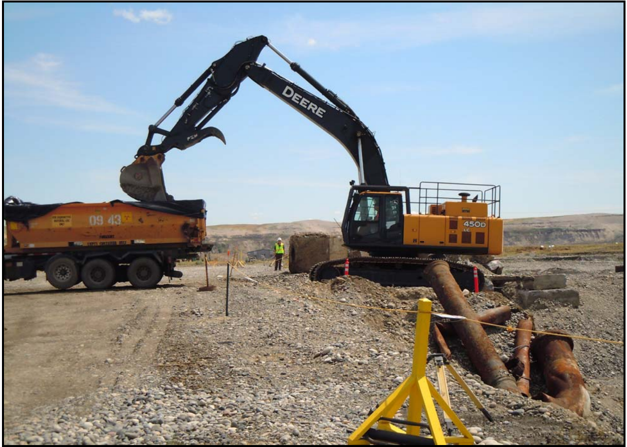
Washington Closure Hanford subcontractor loads out concrete and other debris from site 100-F-57. (Photo 7)
