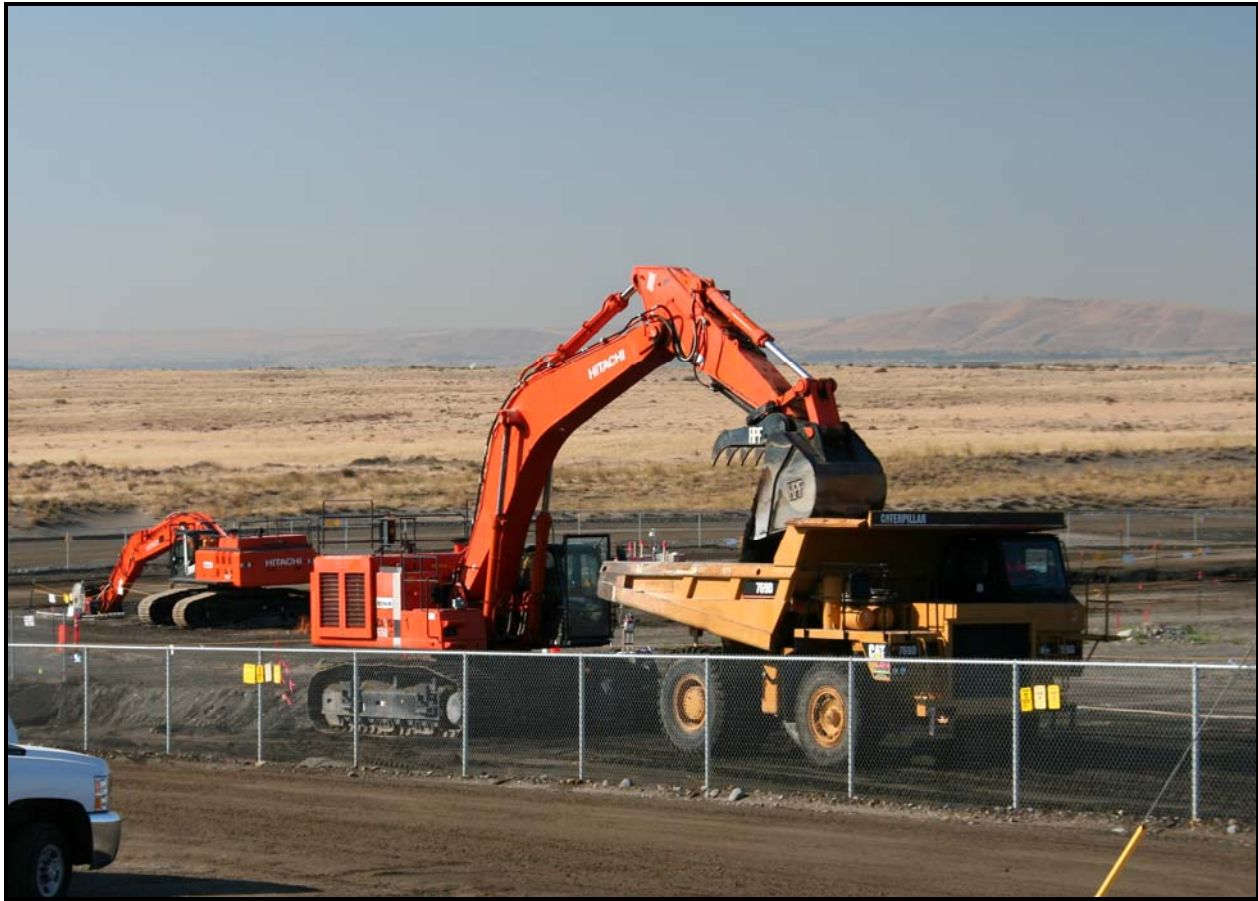
The project team enlarges a surge trench on the east side of the 618-10 Burial Ground. Surge trenches are excavated in clean soil adjacent to the burial ground. They provide a below-ground area to hold material excavated during the trench excavation process. (Photo 4)
