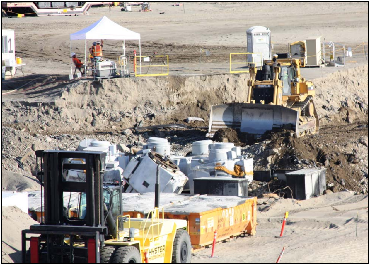
The disposal team at the Environmental Restoration Disposal Facility spreads contaminated soil over motors from the water intake structures at K reactors. (Photo 2)
