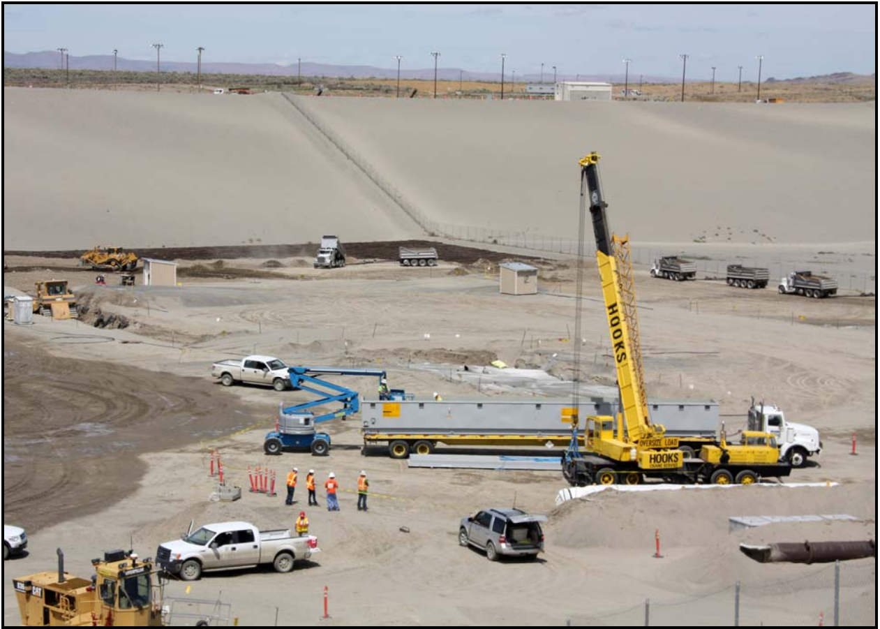
A pump from Tanks Farms is delivered to super cell 10 at the Environmental Restoration Disposal Facility. (Photo 1)
