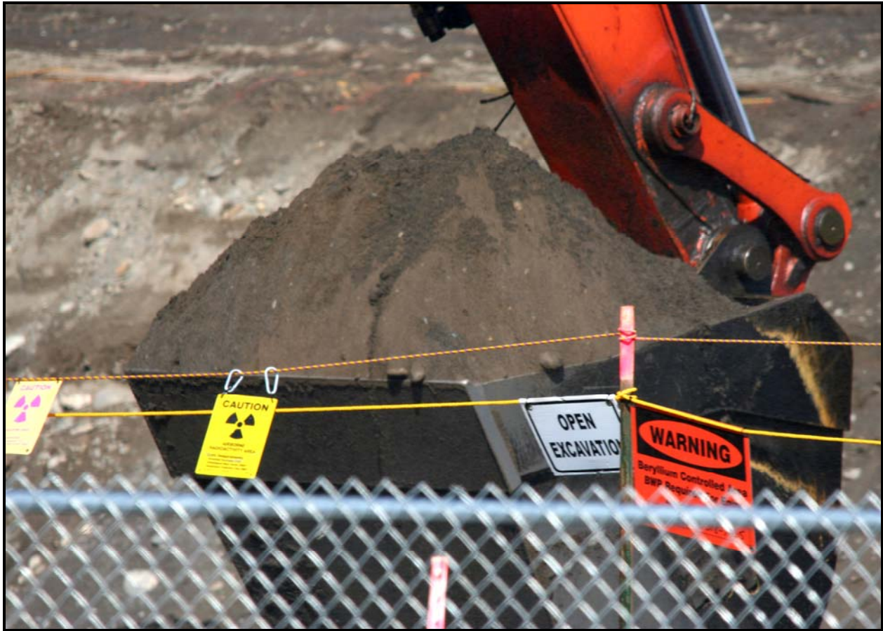
More than 35,000 bank cubic meters have been removed since excavation of the waste trenches began in April. (Photo 6)
