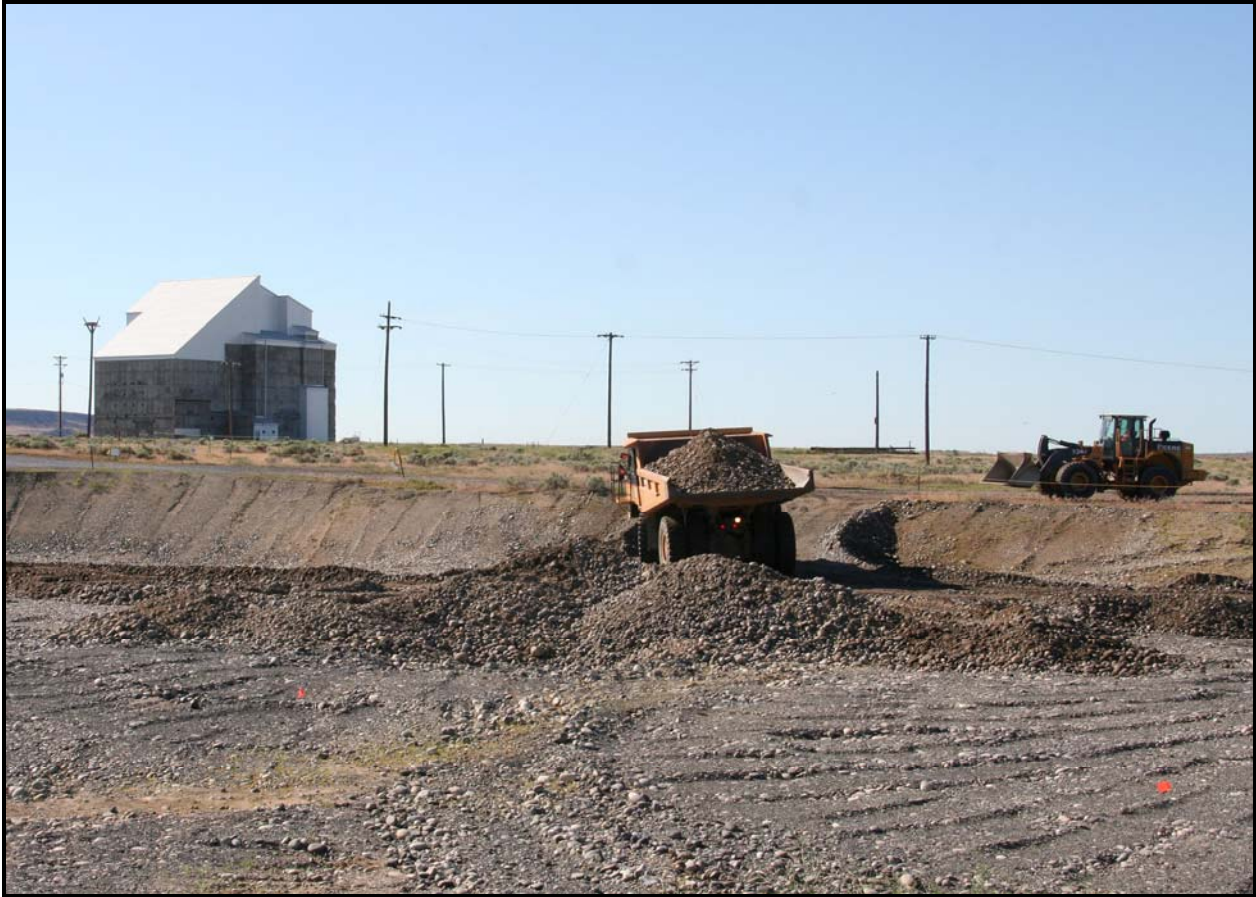
Ojeda constructs a clean path for its trucks as Washington Closure prepares 100-F-47 for further excavation. The site is a former substation. (Photo 9)
