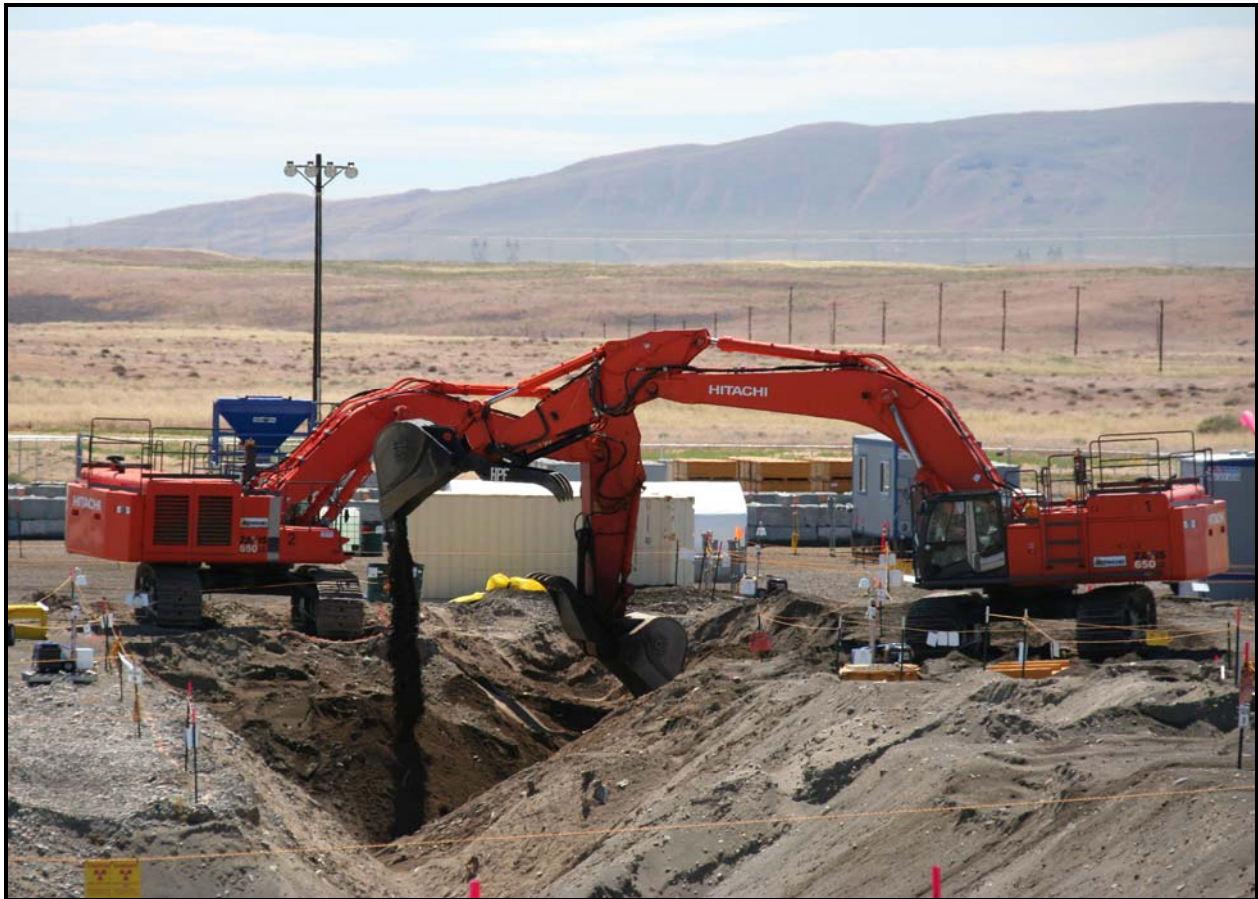
Washington Closure Hanford continues to excavate the waste trench on the north side of the 618-10 Burial Ground. (Photo 5)
