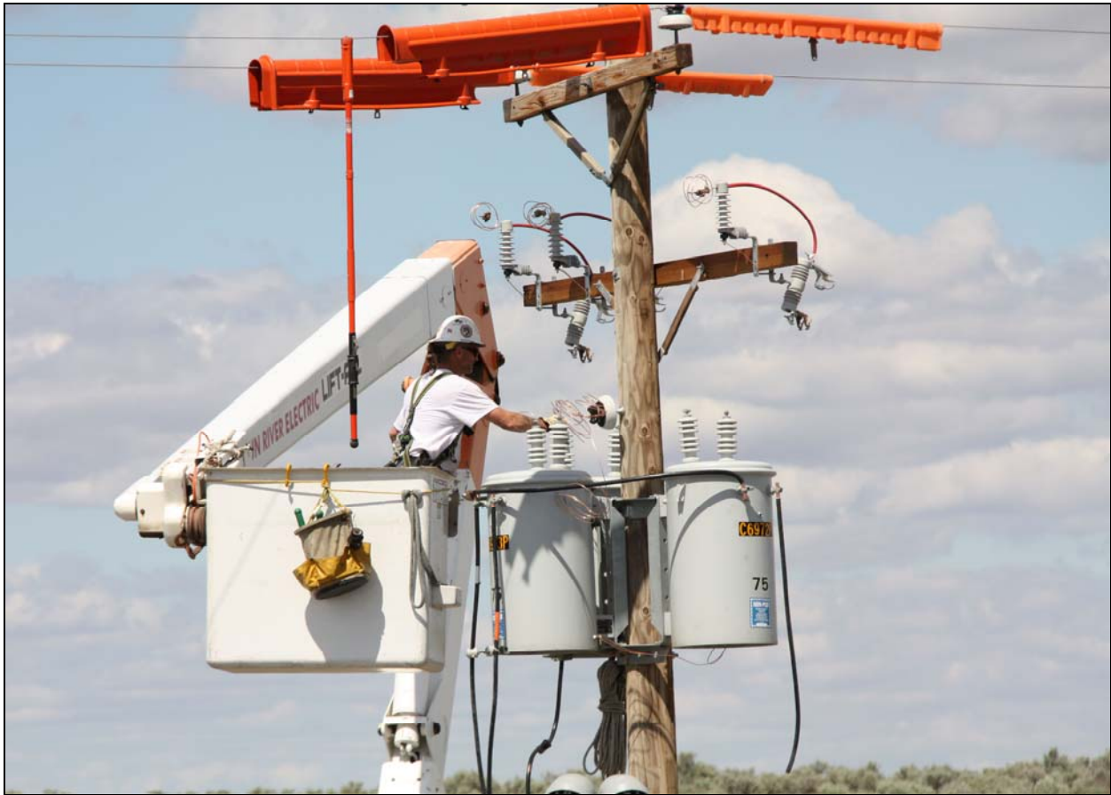
A worker with Washington Closure Hanford subcontractor ELRFowler performs electrical work for the equipment maintenance facility/operations center. (Photo 3)
