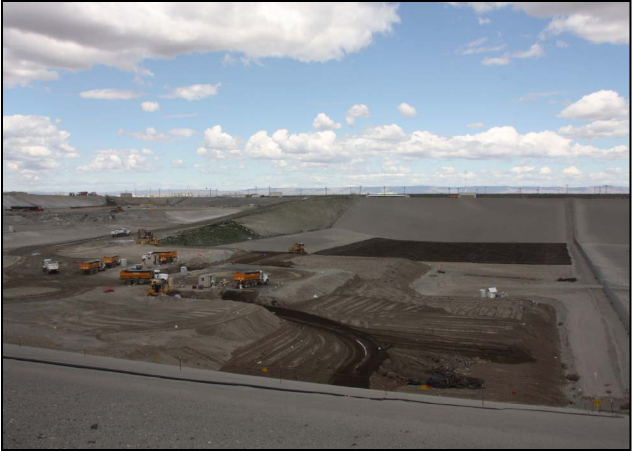
Washington Closure Hanford continues to dispose waste in super cell 9 at the Environmental Disposal Facility. The super cell was placed into service in February. (Photo 1)
