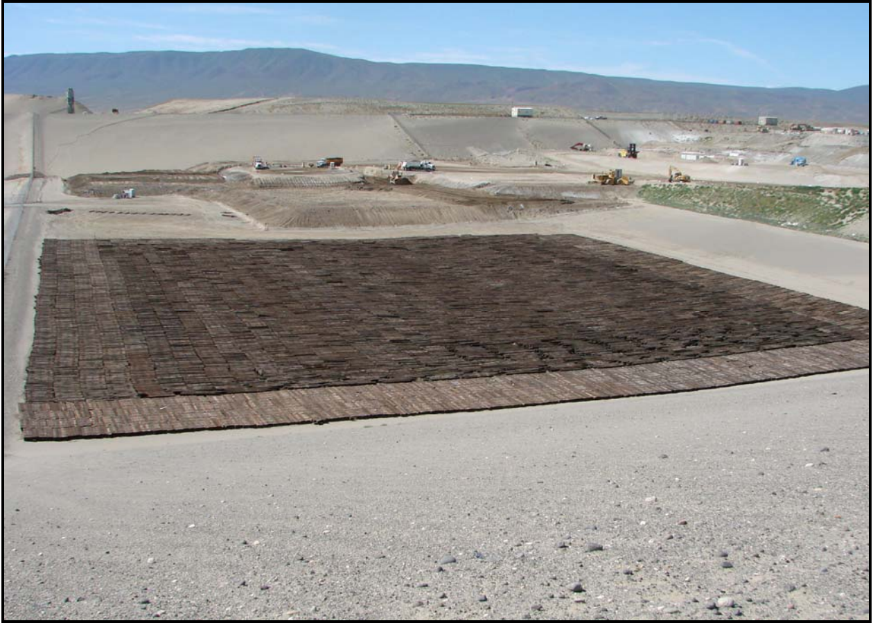
ERDF received the final shipment of 58,500 railroad ties from the Hanford Site. The railroad ties were disposed in super cell 9. (Photo 2)
