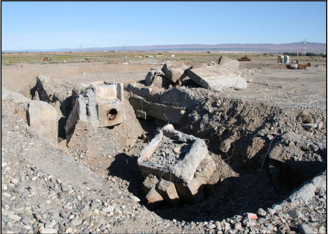
Washington Closure Hanford subcontractor Ojeda Business Ventures is demolishing concrete at 100-F-57. The site is a former water pumphouse and contains hexavalent chromium. (Photo 8)
