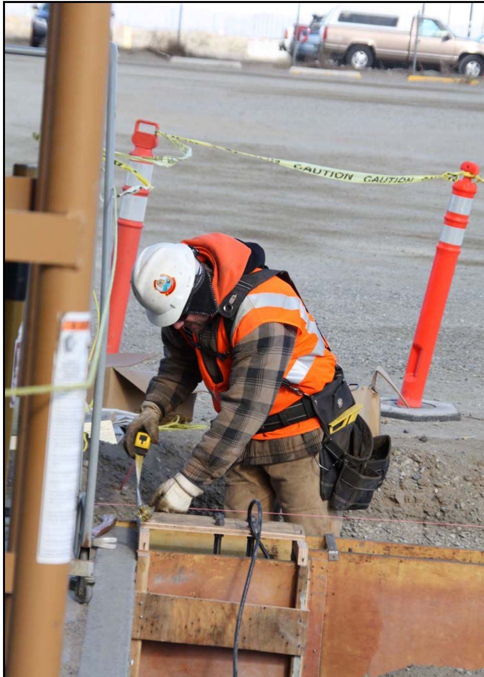
A Washington Closure Hanford subcontractor prepares to pour the concrete footers at ERDF's transportation maintenance facility. (Photo 4)
