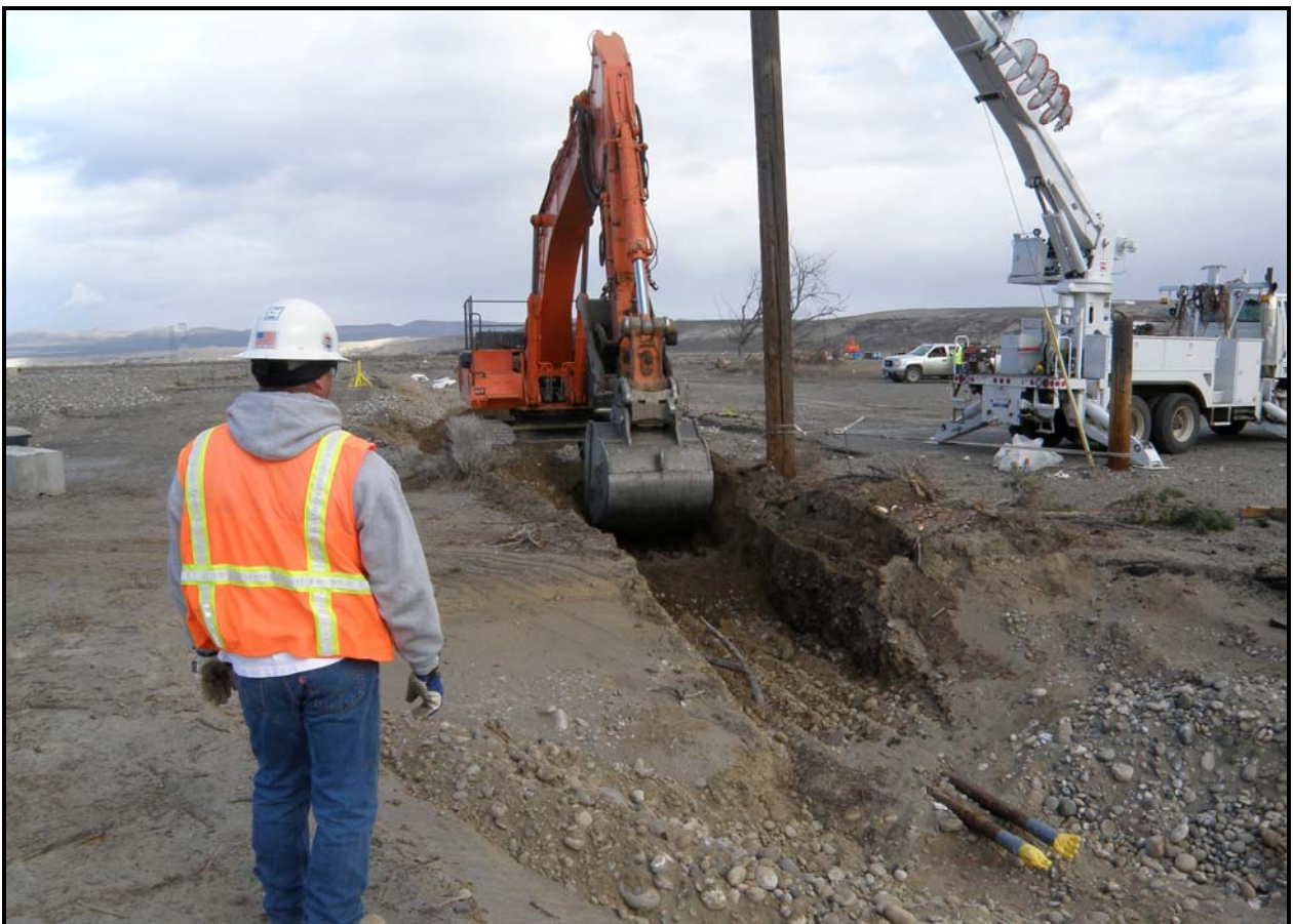
Washington Closure Hanford subcontractor Ojeda Business Ventures removes the final sections of pipe at 100-F-26:7 after Hanford subcontractor Mission Support Alliance deactivated power lines. (Photo 9)
