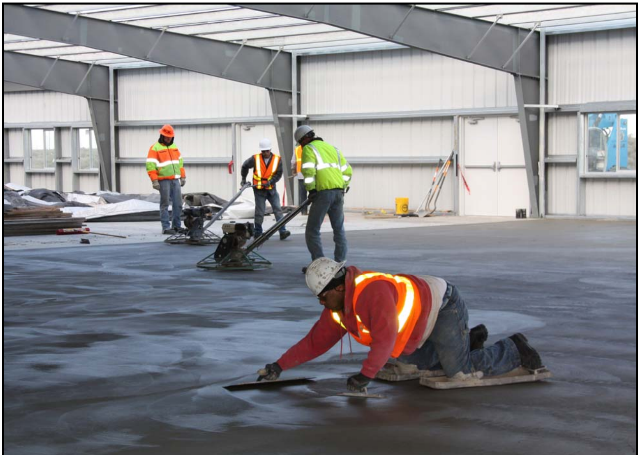
Washington Closure Hanford subcontractor ELRFowler places the second section of the concrete floor at ERDF's equipment maintenance facility/operations center. (Photo 2)
