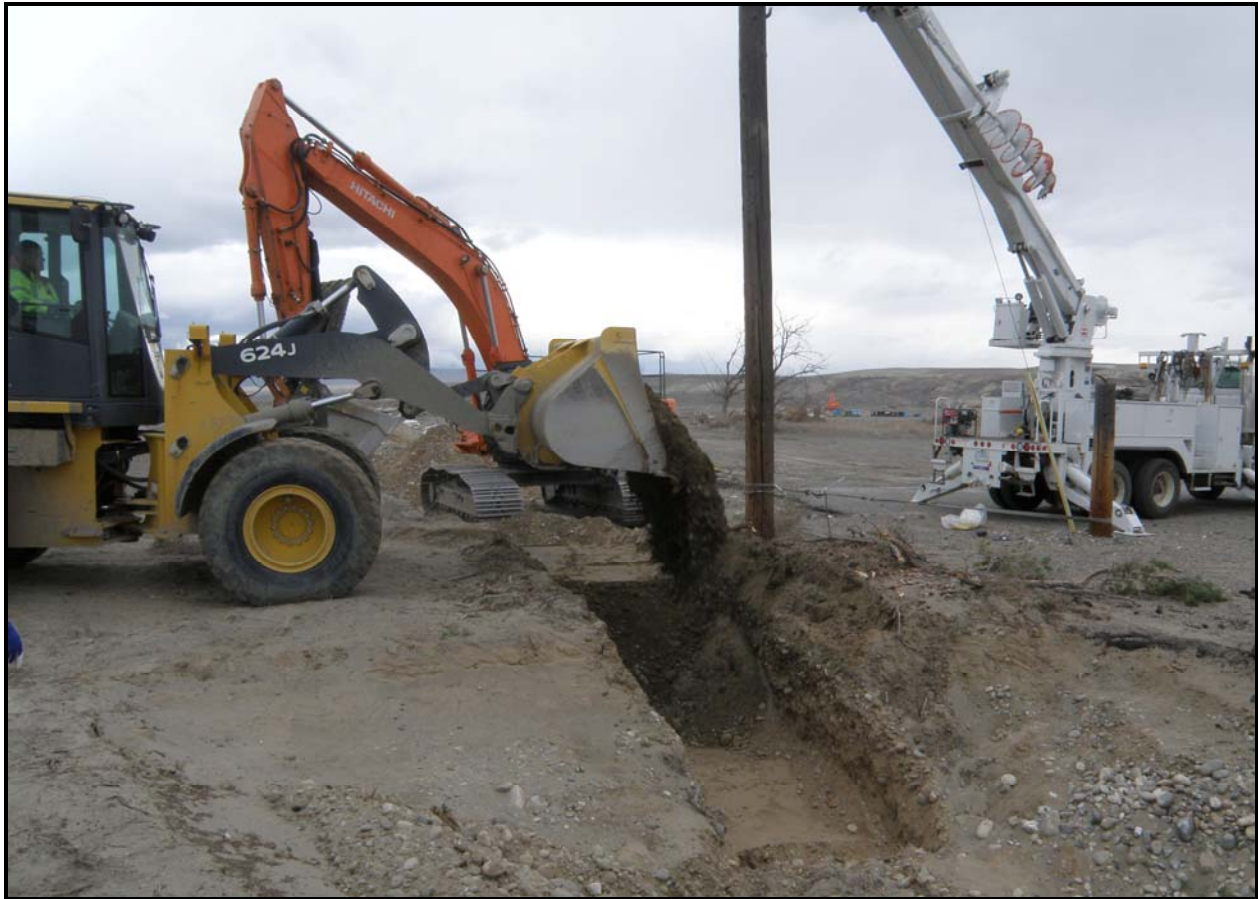
Ojeda Business Ventures backfills a trench after removing the final sections of pipe at 100-F-26:7. Last week, Washington Closure Hanford safely secured 200 gallons of sodium dichromate from pipelines at the site. (Photo 10)
