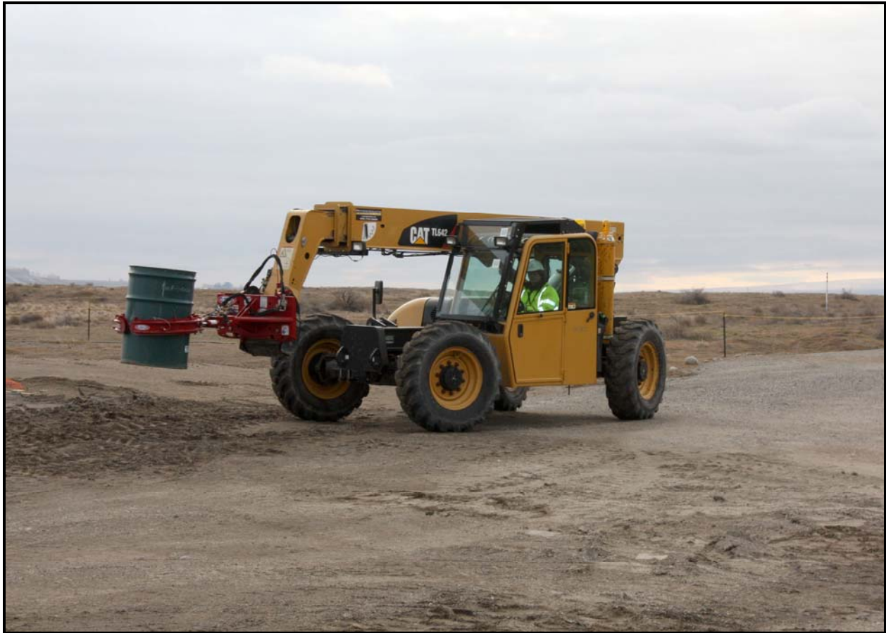
A telehandler transports a salvage container with a concreted drum during remediation mock-up exercises at the 618-10 Burial Ground. (Photo 6)
