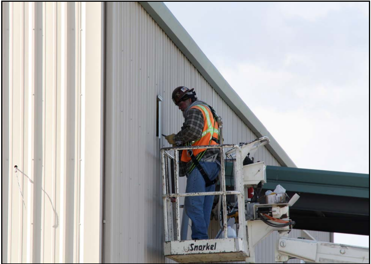
An ELRFowler employee installs siding along the north side of ERDF's container maintenance facility. (Photo 3)
