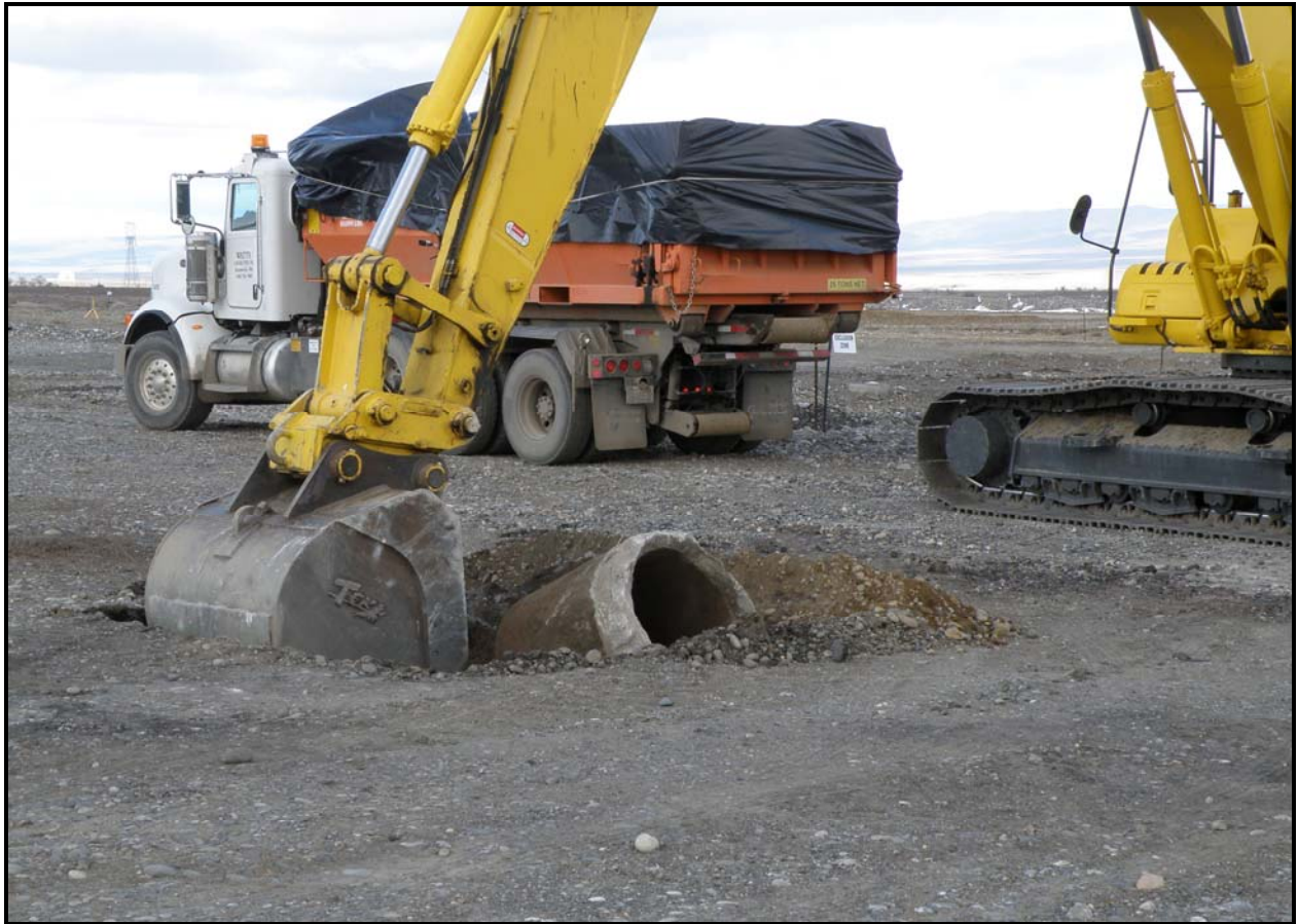
Ojeda began excavation and loadout activities at 100-F-8, a site that contains an underground injection control well. (Photo 11)
