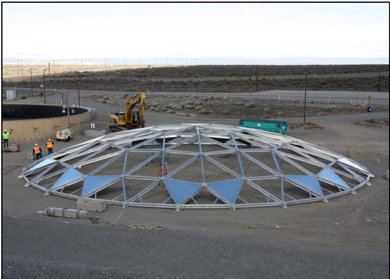
Washington Closure Hanford subcontractor TradeWind Services installs the decking panels on the dome cover for one of ERDF’s new leachate storage tanks. (Photo 1)
