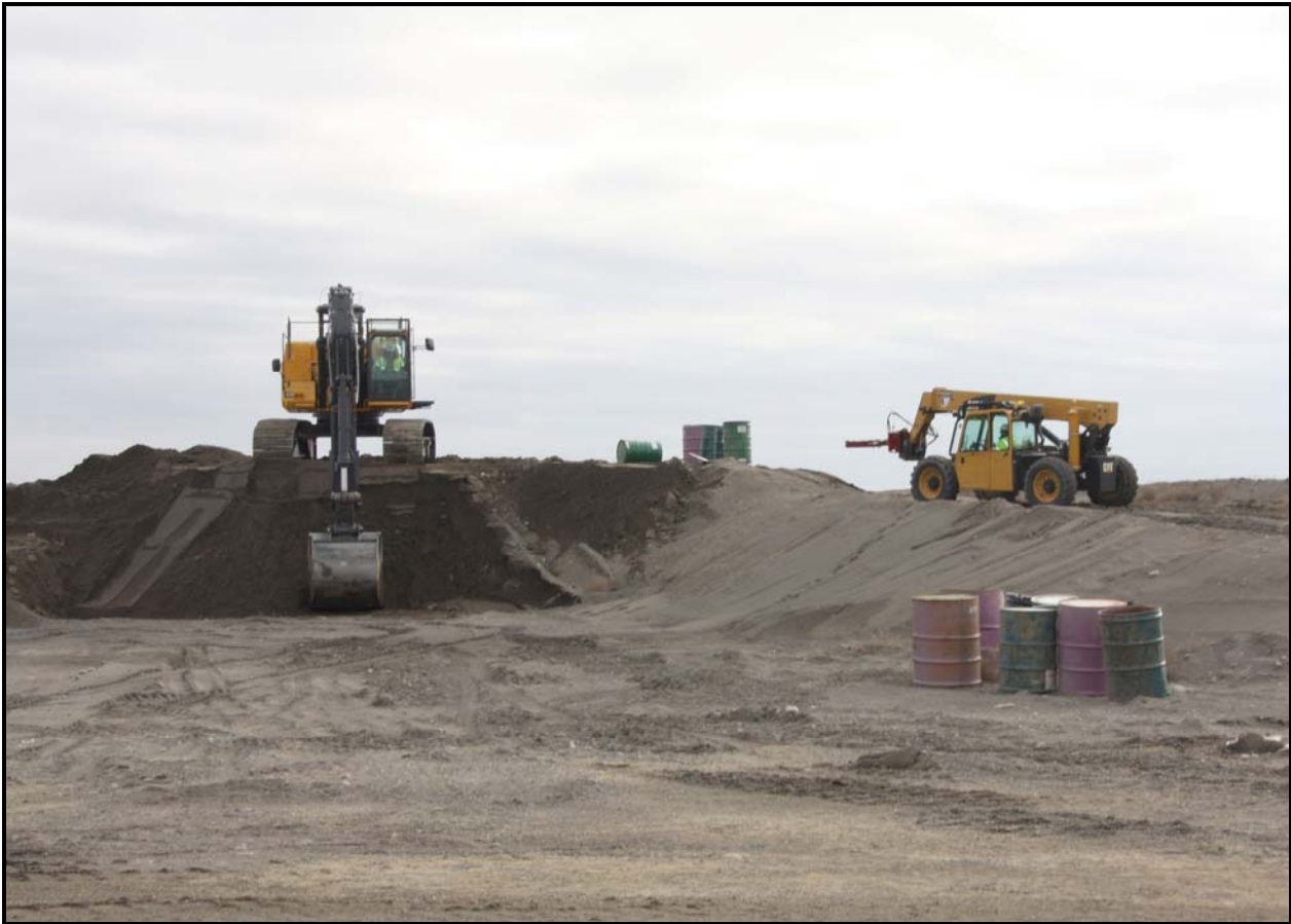
Remediation mock-up exercises continue at the 618-10 Burial Ground. Full-scale remediation is scheduled to begin in March. (Photo 5)
