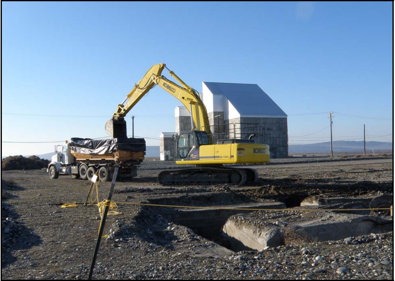
Washington Closure Hanford subcontractor Ojeda Business Ventures loads out old pipe cradle rubble from 100-F-57. (Photo 11)
