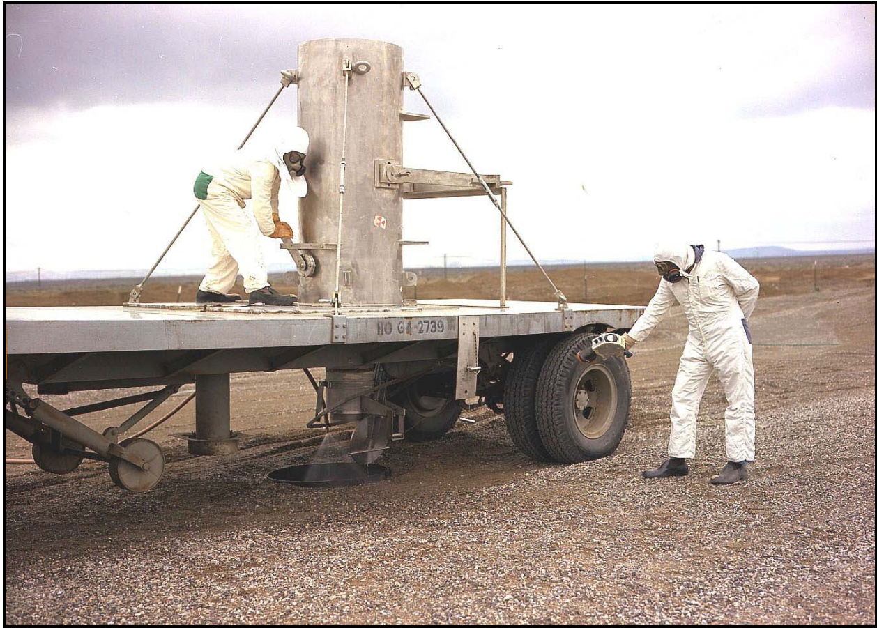
This photo from April 1967 shows delivery of waste to the 618-11 Burial Ground. One worker opens the cask that opens the cask cover allowing the waste to drop into a caisson. The other worker checks radiation levels. A water spray keeps dust particles from dispersing into the environment. (Photo 9)
