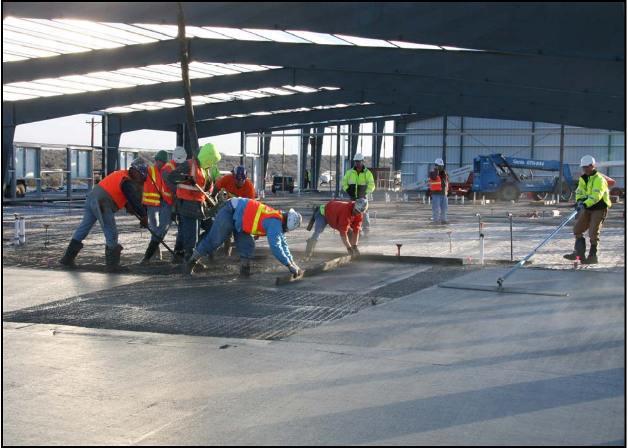
Washington Closure Hanford subcontractor ELRFowler began pouring concrete at ERDF's equipment maintenance facility/operations center. The project team also began installing the siding on the east side of the building. (Photo 1)
