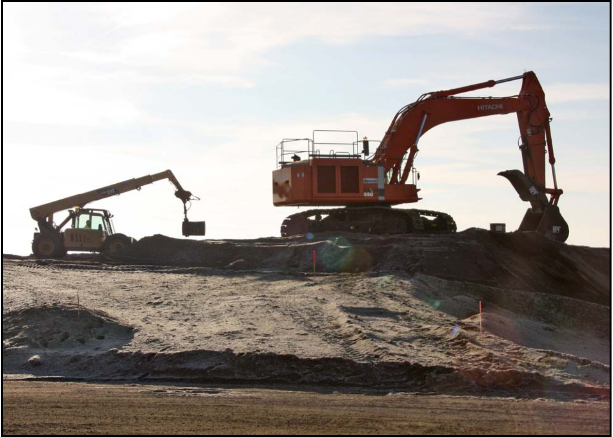
An excavator and telehandler perform mock-up exercises at the 618-10 Burial Ground. (Photo 6)
