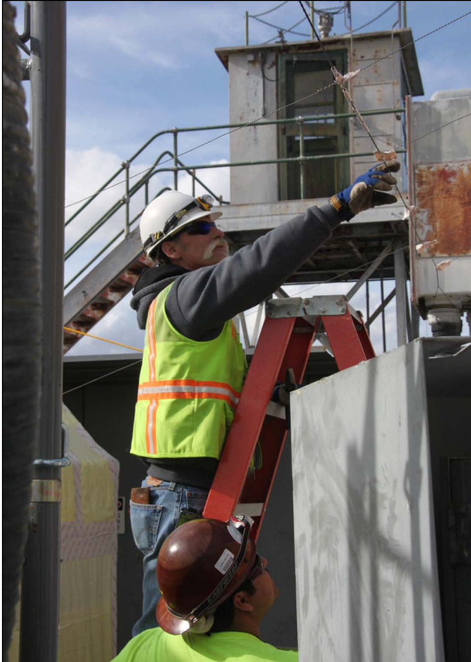
Workers check a wire on a containment structure for the 181-KE River Pump House Structure that CHPRC is preparing for demolition.
