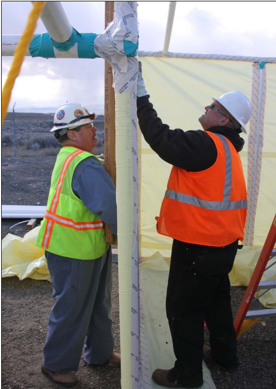
An asbestos containment tent is constructed at the site of the 181-KE River Pumphouse structure.
