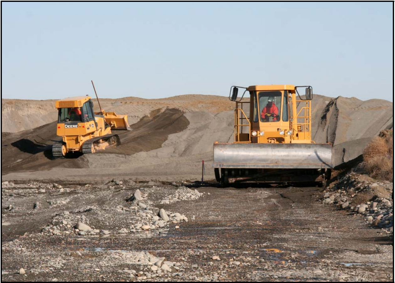
Road work continues at the 618-10 Burial Ground. Crews are constructing a road around the site, a firebreak, and a drum processing area.
