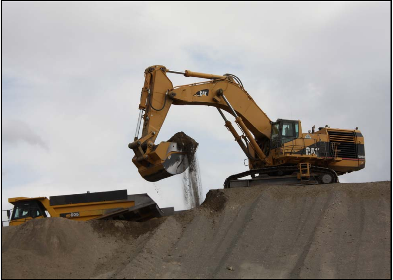
Crews have been removing about 30,000 cubic yards of soil per day on a regular basis at the Environmental Restoration Disposal Facility.
