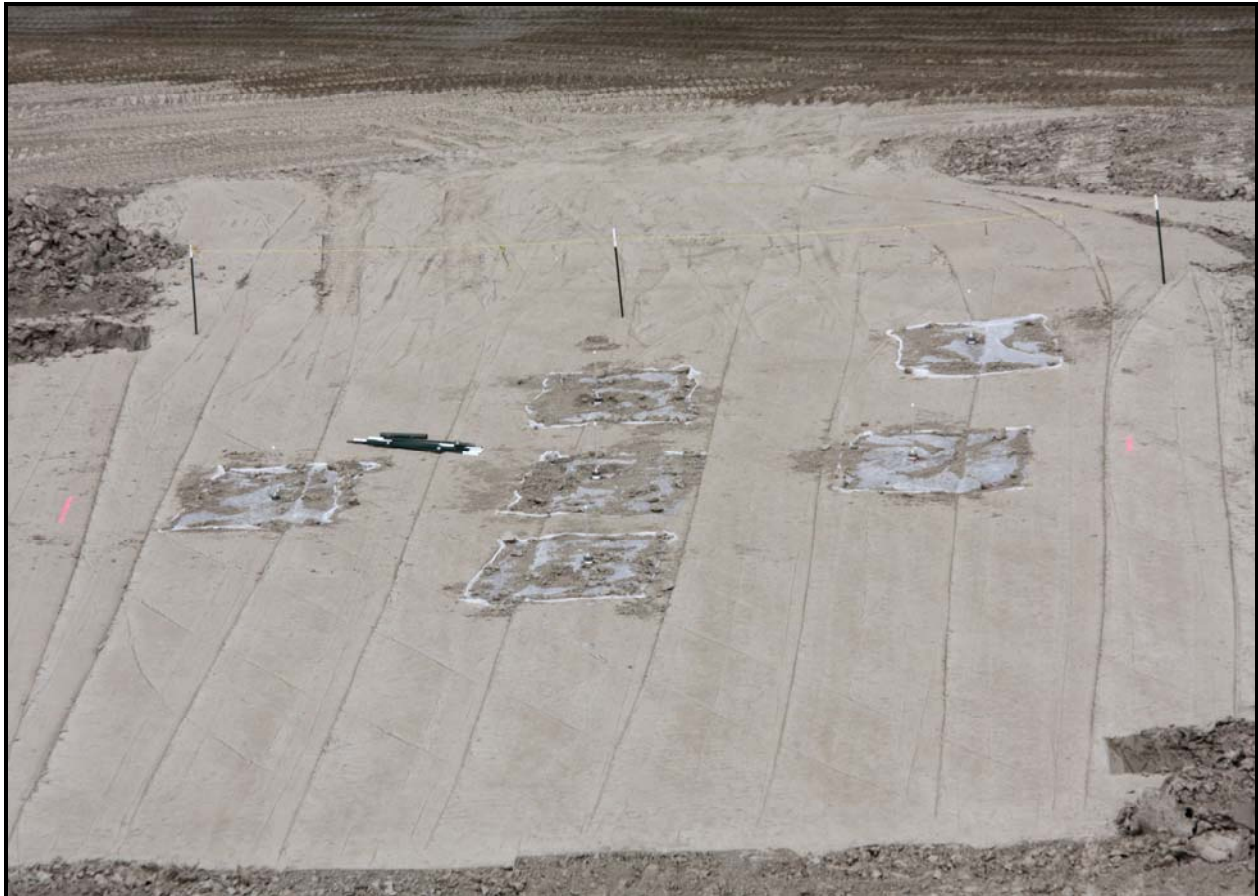
Plastic measuring tubes were inserted into six boreholes drilled into the admix test pad at the Environmental Restoration Disposal Facility.
