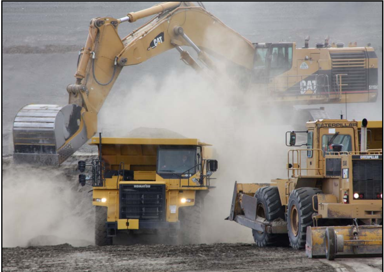
TradeWind Services subcontractor DelHur Industries continues excavation of super cell 10 at the Environmental Restoration Disposal Facility.
