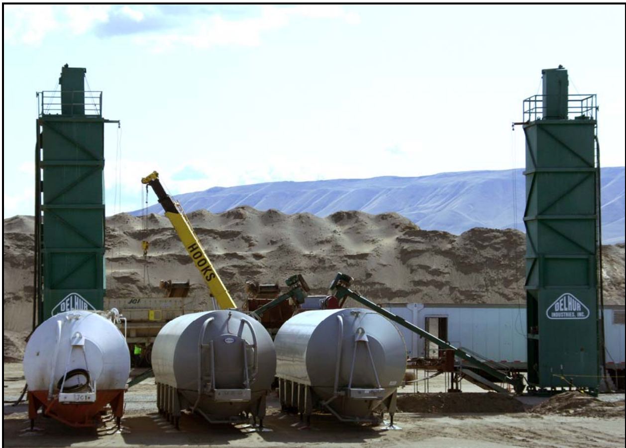
DelHur Industries continues to set up a pug mill, which will be used to create the admix layer of the liner system for super cells 9 and 10 at the Environmental Restoration Disposal Facility.
