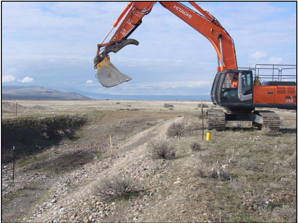
Site 600-343 was one of three sites recently remediated at IU 2&6 Segment 1. Washington Closure Hanford is in the process of closing out the remediated sites.
