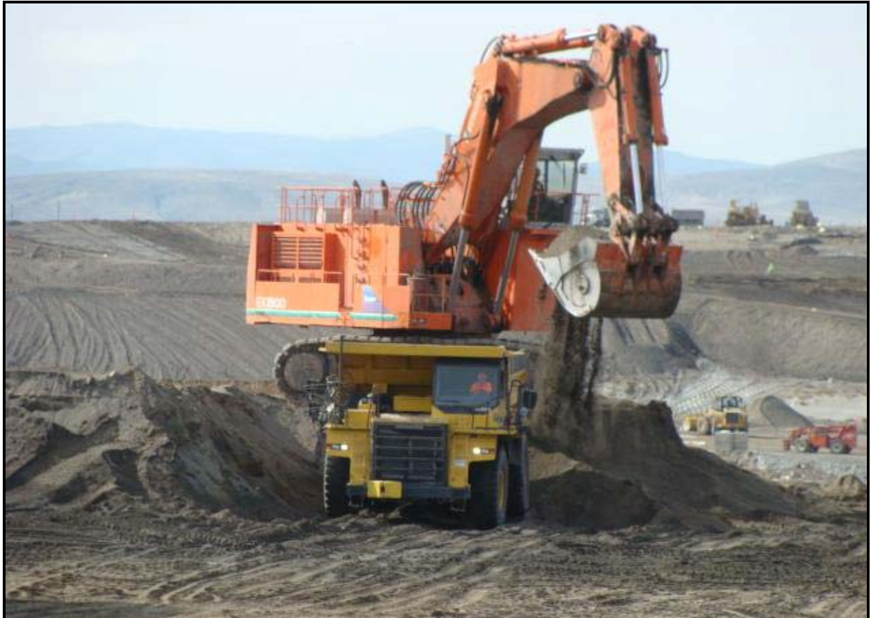
An excavator with a 13 cubic yard bucket was put into service at the Environmental Restoration Disposal Facility.
