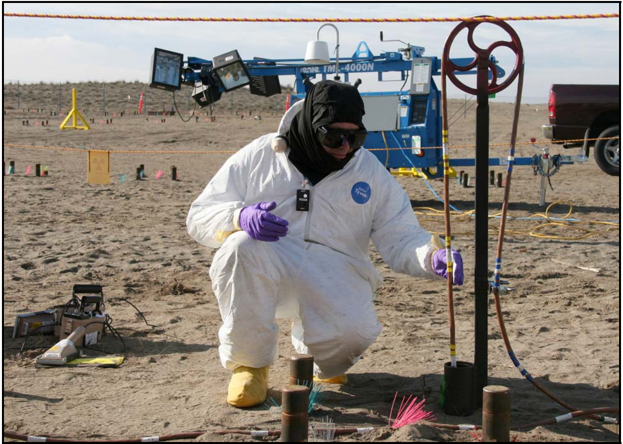
Nonintrusive radiological characterization activities continue in the vertical pipe unit area at the 618-10 Burial Ground.
