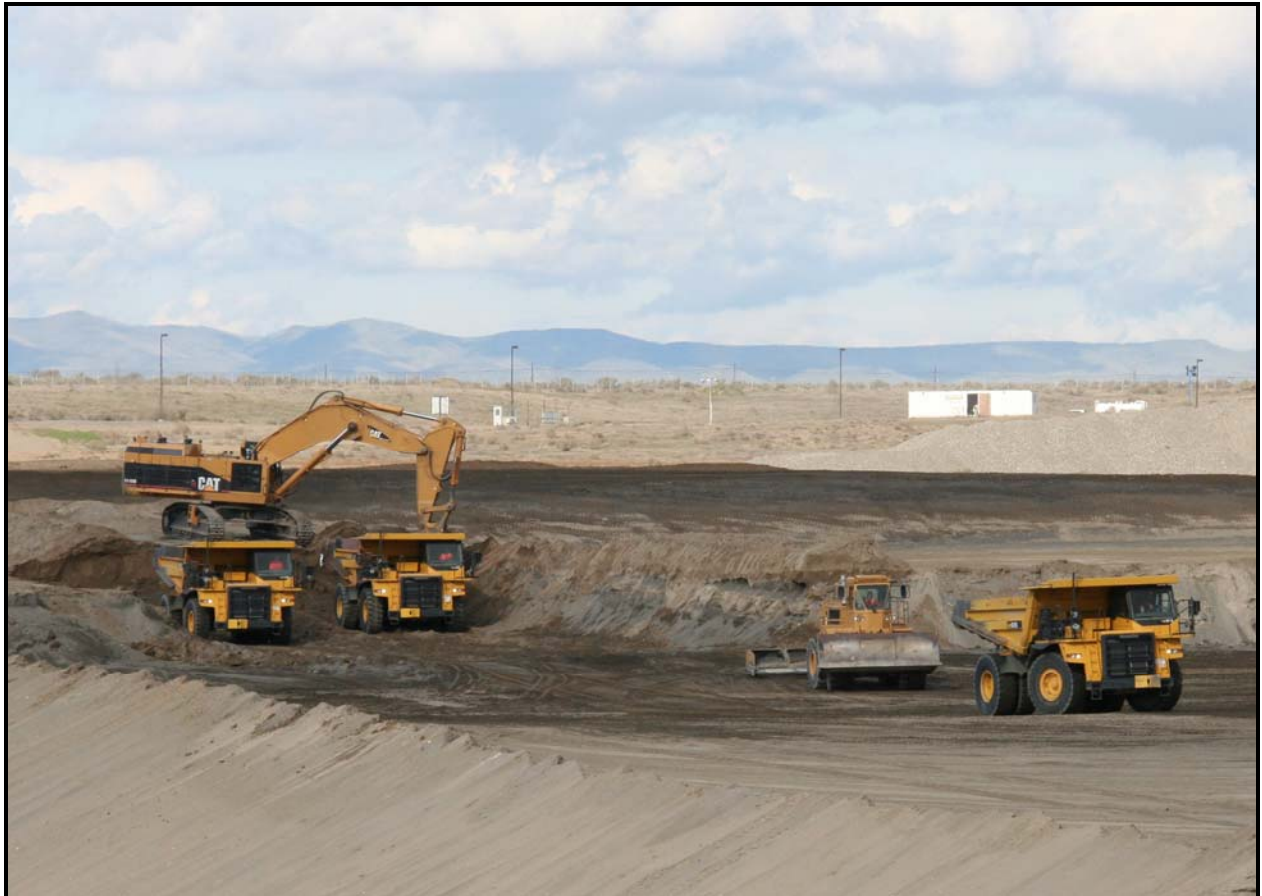
TradeWind Services/DelHur Industries personnel continue to excavate super cell 10 at the Environmental Restoration Disposal Facility.
