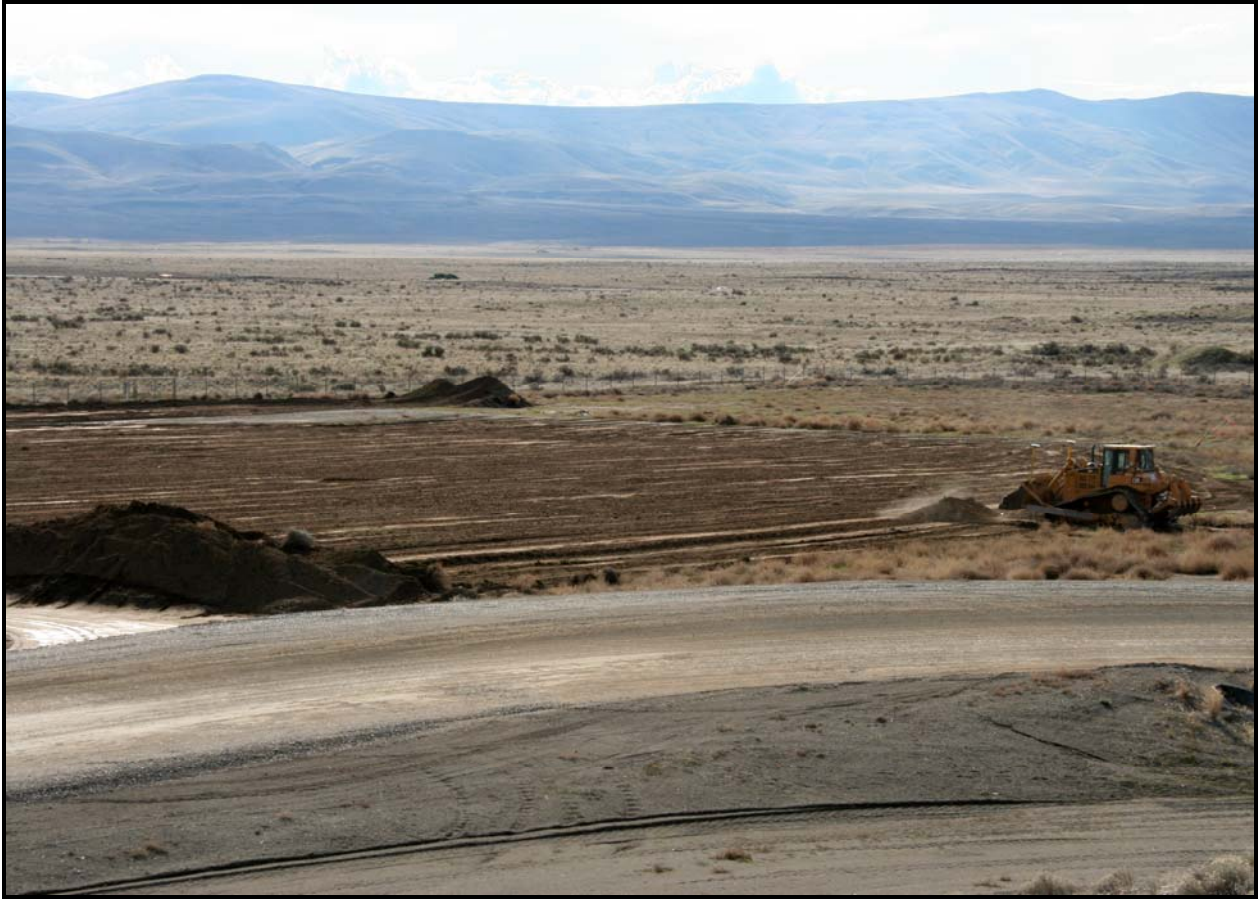
TradeWind Services/DelHur Industries personnel began work on the new transportation yard at the Environmental Restoration Disposal Facility.
