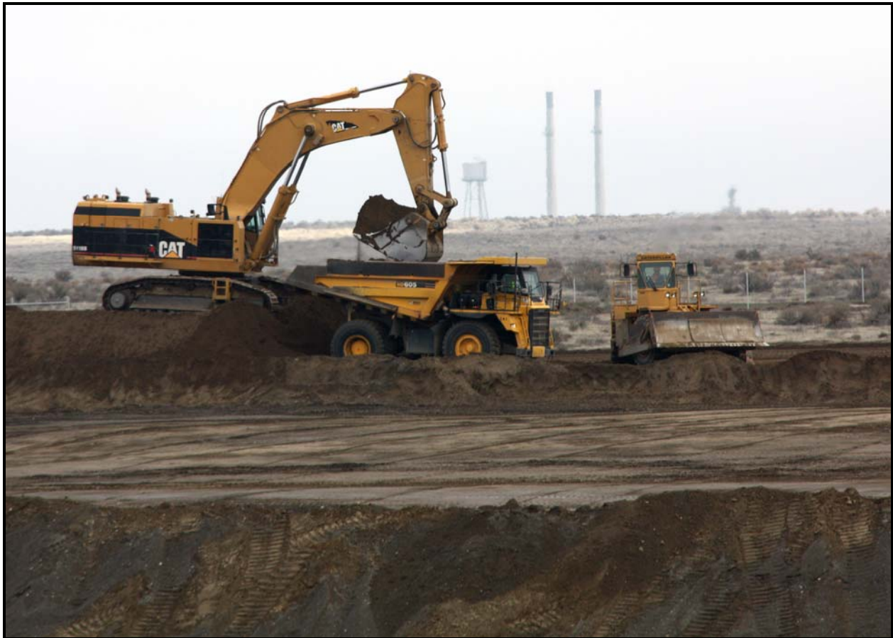
Trade Wind Services/DelHur Industries personnel are in the beginning stages of super cell 10 excavation at the Environmental Restoration Disposal Facility.
