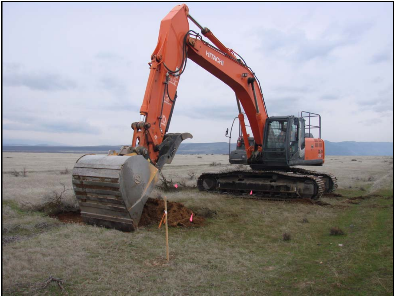
Remediation work was conducted at site 600-345, a stained area that contained oil filters.
