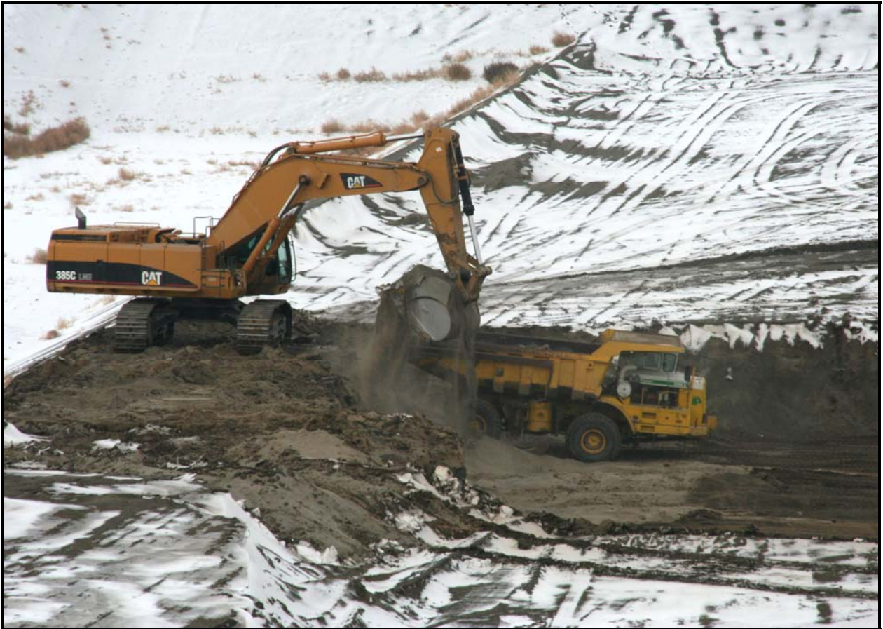
Delhur Industries personnel work through adverse weather conditions as they excavate super cell 9 at the Environmental Restoration Disposal Facility.
