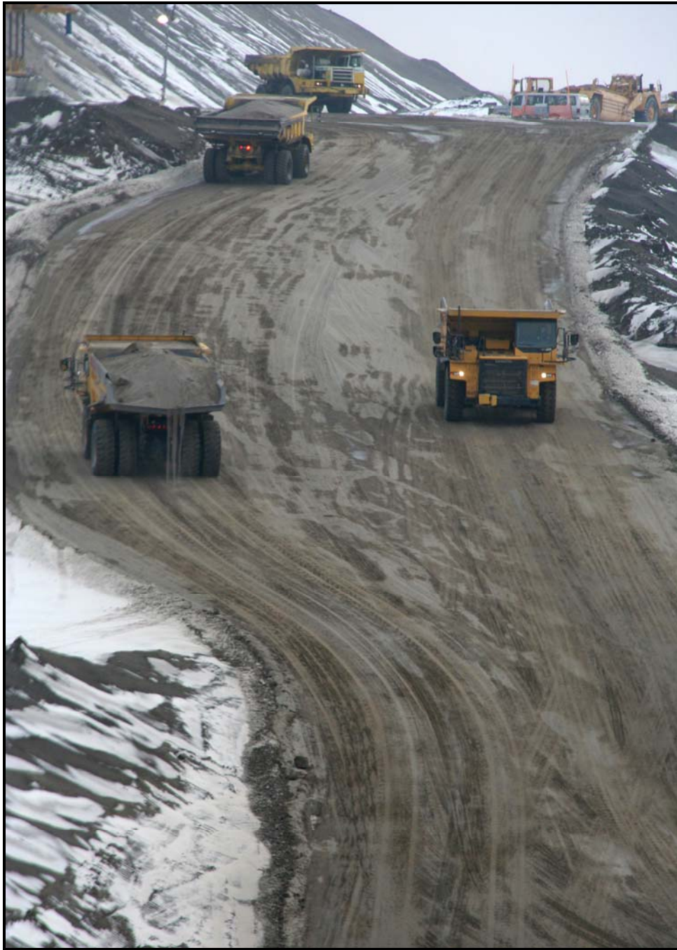
Delhur Industries personnel are excavating 1.6 million cubic yards of dirt from super cell 9 at the Environmental Restoration Disposal Facility.
