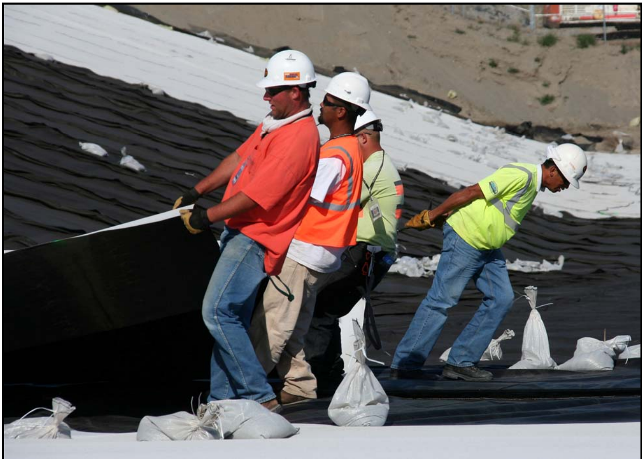
TradeWind Services/DelHur Industries personnel continue to install high-density polyethylene liner in super cell 9 at the Environmental Restoration Disposal Facility.
