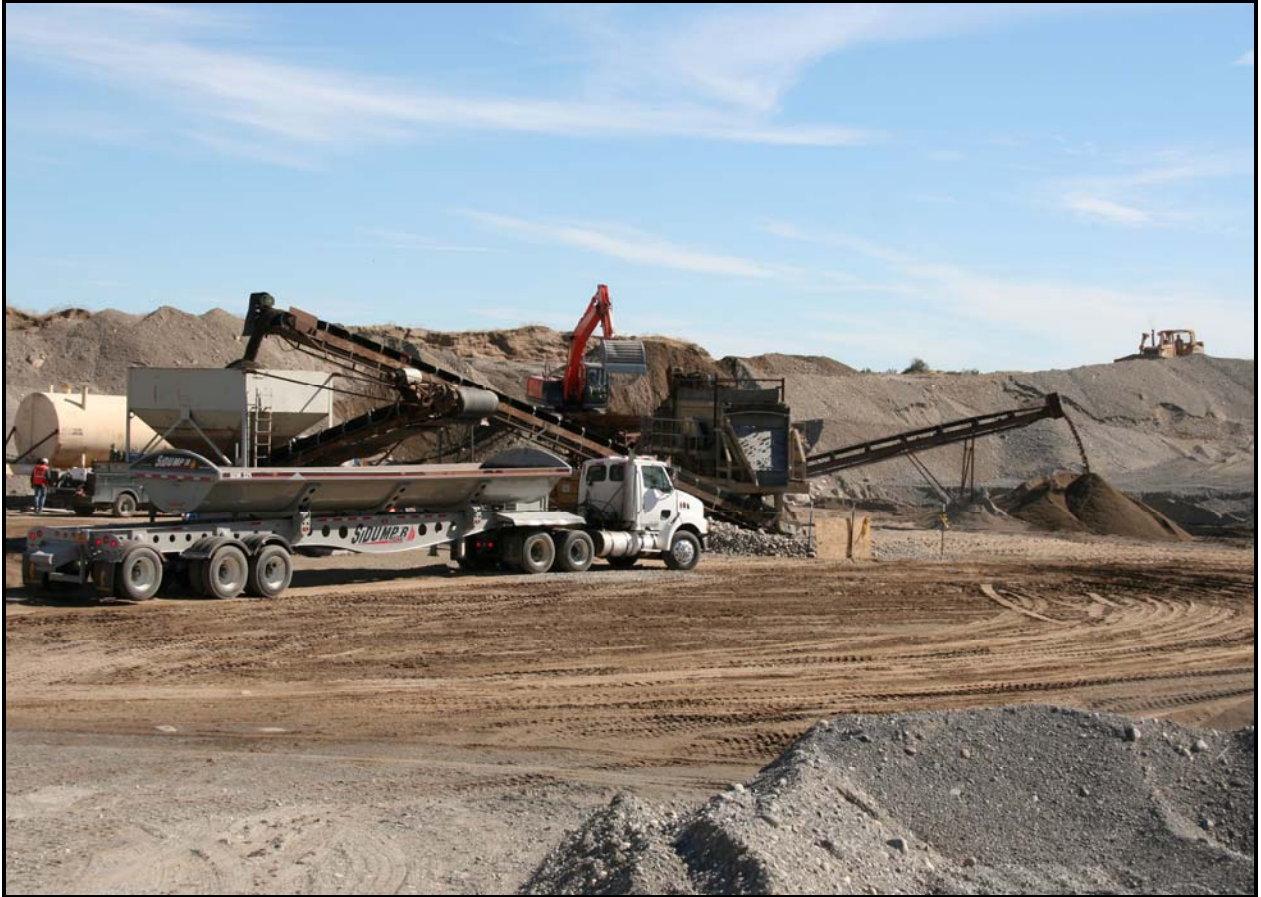
The screening plant is up and running at the Environmental Restoration Disposal Facility. The plant is used to prepare gravel to be used in the liner and leachate collection systems in super cells 9 and 10.
