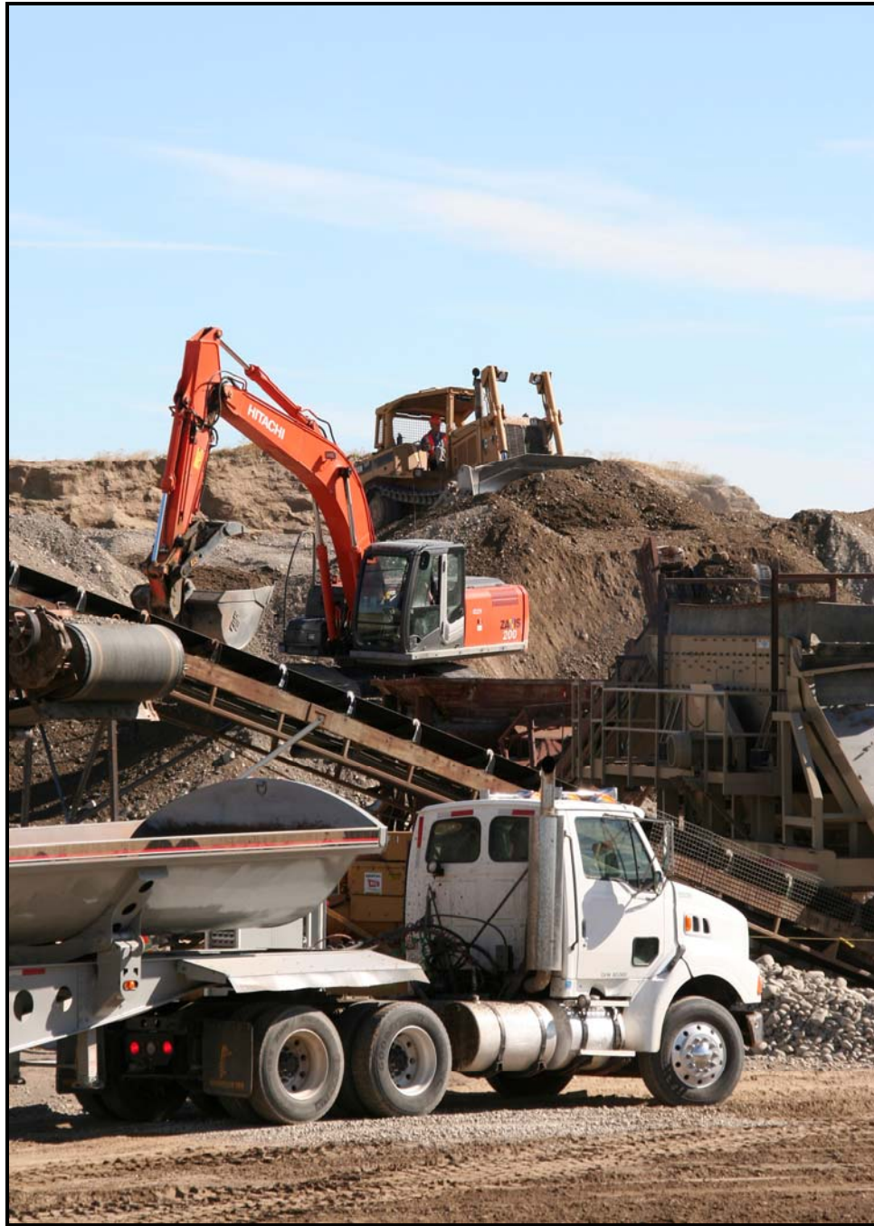
The liner and leachate collection systems for super cells 9 and 10 at the Environmental Restoration Disposal Facility will require 40,000 cubic yards of gravel.
