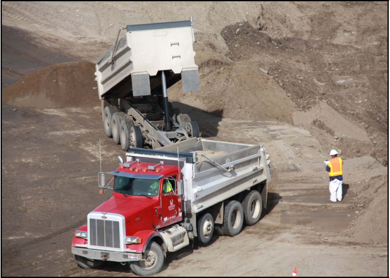
Washington Closure Hanford subcontractor George A. Grant began installing lighting at the Environmental Restoration Disposal Facility's transportation yard. The transportation yard is used for truck-and-trailer combinations (above) and other equipment.
