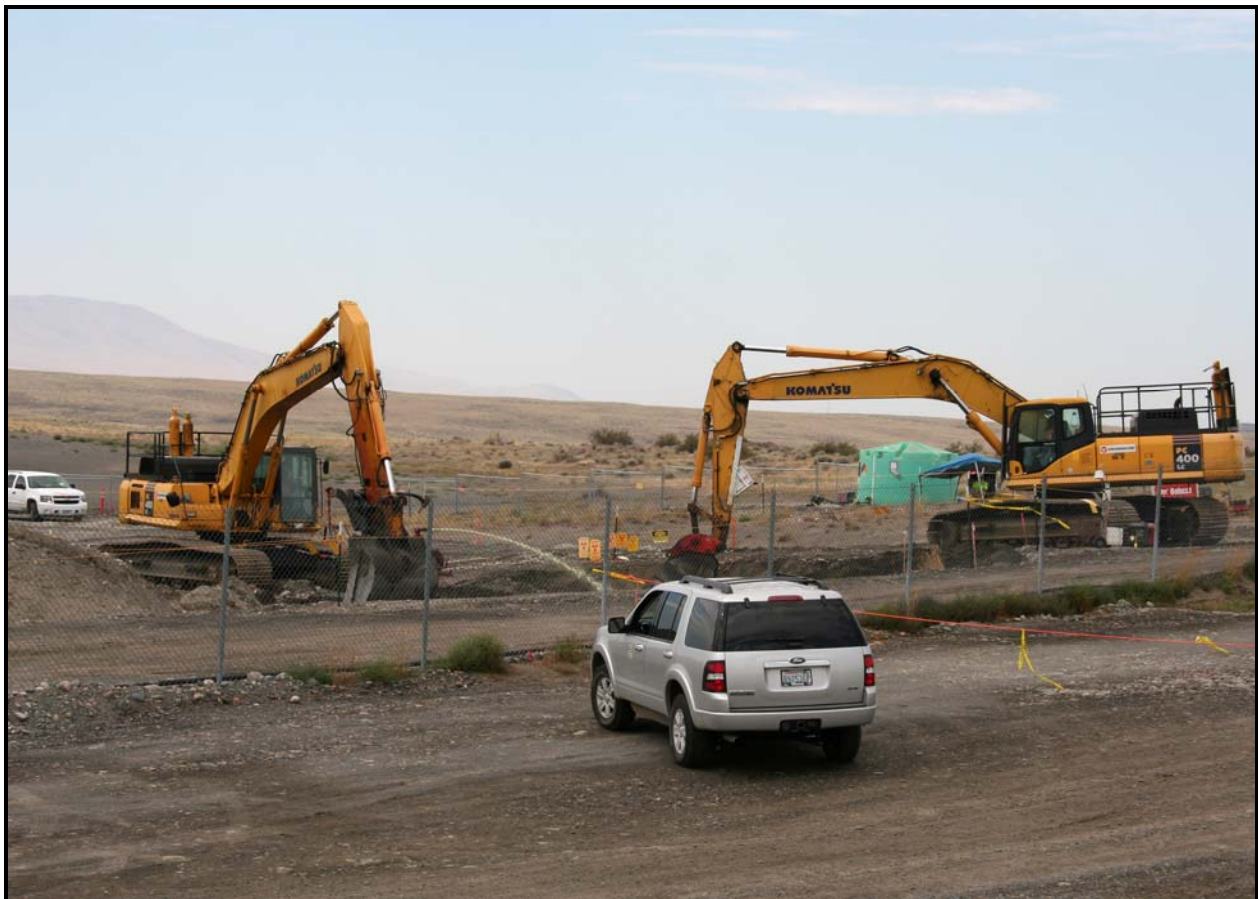
Trenching activities in support of intrusive characterization continued at the 618-10 Burial Ground.
