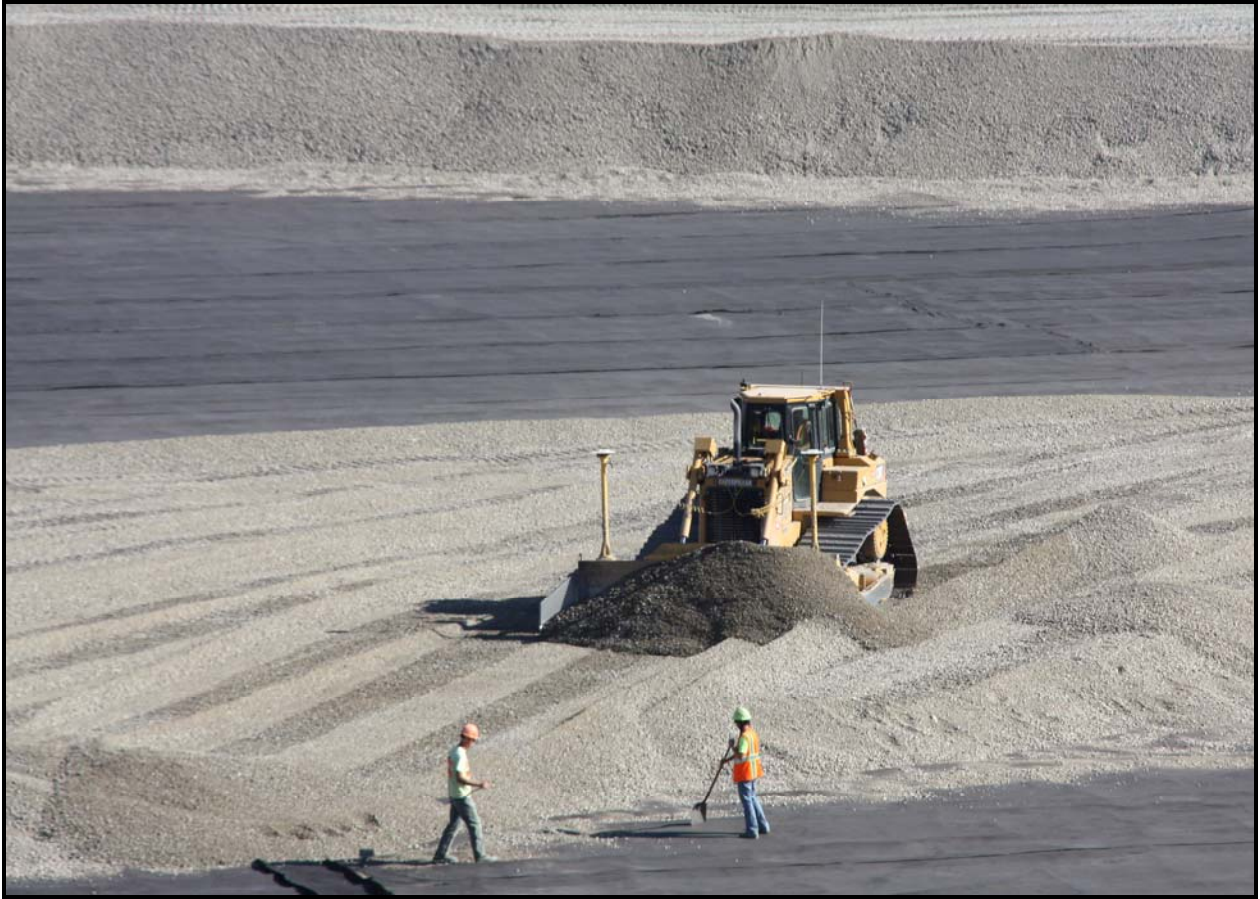
Workers spread gravel in super cell 9 at the Environmental Restoration Disposal Facility. The gravel is used for the gravel drainage layer of the liner system.
