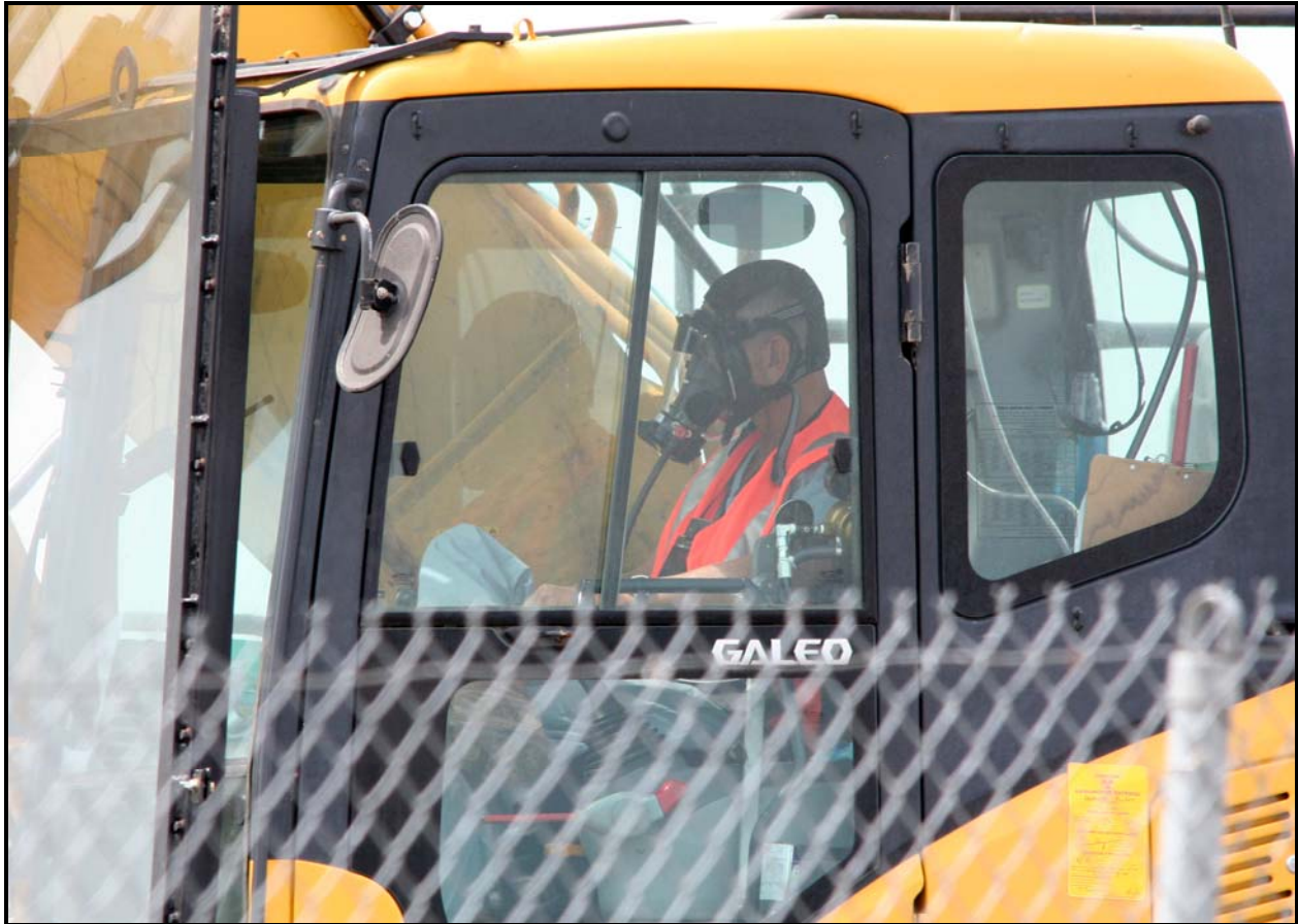
An employee of Washington Closure Hanford subcontractor Envirocon operates a track-hoe during trenching activities at the 618-10 Burial Ground.
