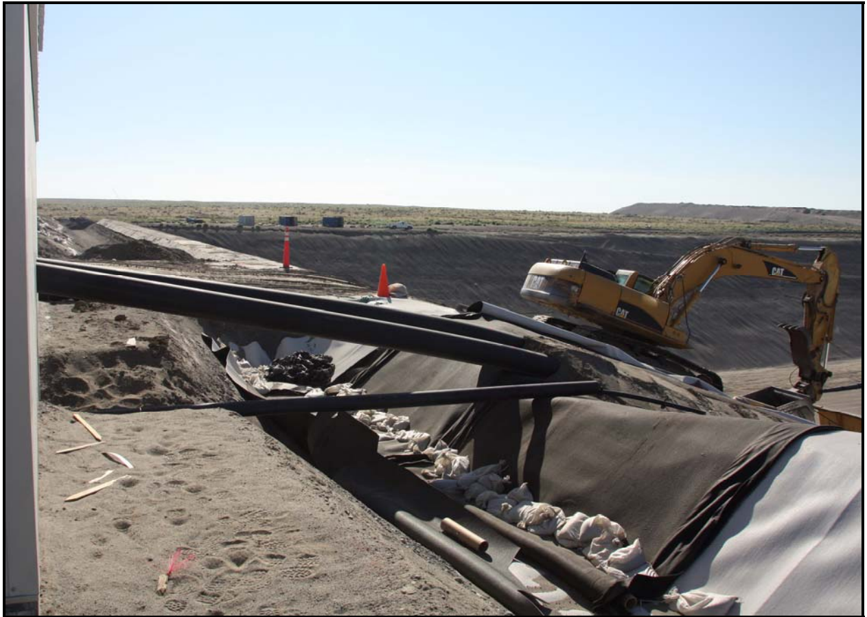
The secondary riser pipes from the sump to the crest pad building are installed in super cell 10 at the Environmental Restoration Disposal Facility.
