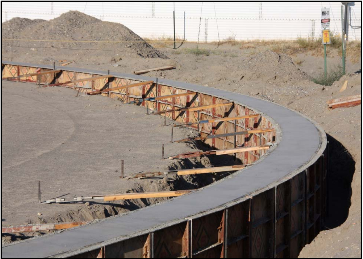
The concrete foundation was poured for the new leachate holding tank at the Environmental Restoration Disposal Facility.
