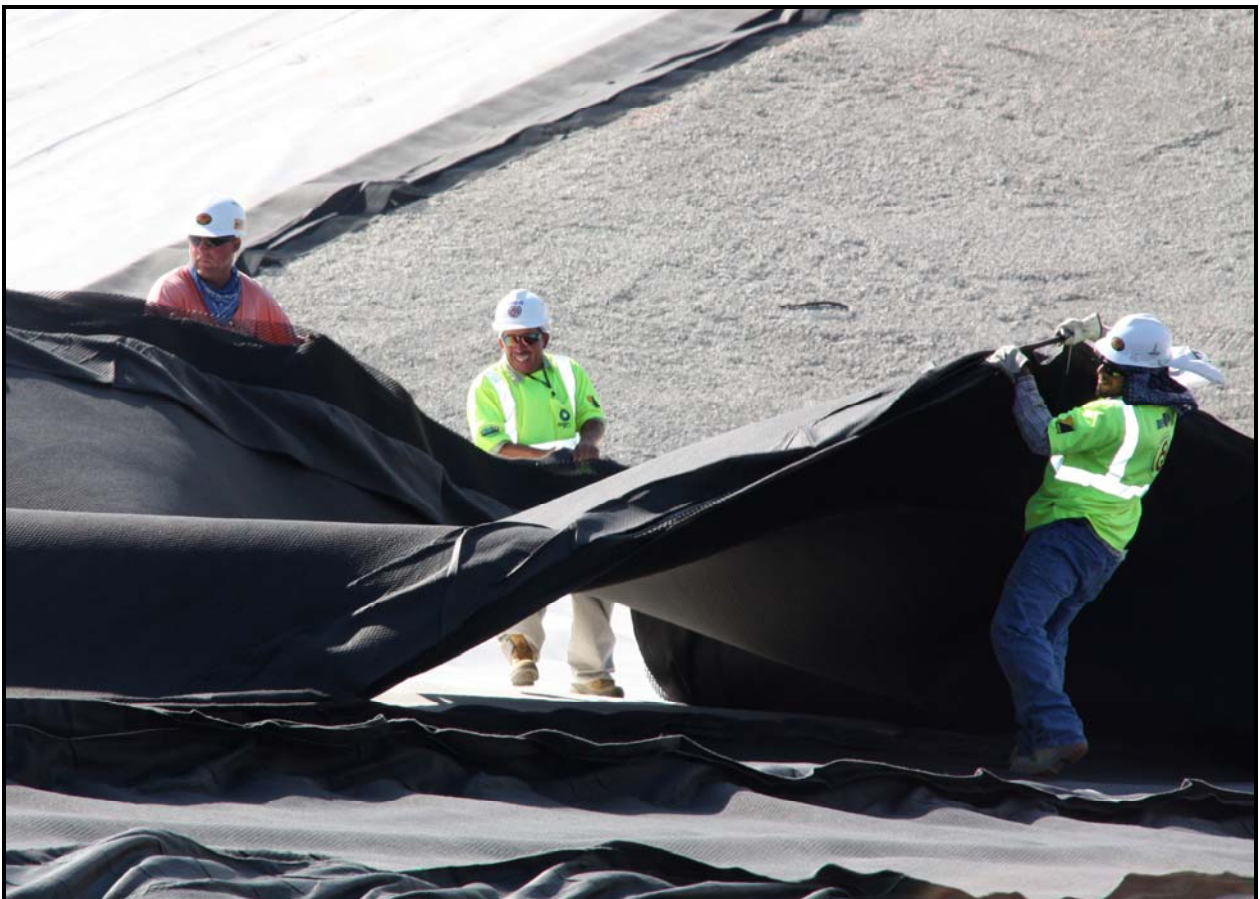
Workers install the geocomposite layer on the north slope of super cell 9 at the Environmental Restoration Disposal Facility.
