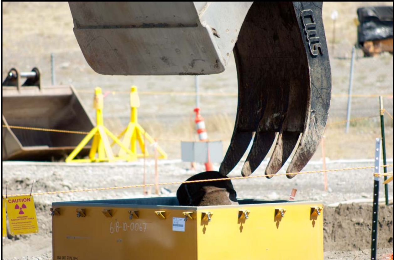
A track-hoe places the first unearthed drum into a steel container during intrusive characterization field operations at the 618-10 Burial Ground.
