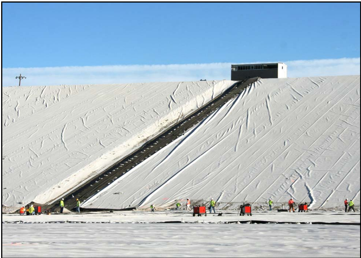
The project team completed the installation of the secondary high-density polyethylene layer in super cell 9 at the Environmental Restoration Disposal Facility.
