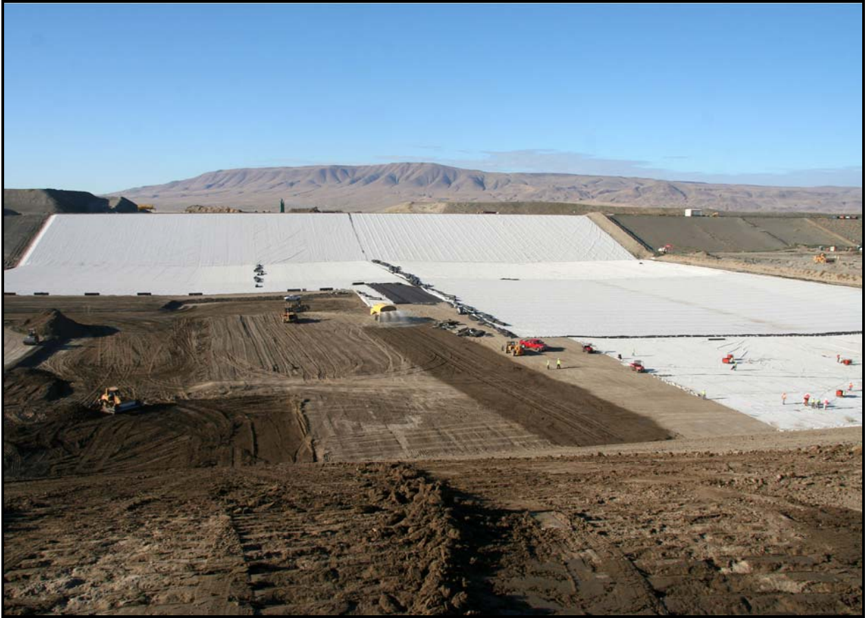
A view from the north end of super cell 10 shows the installation of the high-density polyethylene layers for super cells 9 and 10 and the placement of admix in super cell 10.
