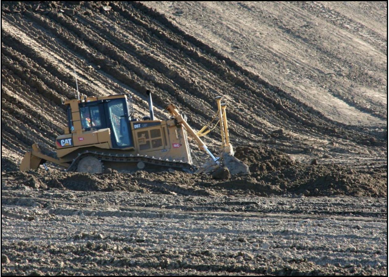
Work to form the sump area in super cell 10 is under way at the Environmental Restoration Disposal Facility.
