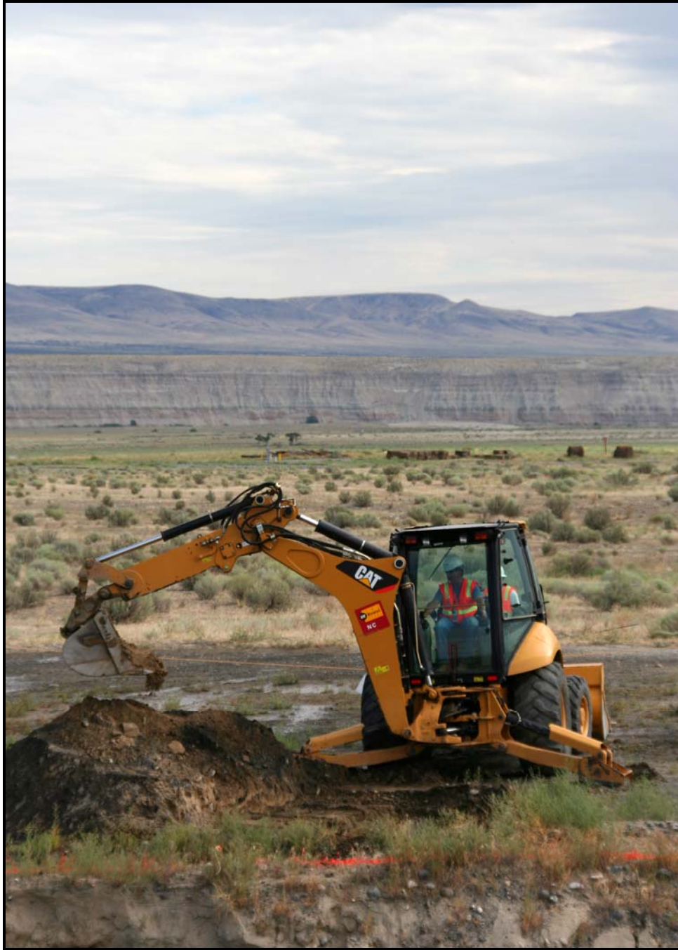
A TerranearPMC employee digs a test pit during Confirmatory Sampling activities at 100-D Area.
