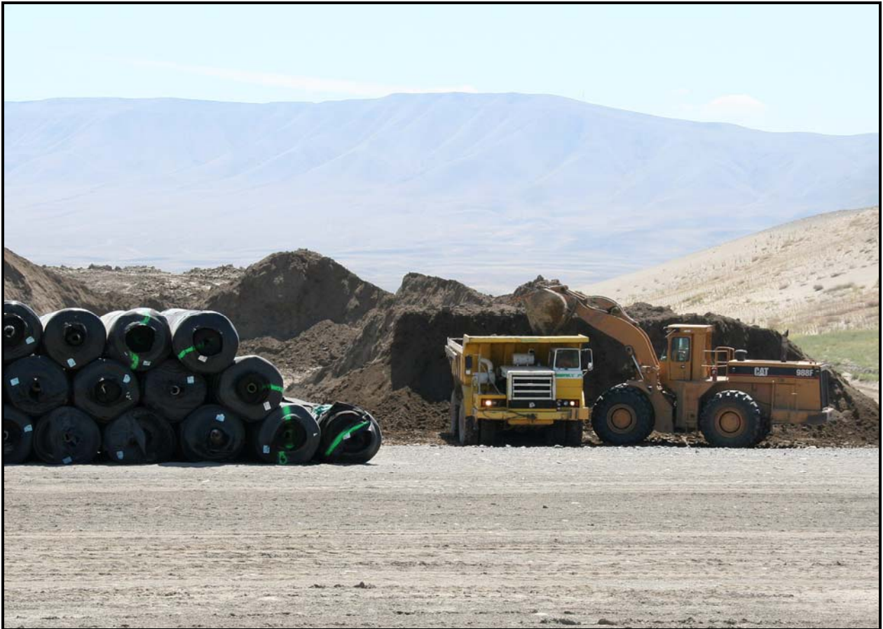
TradeWind Services/DelHur Industries personnel load admix manufactured at an onsite pugmill at the Environmental Restoration Disposal Facility. At left are rolls of high-density polyethylene.
