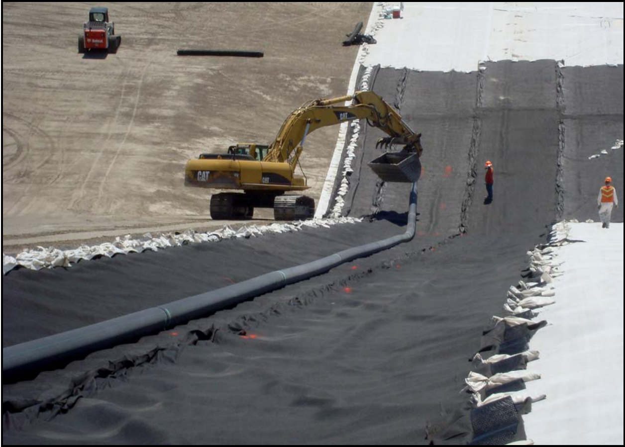
The secondary riser pipe is installed down the north slope of super cell 9 at the Environmental Restoration Disposal Facility.
