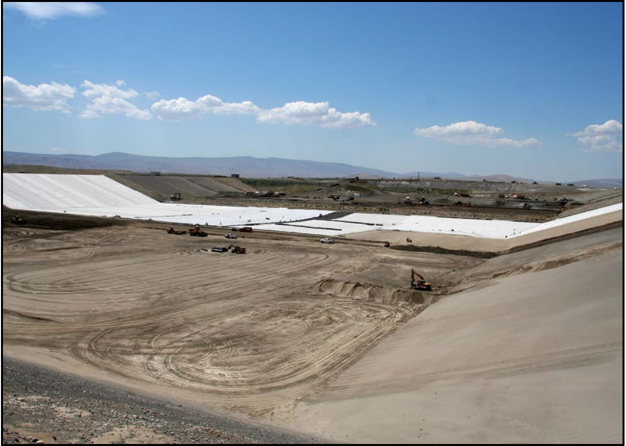
A view from the northeast corner of the Environmental Restoration Disposal Facility shows the high-density polyethylene liner being installed in super cell 9 and admix being placed in super cell 10.
