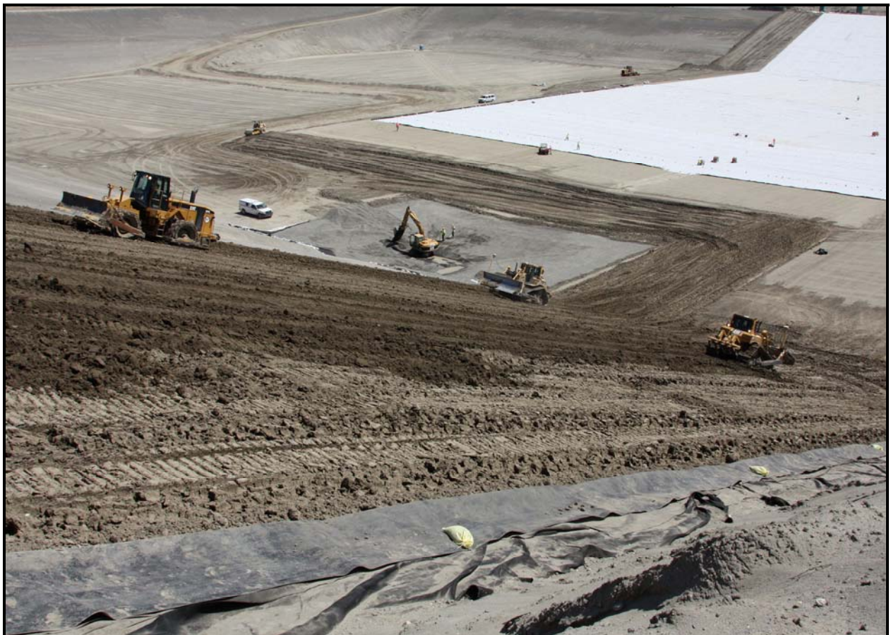
TradeWind Services/DelHur Industries personnel begin to place admix on the north slope of super cell 9 at the Environmental Restoration Disposal Facility.
