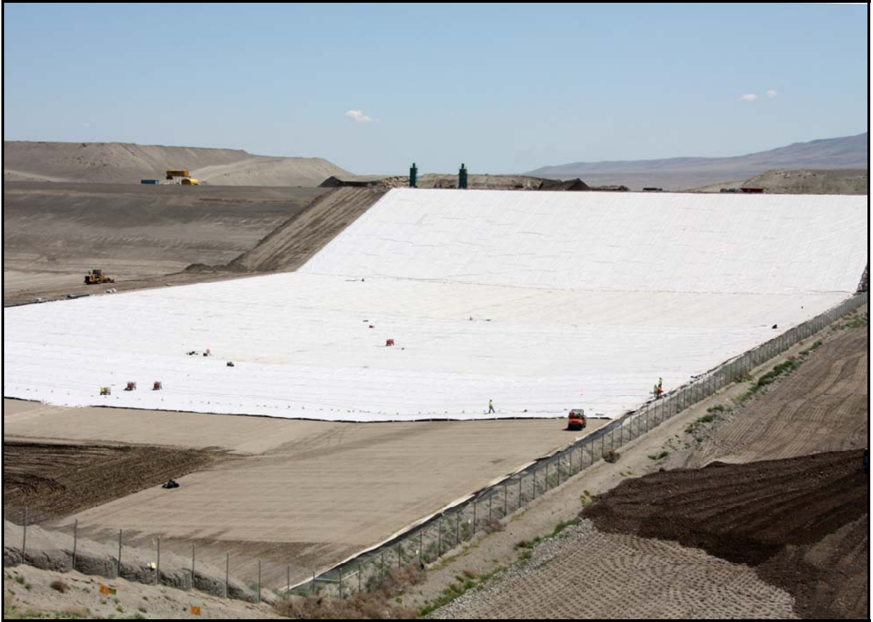
TradeWind Services/DelHur Industries personnel continue to install the secondary high-density polyethylene liner in super cell 9 at the Environmental Restoration Disposal Facility.
