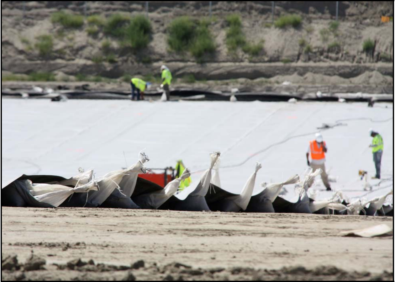
The 60-mil high-density polyethylene is rolled out in 540-by-22-foot sections and heat-welded together.
