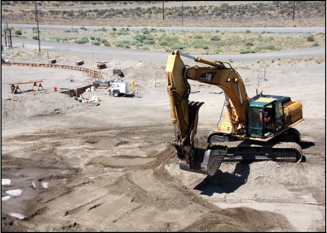
TradeWind Services/DelHur Industries personnel work on a new leachate holding tank near the main entrance to the Environmental Restoration Disposal Facility.
