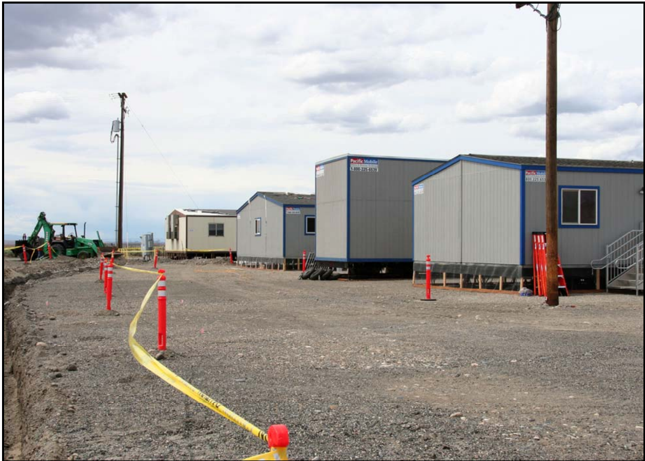
Three trailers are being installed and electrical work is being conducted at 100-F Area in preparation for Washington Closure Hanford to remediate 18 waste sites.
