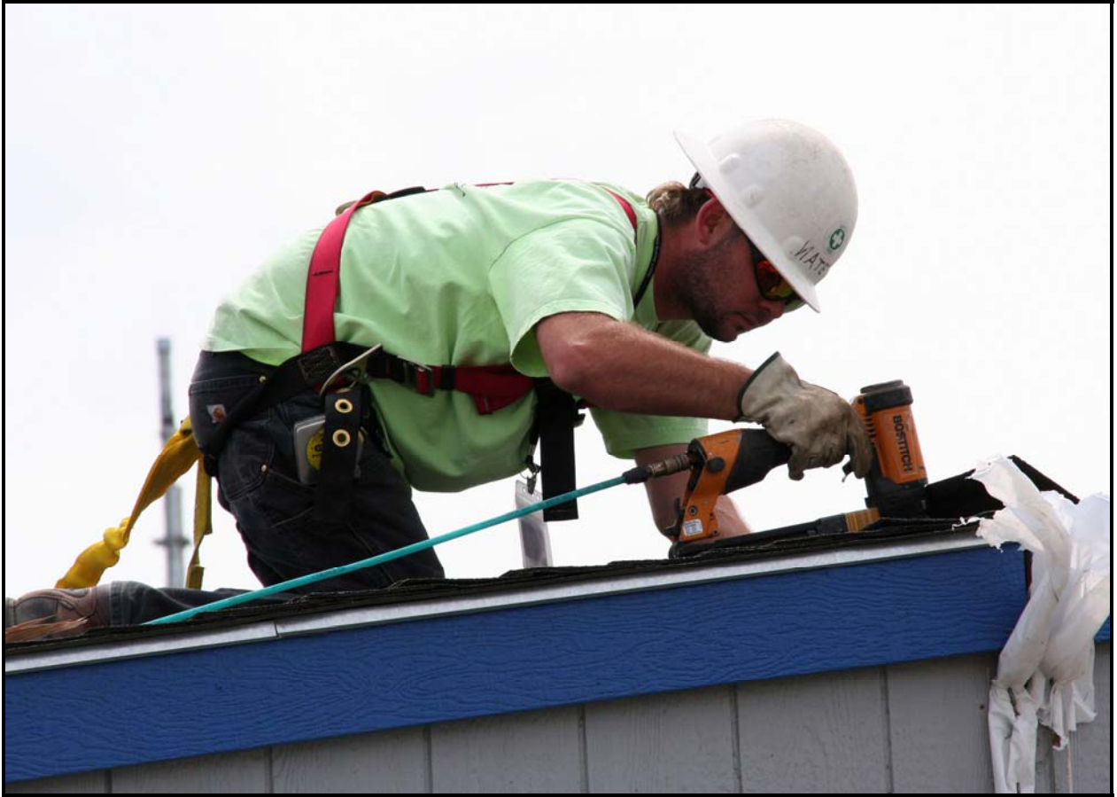
A Washington Closure Hanford subcontractor installs roofing tiles on a mobile trailer at 100-F Area.
