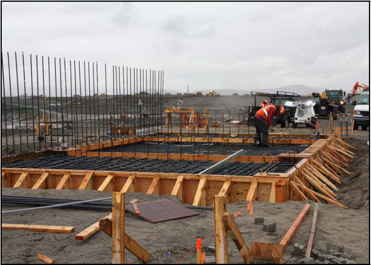
Work continues on the foundation of the crest pad building for super cell 9 at the Environmental Restoration Disposal Facility.
