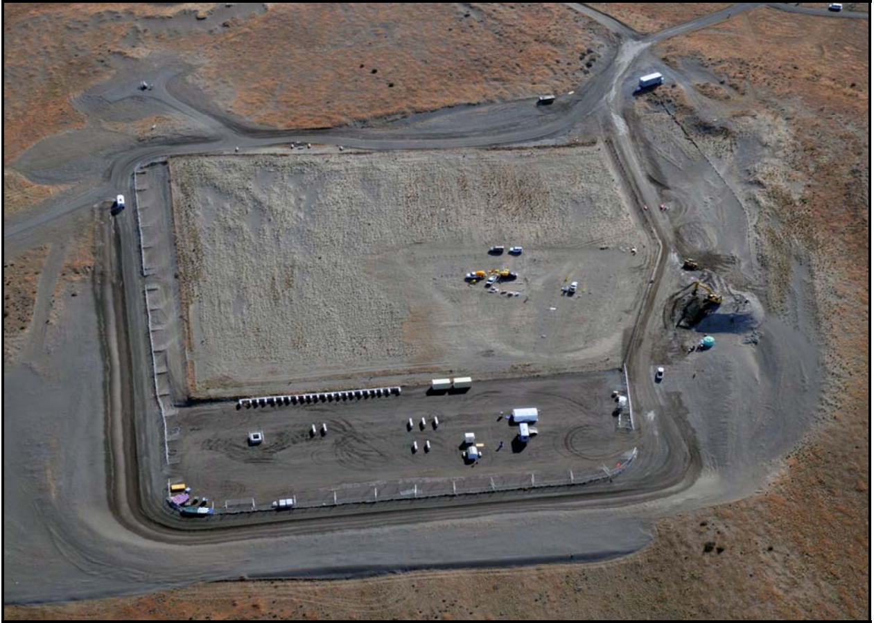
An aerial photo taken earlier this month from the west side of the 618-10 Burial Ground shows the nonintrusive characterization project team (center) characterizing vertical pipe units.
