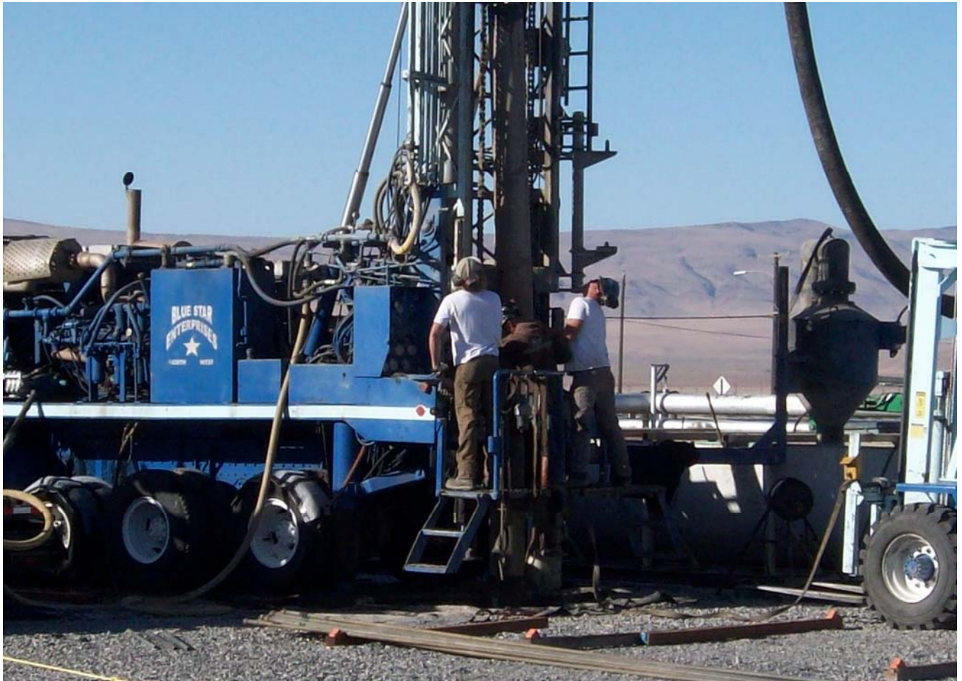
Workers from the subcontractor Blue Star add a casing to a well for the 200-ZP-1 system, for which two wells were recently drilled to total depth.
