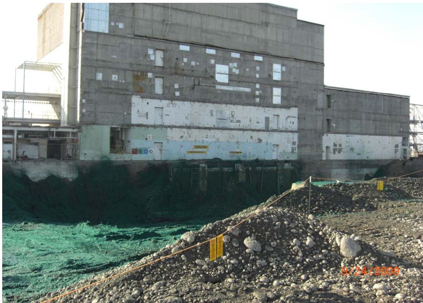
Application of this fixative is part of the effort on the 100K project to ensure positive contamination control to protect people, the environment and equipment during remedial action work beneath the basin.
