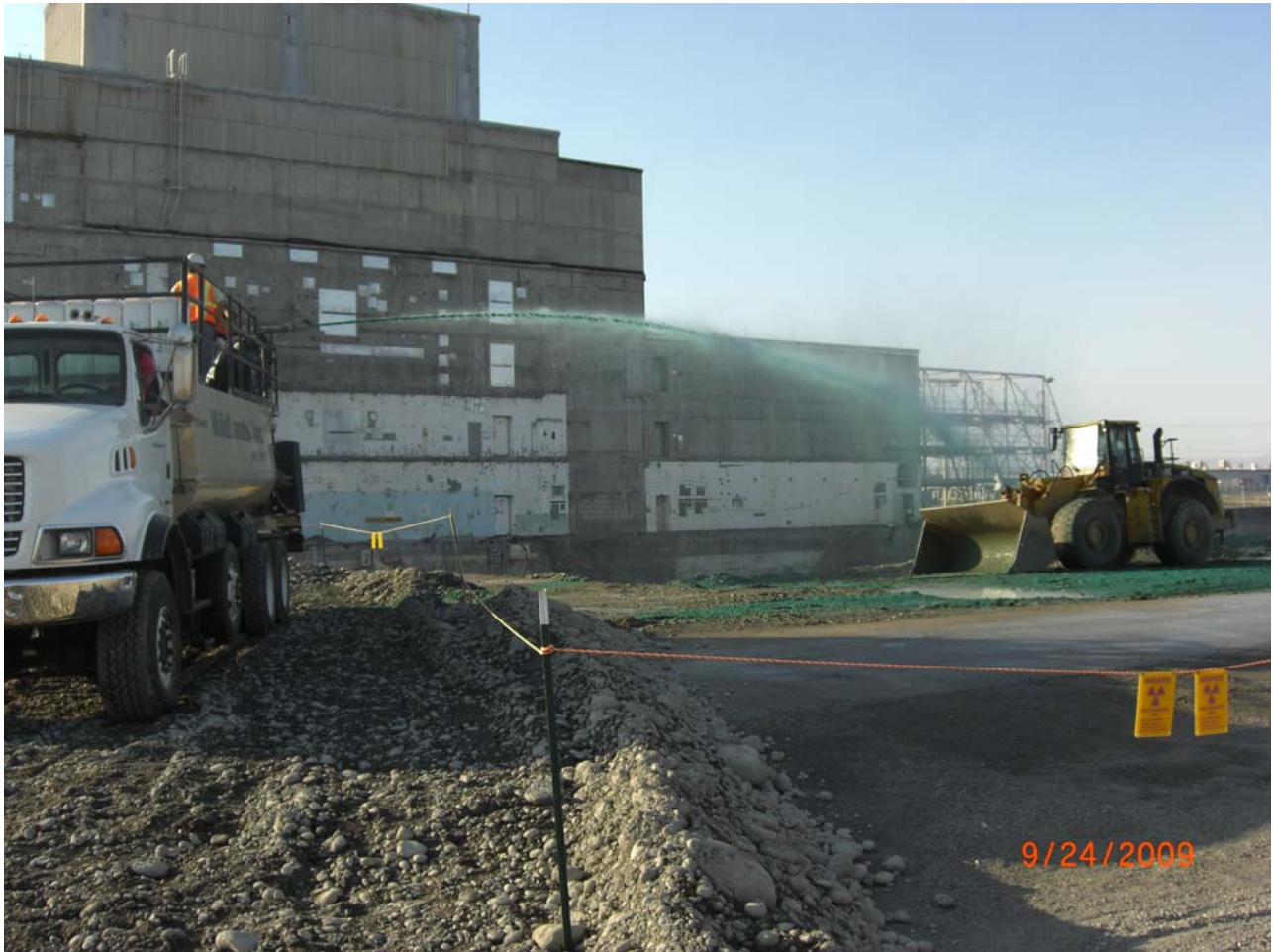
Workers apply fixative to the contaminated soil beneath the 105KE Fuel Storage Basin.
