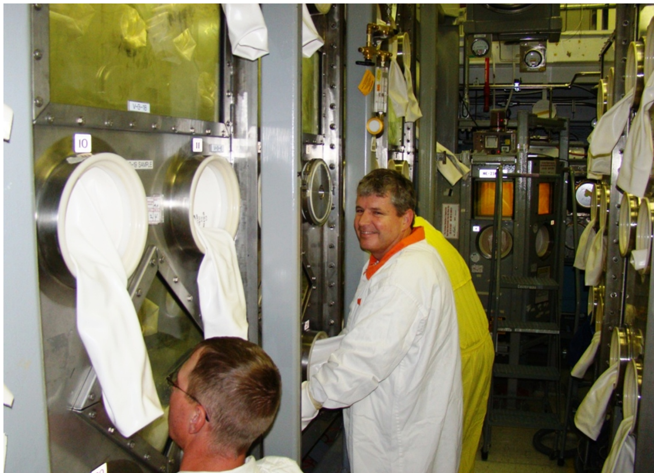
Workers prepare waste in the HC-230C-3 glove box for seal out. Internal supports had to be size reduced and removed because they could not be adequately accessed for cleaning.
