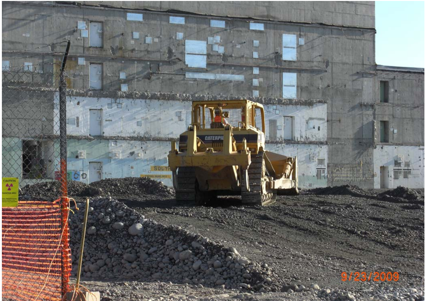
A bulldozer pushes clean fill into the UPR-100-K-1 waste site to create a clean pad that will support the basin remediation efforts.
