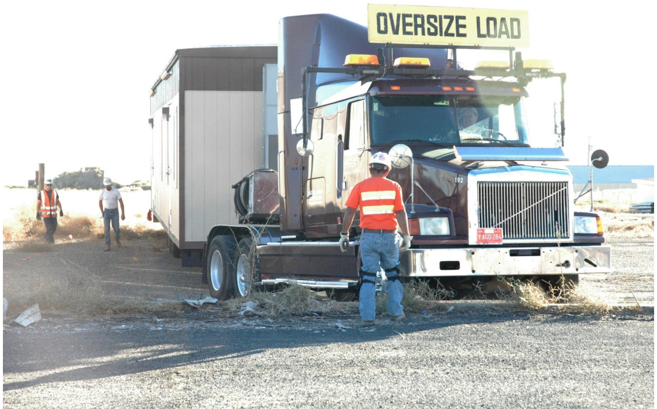
Workers coordinate the positioning of a trailer. While the trailers are being set up, preparations for demolition are already in progress, including controlled burning, weeding, and spraying or fogging for insects.
