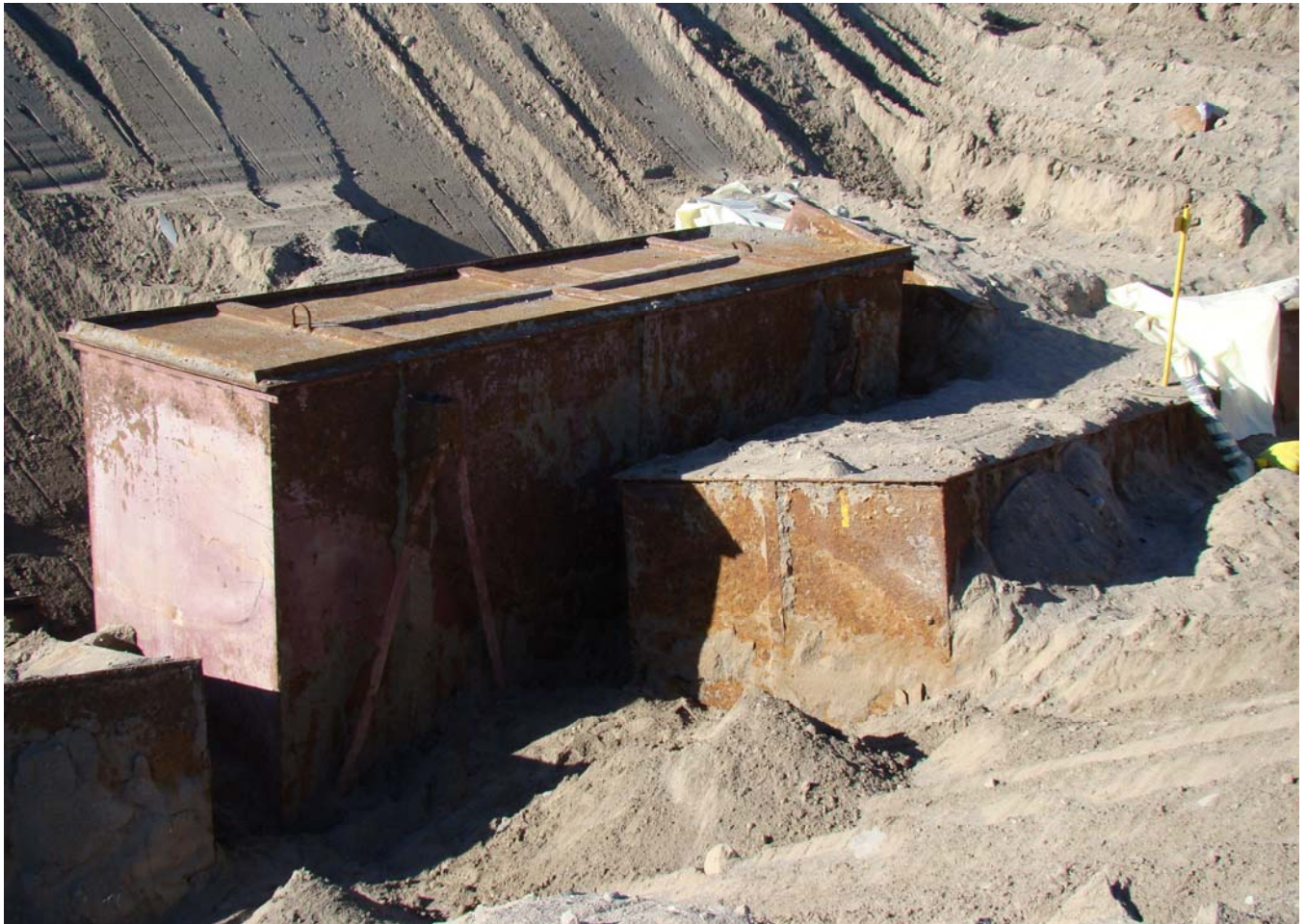
A metal waste container, to be removed from 218-W – 4B Trench 11, is engineered to handle the lathe (~25,000 pounds) that is inside. This non-standard waste container required the Engineering Group to evaluate its integrity to ensure it is sound for lifting and/or needs repairs. The Engineering Group will work with the Hoisting/Rigging Group to determine how to lift the box from the trench.
