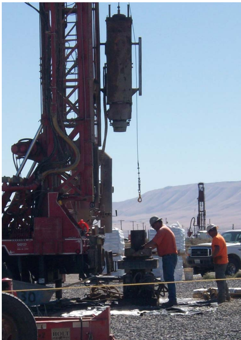
Workers from the subcontractor Water Development prepare to backpull a casing for construction of a well supporting the 200-ZP-1 groundwater treatment facility.
