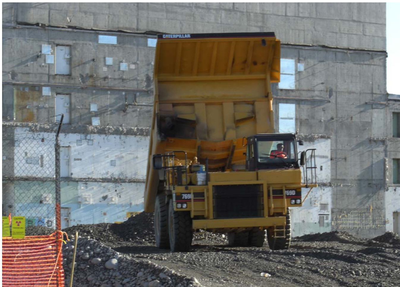
A rock truck dumps dirt that will be used to fill the UPR-100-K-1 waste site.
