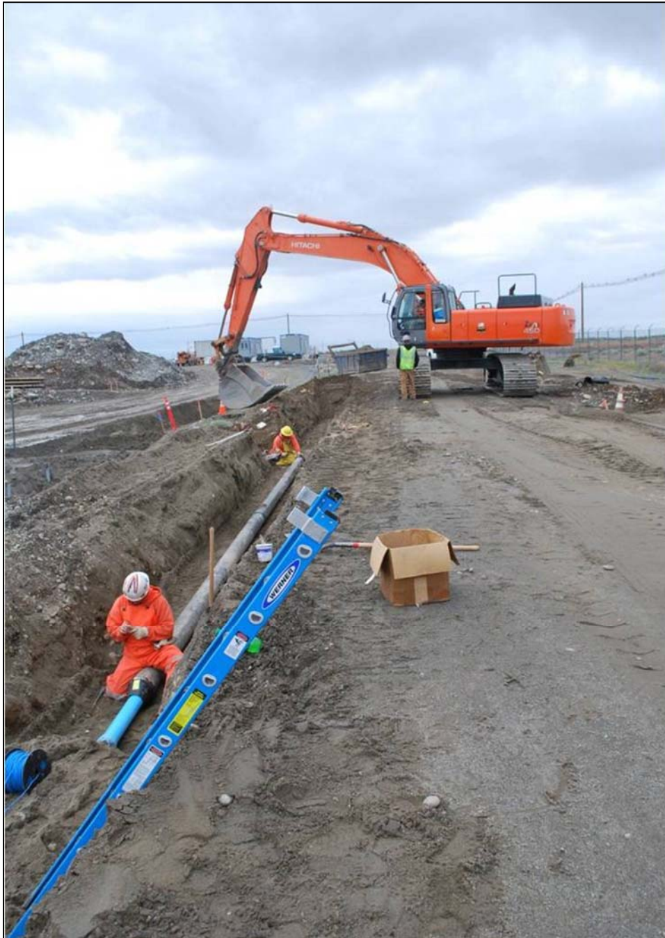
Workers install a section of the 4-inch potable water line in the 100K Area.
