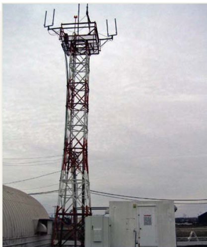
A 1-kW fuel cell system providing power for this FAA radio tower near Chicago
