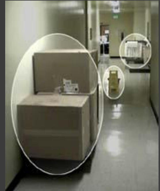
Obstructed exit route
