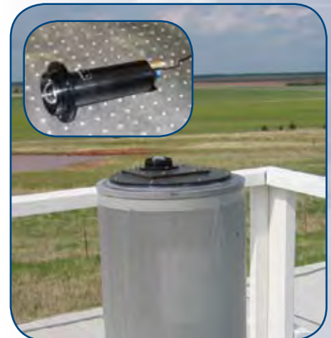
A ceiling port in the SGP Optical Trailer houses the optic element of the SWS, which connects to the spectrometer inside the trailer via fiber optic cable.
